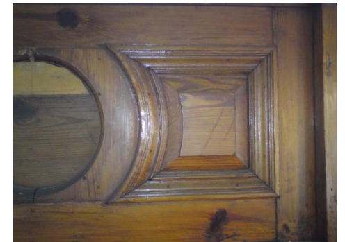
Gallery detail (missing clock)
