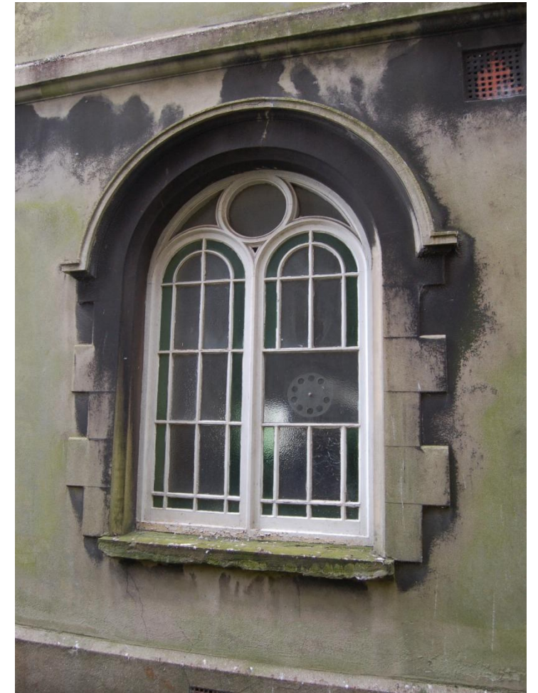
Original 'Florentine' windows with vent omitted within Worship Space (East) of School
