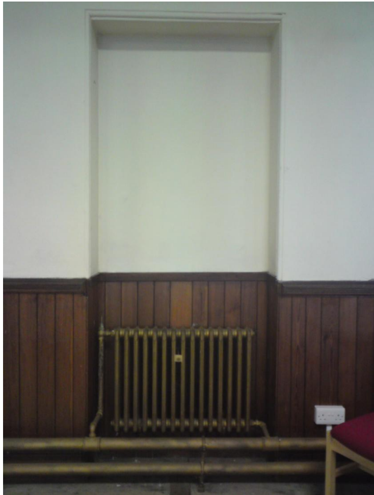
Original folding partition recess with newer cast iron radiator, Worship Space of School
