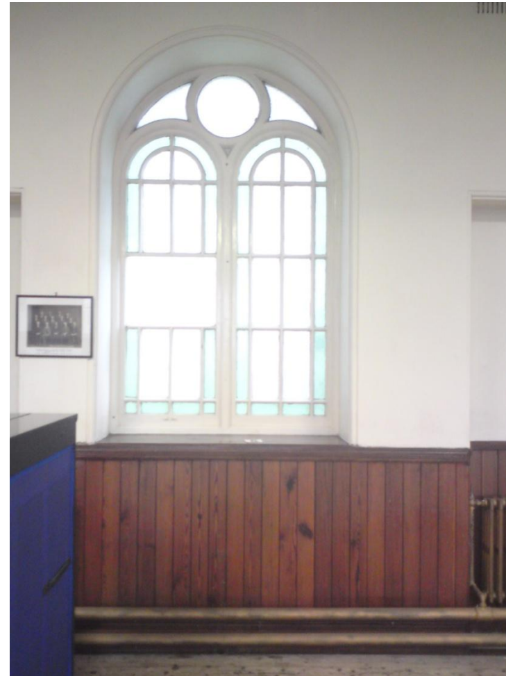
Original 'Florentine' windows with vent omitted within Worship Space (East) of School
