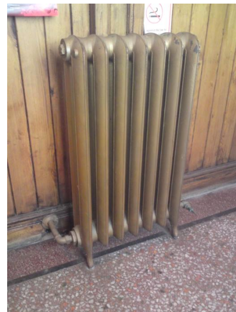
Cast iron radiator
