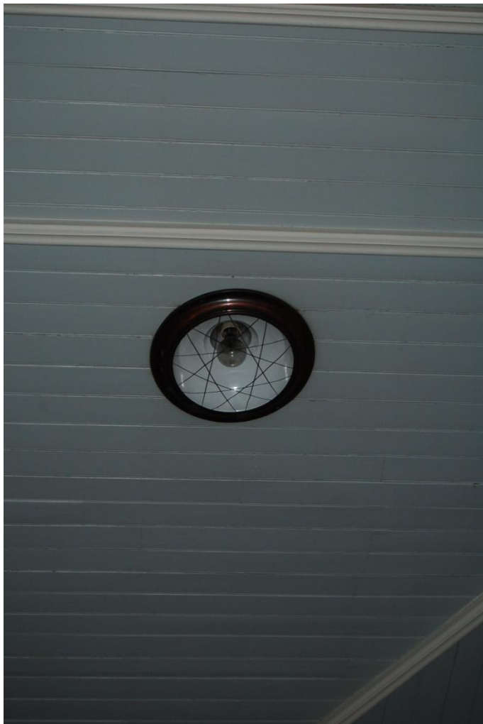
Ceiling level light fitting, Zion Chapel
