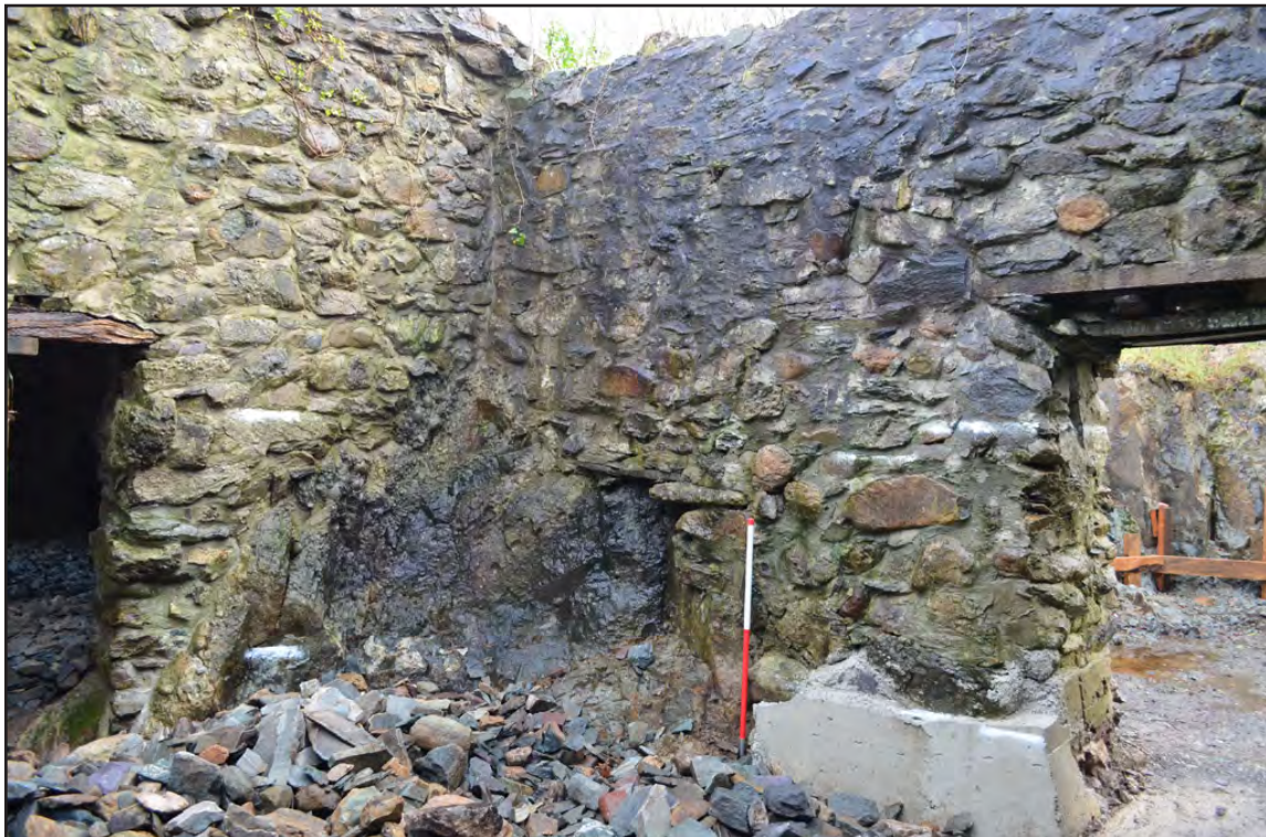
Plate 16: Southwest room - internal elevation: bedrock built into the east corner (Scale: 1 x 1.0m)
