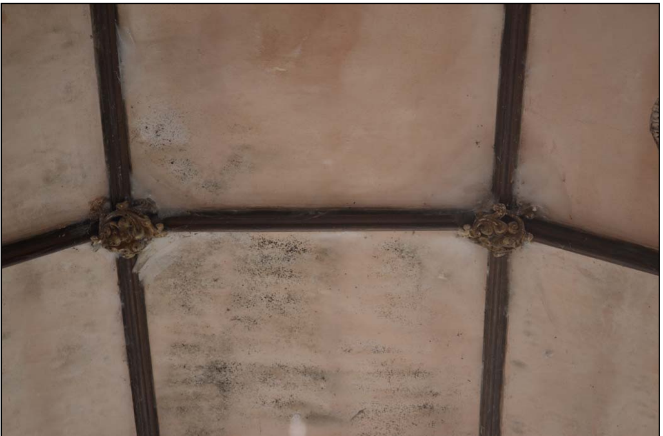
Plate 10: Capel Horeb ceiling showing bosses and ribs. Photograph taken from the northwest.
