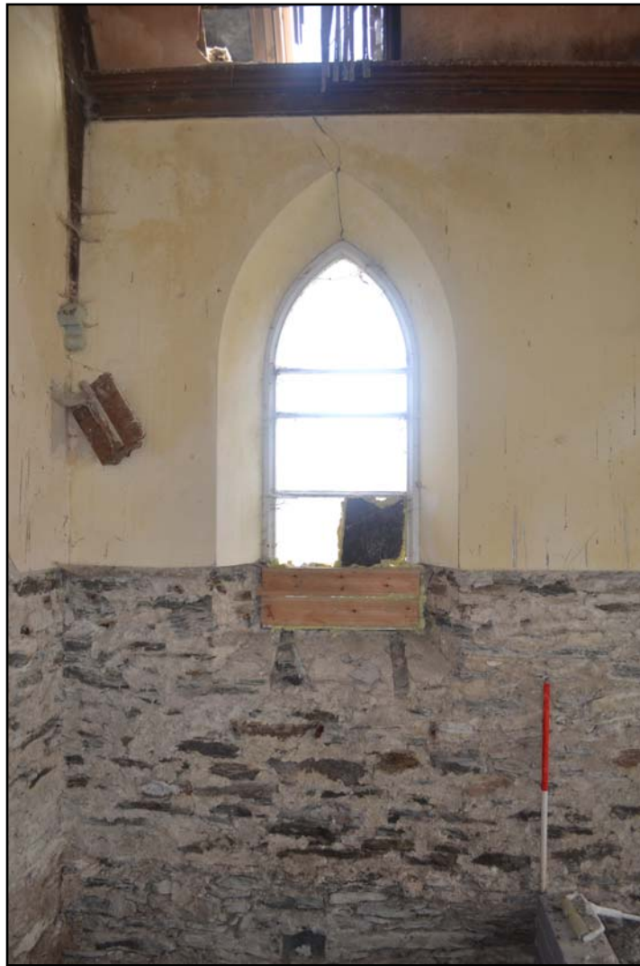
Plate 11: Capel Horeb internal northeast elevation showing lancet window. Photograph taken from the southwest.
