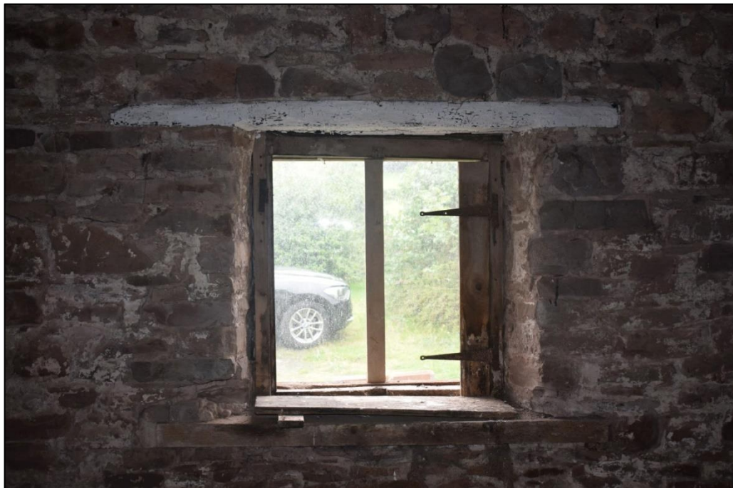
Fig. 8 Internal view of the mullion window in the south-east elevation Photo CPAT 4691-25
