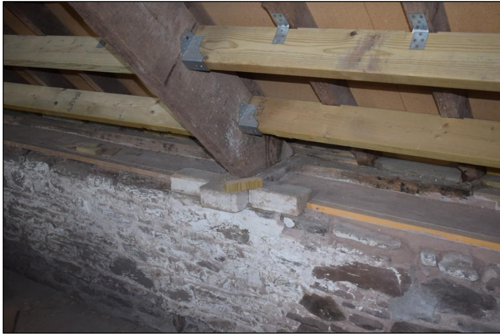
Fig. 15 Cruciform plinth to support the base of the rafter and boarding enclosing the eaves, viewed from the south Photo CPAT 4691-51
