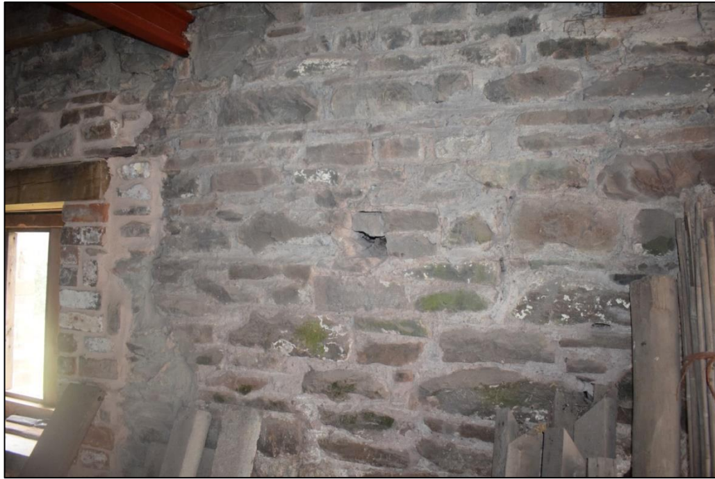
Fig. 11 One of a series of holes in the south-east elevation wall fabric Photo CPAT 4691-37
