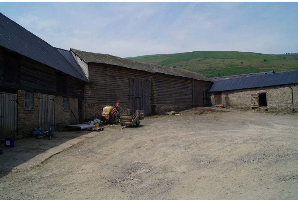
Plate 10: The view northwards to the western farmyard building range at Bache Farm.
