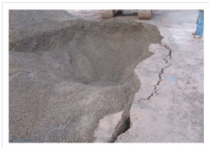
Plate 19: East tank position
