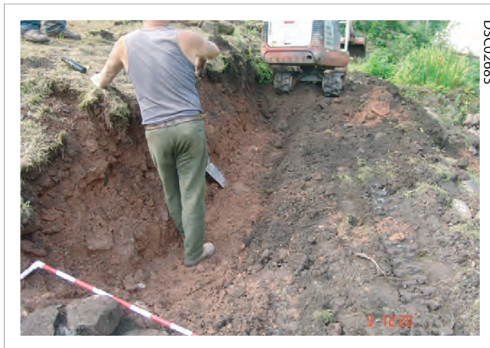
Plate 03: Removal of upper terrace garden wall revetment to provide a foundation for replacement wall.
