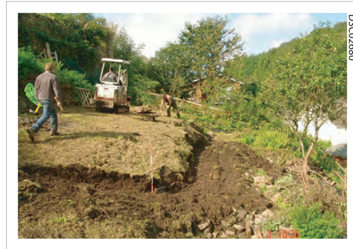
Plate 06: Overview of access path at upper terrace. Wall section at ranging rods
