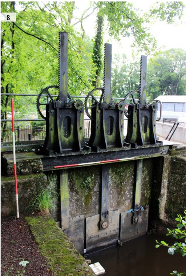
ILLUS 6 Corner of retaining wall on entrance to feeder channel (photograph taken prior to current development) ILLUS 7 Overflow channel (photograph taken prior to current development) ILLUS 8 Post-1875 sluice gates at western end of feeder channel (west elevation)
