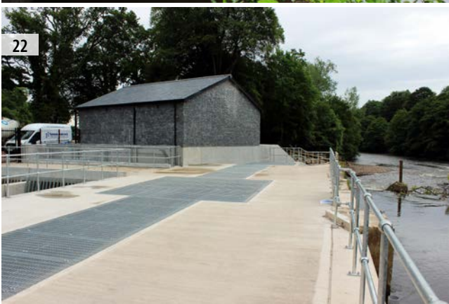
ILLUS 16 Section of backfilled overflow channel (following completion of site works) ILLUS 17 Excavation of hydroelectric plant footprint (photo courtesy of Dawnus Construction) ILLUS 18 Demolition of 20th century fish pass structure (photo courtesy of Dawnus Construction) ILLUS 19 Demolition of section of retaining wall to create feeder channel for Hydroelectric plant (photo courtesy of Dawnus Construction) ILLUS 20 Corner of retaining wall on entrance to feeder channel (following development) ILLUS 21 Eastern end of weir (following development) ILLUS 22 Hydroelectric plant and fish pass following development
