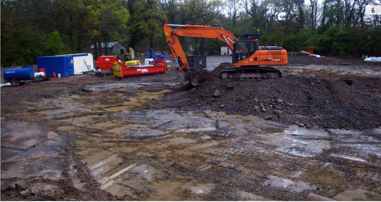
ILLUS 3 Working shot of machine stripping, facing NE ILLUS 4 Machine stripping in progress ILLUS 5 Modern path, facing E ILLUS 6 Stripped area showing modern path
