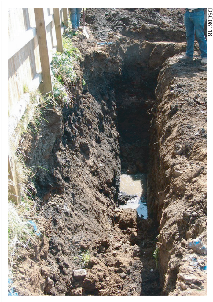
Plate 11: Trench 3, eastern face showing second collapse undermining boundary fence
