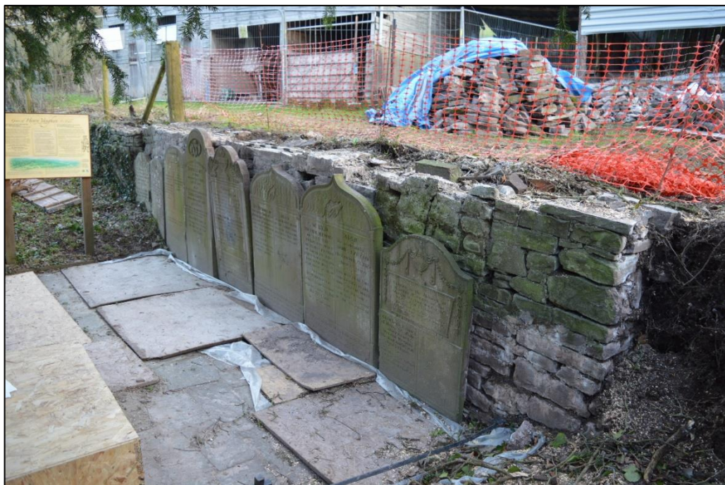
Fig. 7 West elevation of building forming part of the churchyard boundary. Photo CPAT 4586-0002
