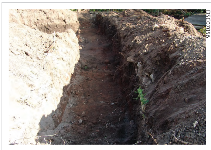
Plate 01: Overview of trench 1 at end of excavation with mechanical digger, sides collapsing
