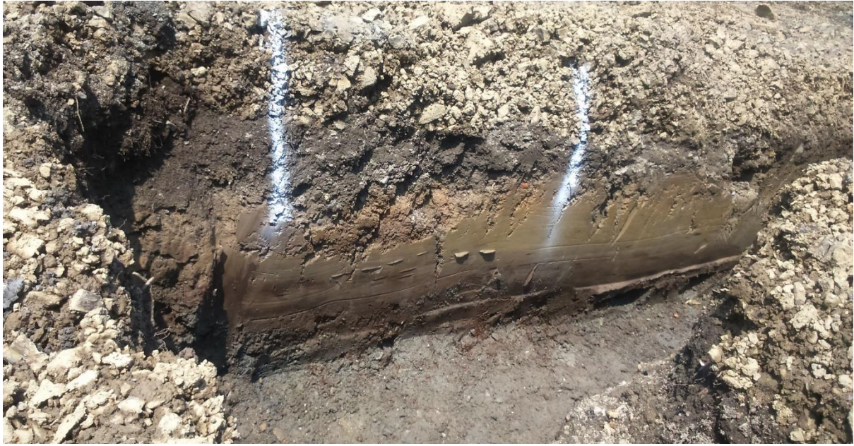
Plate 8: Foundation of rear side (southeast) Trench 9, corner with Trench 8 (northeast side), facing southeast
