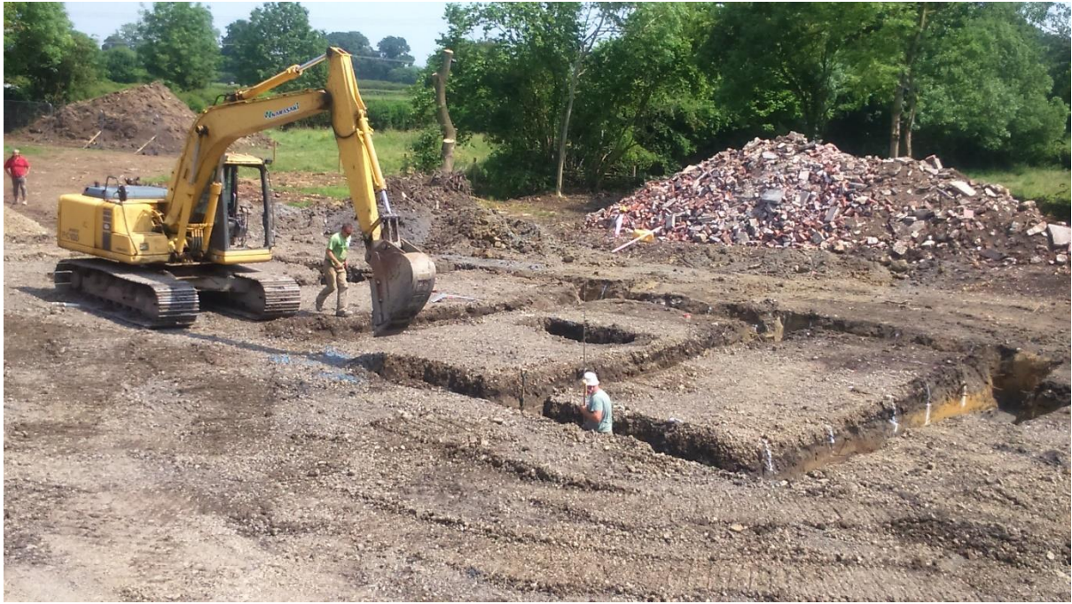
Plate 10: Rhos Common, Llanymynech, layout after excavation of new dwelling foundations, facing east
