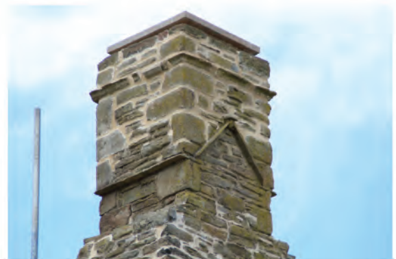
Plate 43: View of feature (28) within fabric of west chimney (27) of Abbot's House in west wing.
