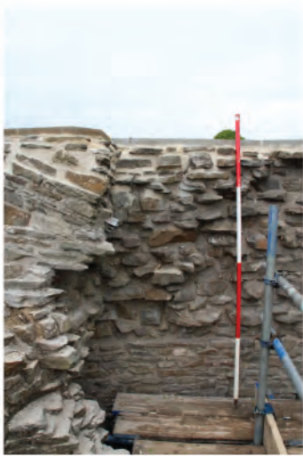
Plate 202. Interior view of spring of arch in Abbot's Stairwell at upper level. Looking west.
