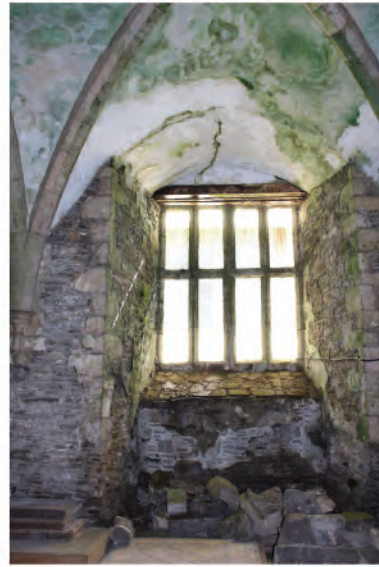
Plate 261. West window of South wall in undercroft prior to lintel replacement. Looking south
