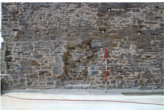
Plate 76: Remains of blocked in former 13th century dormitory window (200) in west wall internal side. Looking west following scaffold removal.
