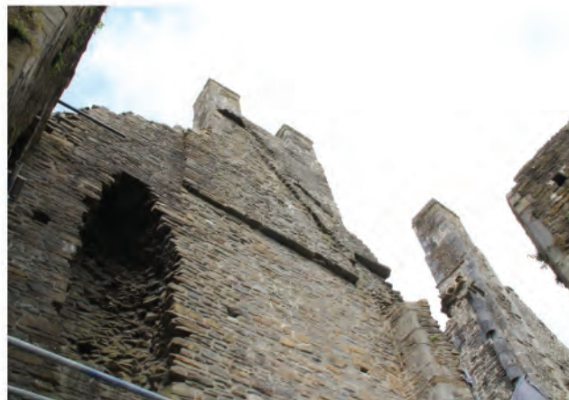
Plate 109. View of southern end of east facing external elevation of east wall, showing projecting back of chimney and vice passage opening (81). Looking northwest.
