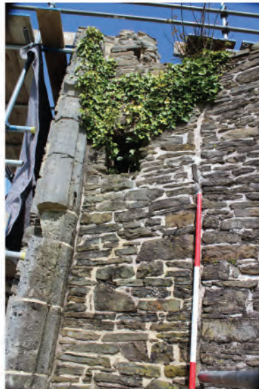
Plate 198. View of hidden window in core of east wall abutting Abbot's Stairwell. Looking north.
