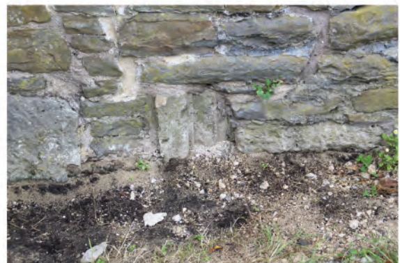
Plate 88. Detail shot showing remains of moulded door jambs (66) in south wall below east window in south wall. Looking north.
