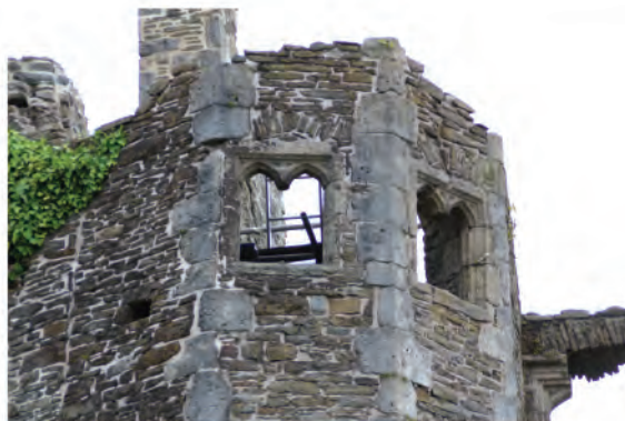
Plate 195. View of Abbot's Stairwell showing 15th - 16th century window pair in south elevations. Looking northwards.
