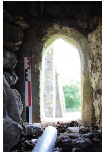
Plate 213. Interior view of small loop window in east facing elevation of Abbot's Stairwell. Looking east.
