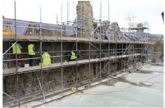
Plate 61: Working shot of east facing elevation of west wall during consolidation work. Looking northwest.
