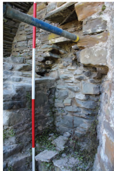
Plate 19: Detail of blocked opening (19) below relieving arch of Day Stair. Looking eastwards.
