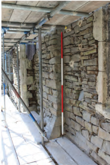
Plate 97: View of buttress (101) at first floor level in east facing elevation of east wall. Looking southwest.
