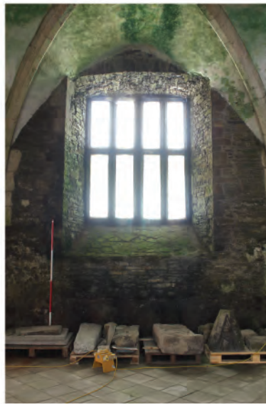
Plate 179. View of inserted late Tudor window in undercroft east wall. Looking west.
