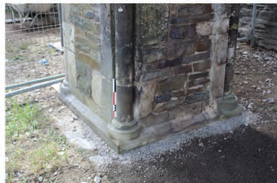
Plate 168. Detail of bottom mouldings of central bridge support pier on south side of bridge. Looking southwest.
