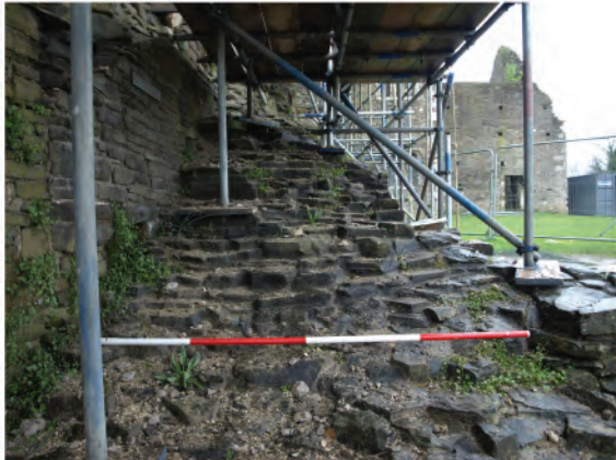
Plate 14: View of remains of Monk's Day Stairs at north end of West wall. Looking south.
