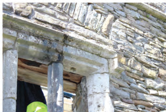
Plate 104. View of hood moulding of late Tudor window in east facing elevation of east wall (120). Looking westwards.
