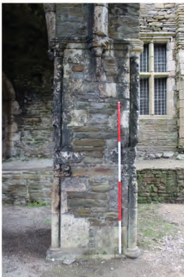
Plate 167. View of central bridge support pier on north side of bridge. Looking west.
