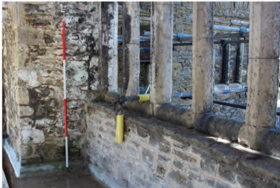
Plate 68: View of square headed late Tudor window (8) in west wall. Looking south-west.
