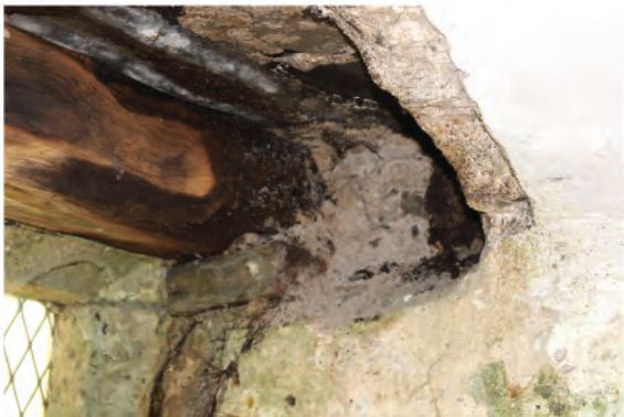
Plate 267. Timber lintel removed in east window. Looking southwest into beam slot.
