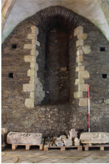
Plate 182. Blocked 13th century lancet window in west wall in undercroft. Looking west.
