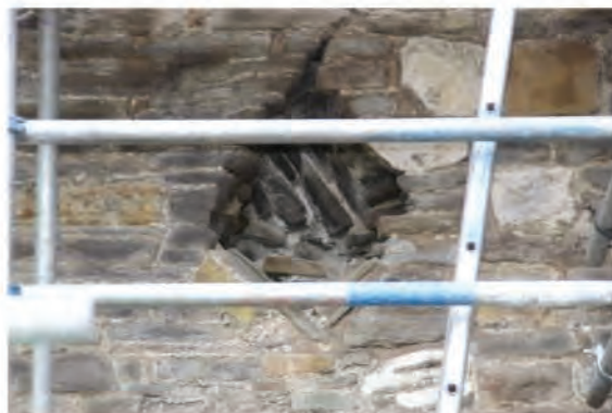
Plate 135. Small niche or recess in east wall at far southern end (85). Looking west.
