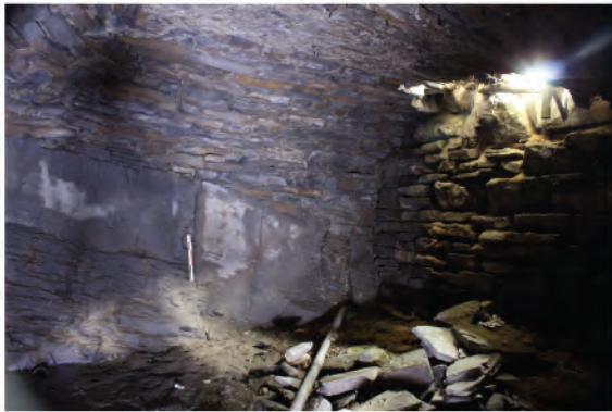
Plate 188. View of south facing wall of cell / vault beneath Slype passage. Looking north.
