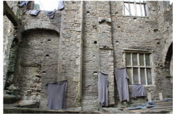
Plate 12: View central part of east facing elevation of undercroft following removal of scaffolding. Looking west.
