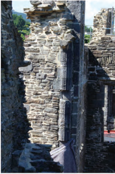
Plate 147. Detail shot of side jambs in tall late 15th - early 16th century window in east wall (92). Looking north.
