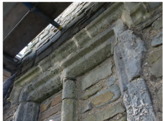
Plate 162. Detail shot of jambs and mullion in false window in south facing elevation of south wall of bridge (160). Looking northwest.
