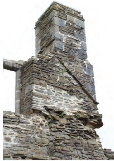
Plate 149. View of chimney (98) and former roof lines (180) in west facing elevation of east wall. Looking east.
