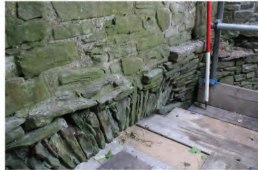
Plate 203. Interior view of top of doorway arch in Abbot's Stairwell at upper level. Looking east.
