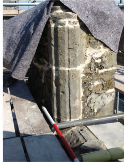
Plate 39: Detail of side jamb in top attic window (3) in west wall. Looking northwards.
