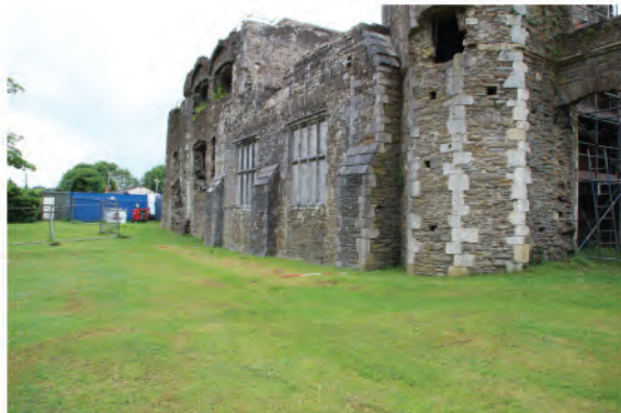
Plate 218. Oblique view of south wall and area of proposed drainage trench. Looking westwards.
