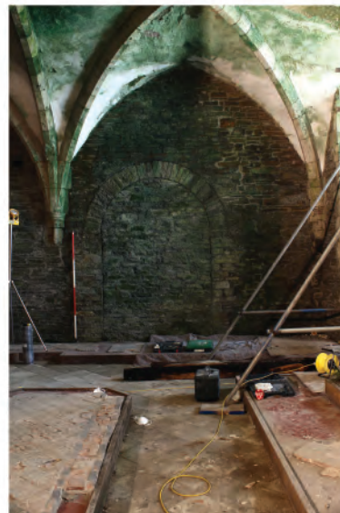
Plate 181. View of blocked round arched doorway at south end of undercroft in east wall. Looking west.
