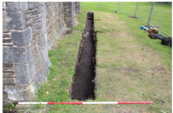
Plate 229. View of drainage trench following removal of redeposited material to required depth. Looking eastwards.
