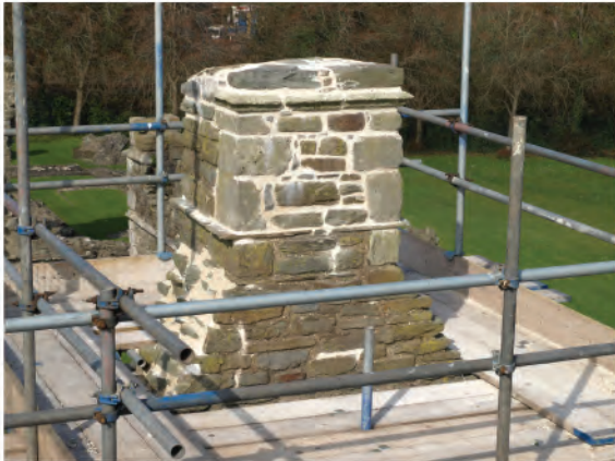
Plate 95: View of top of chimney stack in south wall of bridge. Looking northwards.
