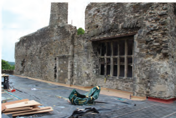
Plate 64: View of east facing elevation of west wall following scaffold removal. Looking southwest.
