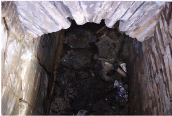
Plate 186. Entrance into cell or vault in floor of north unit of Novice Room. Looking north.
