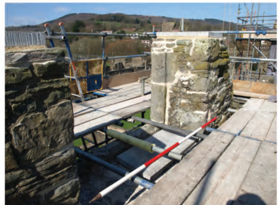
Plate 37: View of remains of top attic window in west wall (3). Looking northwest.
