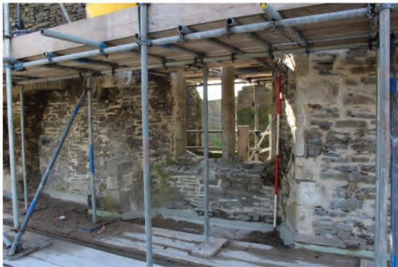
Plate 158. View of west window of north facing internal elevation of south wall of bridge. Looking southeast.
