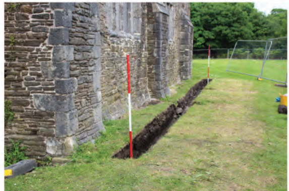
Plate 227. View of drainage trench following removal of redeposited material to required depth. Looking eastwards.
