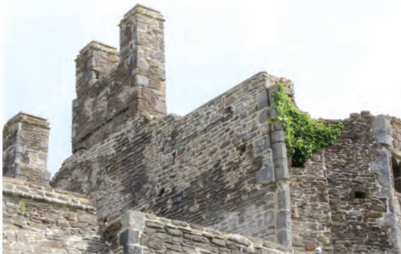
Plate 145. Detail shot showing chimney pair at southern end of east wall. Looking northwest.
