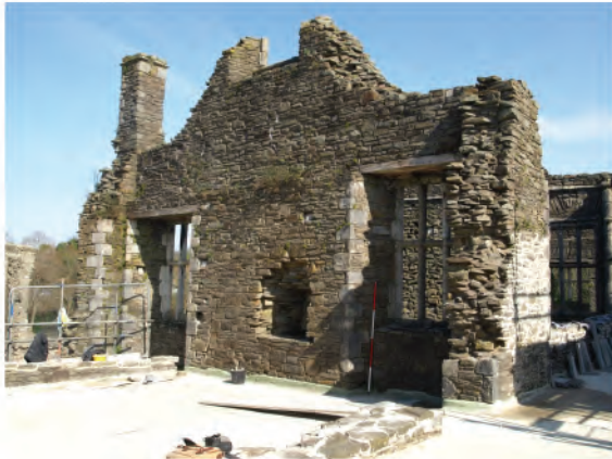
Plate 136. View of northern end of west facing internal elevation of east wall. Looking northeast.
