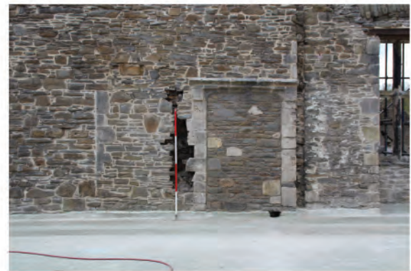
Plate 75: Remains of blocked 15th century doorway (33) in west wall from internal side. Looking west following removal of scaffolding.
