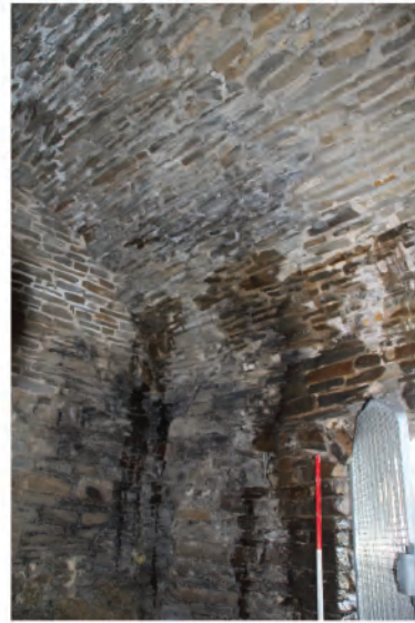
Plate 236. North-western corner of Novice Room where bore-hole was proposed through barrel vaulted ceiling. Looking northwest.
