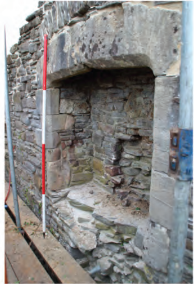
Plate 51: View of remains of 15th century fireplace in west wall at second floor level (30). Looking northwards.
