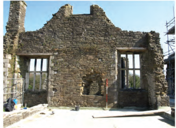
Plate 137. View of northern end of west facing internal elevation of east wall. Looking east.
