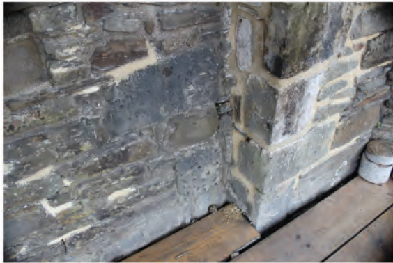
Plate 20: Detail showing line of vertical ashlar quoins (11) on north side of oriel window in west wall. Looking southeast.
