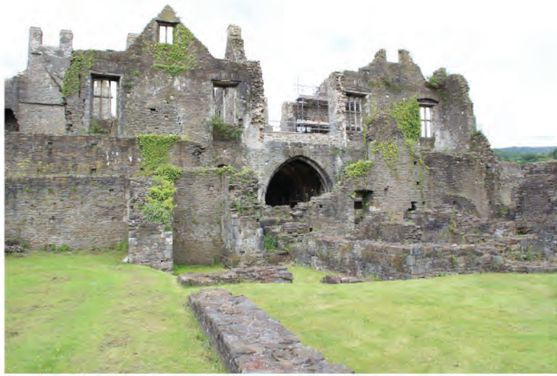
Plate 3. View of eastern wing of Tudor Mansion during consolidation work. Looking northwest.
