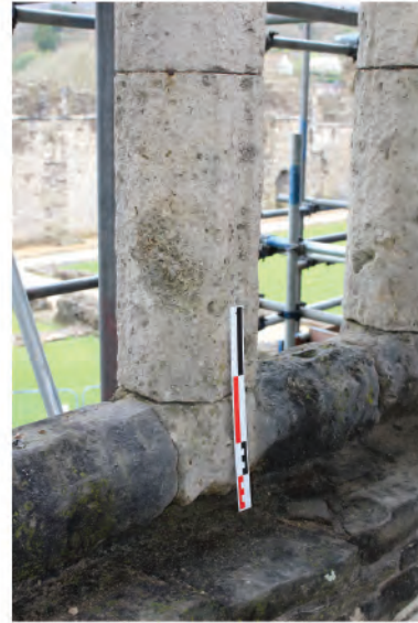
Plate 67: Detail shot of base jamb and mullion in window in west wall (8). Looking northeast.
