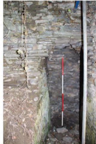
Plate 209. Interior view showing blocked doorway at ground level into undercroft in Abbot's Stairwell. Looking west.
