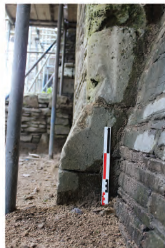
Plate 120. Detail of corner moulding at base of chimney showing pyramidal stop. Looking south.
