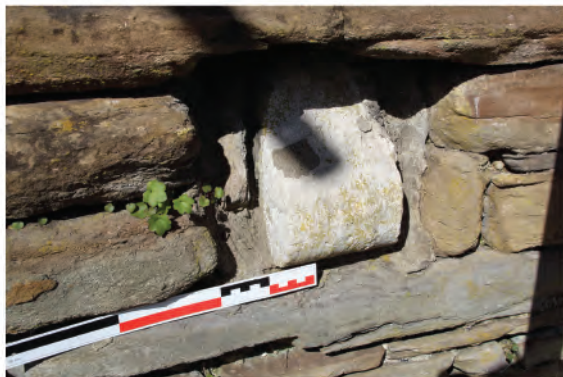
Plate 124. Detail shot showing re-used moulded Sutton stone used to block put-log hole in east wall (128). Looking northwest.
