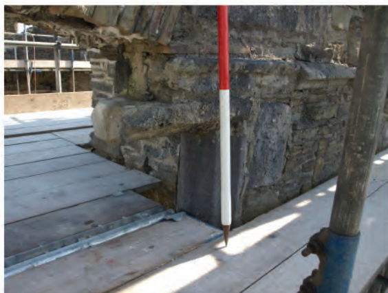
Plate 24: Remains of top and base jamb of oriel window (6) in west wall. Looking southeast.
