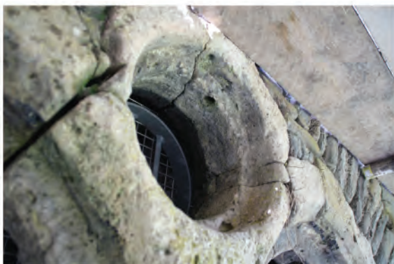
Plate 93. Detail shot of oculus window above doorway into Novice Room (136) in east wall. Looking northwest.
