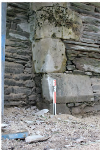
Plate 119. Detail of corner moulding at base of chimney showing pyramidal stop. Looking northwest.
