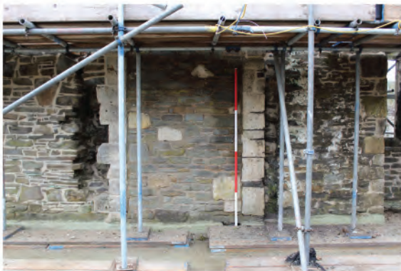
Plate 74: Remains of blocked 15th century doorway (33) in west wall from internal side. Looking west.
