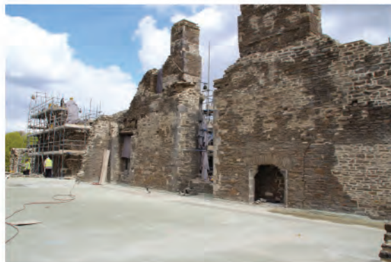
Plate 152. General view of west facing internal elevation of east wall. Looking northeast following removal of scaffolding.
