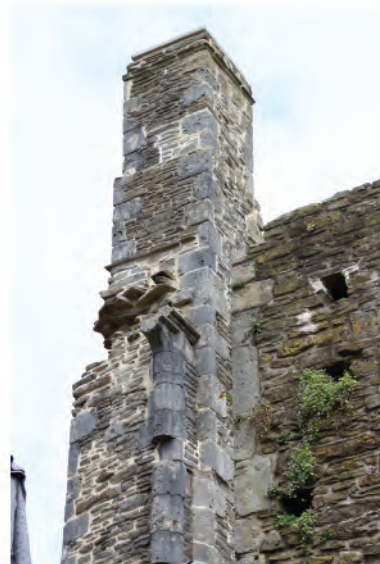
Plate 146. Detail shot of remains of side jambs and hood moulding of tall late 15th - early 16th century window in east wall (92). Looking northwest.
