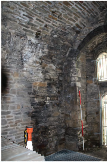
Plate 235. North-eastern corner of Novice Room where bore-hole was proposed through barrel vaulted ceiling. Looking northeast.
