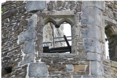
Plate 208. View of double arch window at upper level in Abbott's Stairwell. Looking north.
