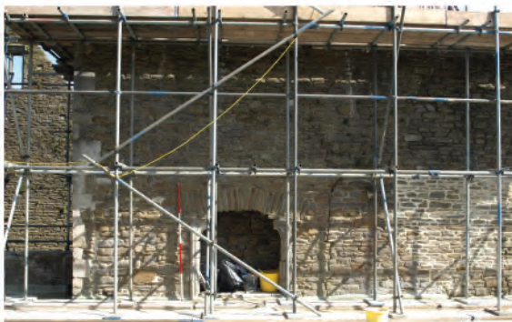
Plate 139. Southern end of west facing internal elevation of east wall showing 15th - 16th century fireplace (186). Looking east.
