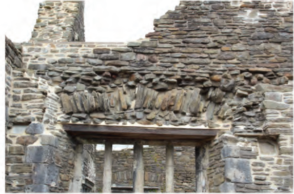
Plate 142. View of exposed relieving arch above square headed Tudor window in east wall (107). Looking east.
