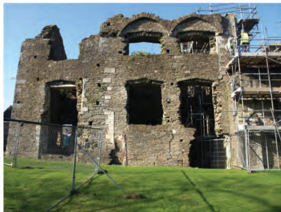
Plate 6: View of south facing elevation of Tudor Mansion (Abbot's House - West wing and former Refectory) during consolidation work. Looking north.
