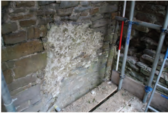
Plate 56: View showing curved area of walling at first floor level in west wall (37). Former stair arrangement. Looking southeast.
