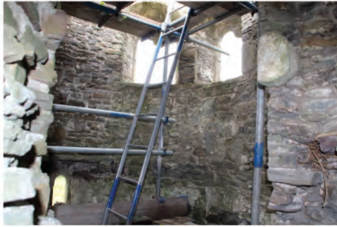
Plate 206. Interior view of double arch window at upper level of Abbot's Stairwell. Looking southeast.
