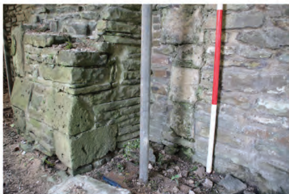
Plate 42: Detail showing base of buttress (44) in west wall at southern end and vertical line of ashlar quoins (45). Looking northeast.
