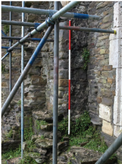
Plate 40: Remains of buttress in west wall (33). Looking northeast.
