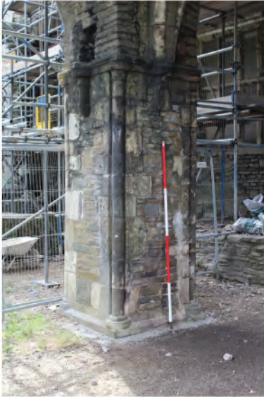
Plate 163. View of central bridge support pier at south side of bridge. Looking southwest.
