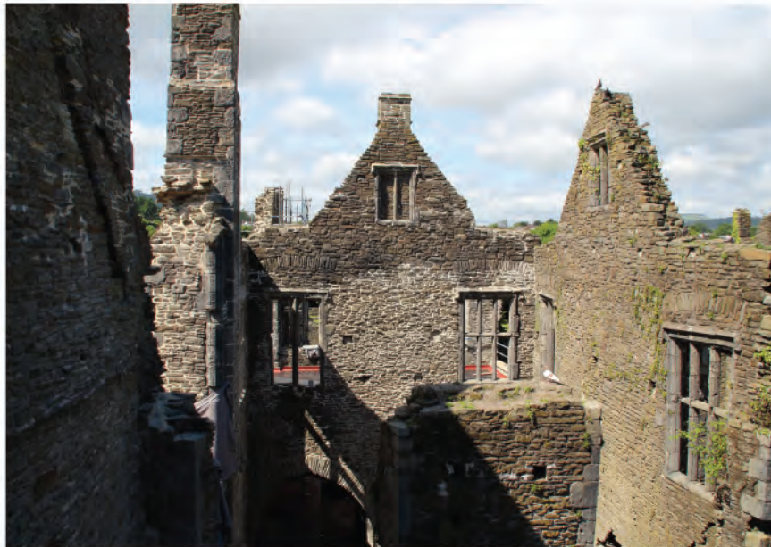
Plate 157. View of south facing elevation of south wall of vaulted bridge. Looking north.
