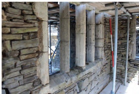
Plate 99. View of square headed window in east wall at first floor level (107). Looking northwest.
