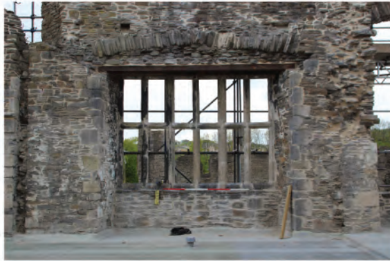
Plate 66: View of square headed late Tudor window (8) in west wall. Looking west.
