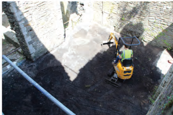
Plate 244. Working shot during clearance of vegetation in area of east wing of Abbot's House. Looking northeast.
