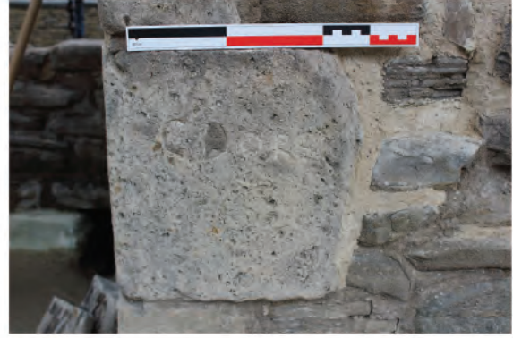
Plate 144. Detail of graffiti in sandstone block in east wall (188). Looking east.
