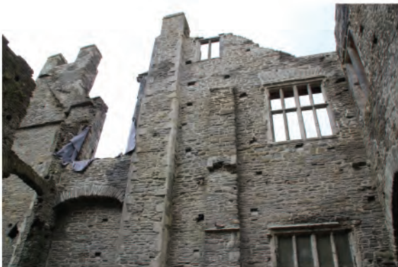
Plate 127. General view of central part of east wall following scaffold removal. Looking west.
