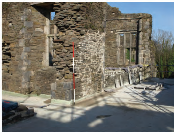
Plate 160. View of south facing internal elevation of north wall of bridge. Looking east.
