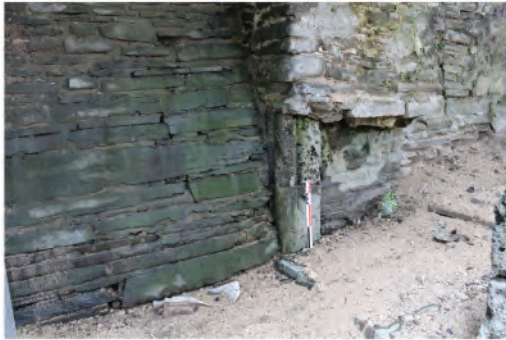
Plate 115. Detail view showing moulded Sutton stone below buttress (102) in east wall. Looking northwest.
