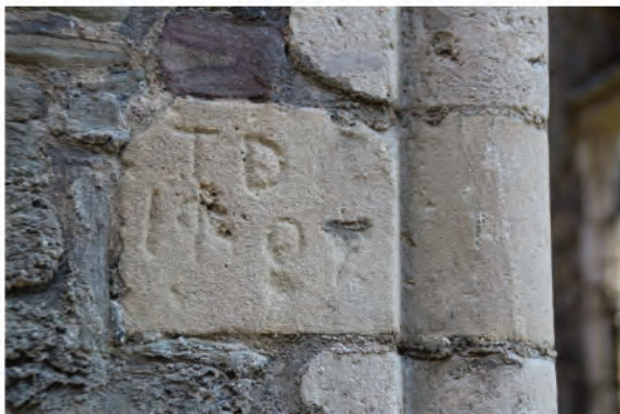
Plate 173. Graffiti in replacement sandstone ashlar quoin in central support pier of bridge. Looking north.
