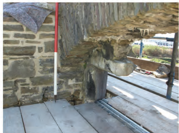
Plate 25: Remains of top and base jamb of oriel window (6) in west wall. Looking southwest.
