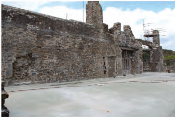
Plate 62: View of east facing elevation of west wall following removal of scaffolding. Looking northwest.
