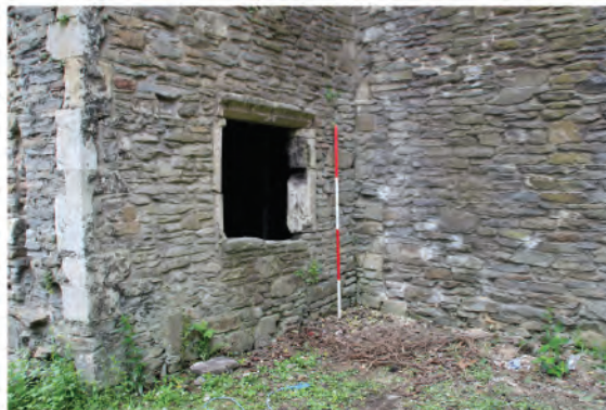
Plate 199. View of square window opening in northern elevation of Abbot's Stairwell. Looking southwest.
