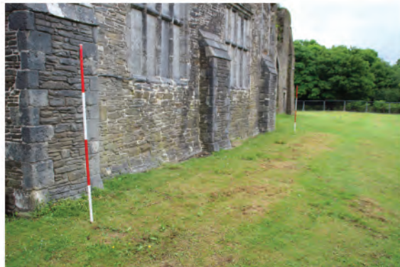
Plate 219. Oblique view of south wall and area of proposed drainage trench. Looking eastwards.
