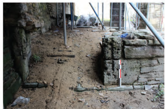
Plate 114. View of former opening in lateral cross wall at foot of east wall at base of buttress. Note moulded base orders. Looking north.
