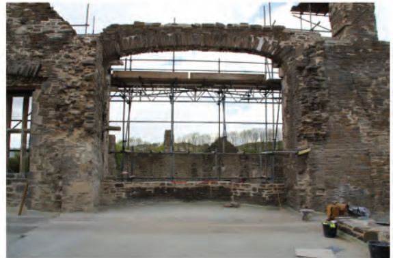
Plate 63: View of large oriel window (6) in west wall during consolidation work. Looking west.
