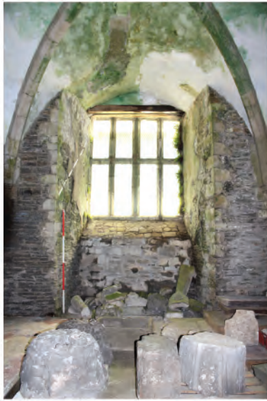
Plate 260. East window of South wall in undercroft prior to lintel replacement. Looking south
