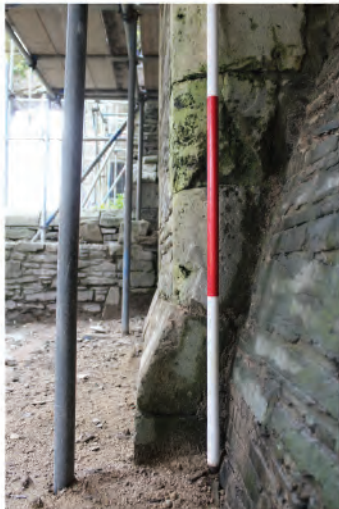
Plate 117. Detail of corner moulding at base of chimney showing pyramidal stop. Looking south.
