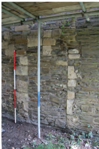
Plate 48: Blocked in doorway in west wall at far southern end (49). Looking eastwards.
