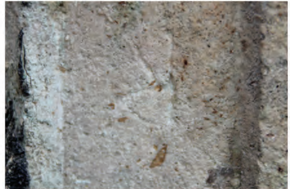
Plate 73: Detail shot showing mason's mark of an inverted letter 'R'. Found in side jamb of large oriel window (6). Looking southwest.
