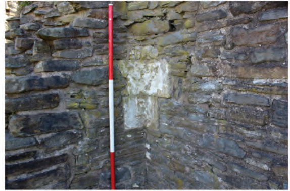
Plate 154. Detail shot showing corner of north wall where the former 13th century vault corbel would have once been set. Original ashlar quoins still present. Looking southeast.
