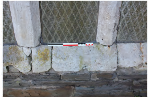
Plate 29: Detail of base jamb in late Tudor window in west wall ground floor (24).
