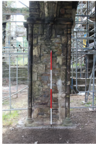
Plate 166. View of central bridge support pier at south side of bridge. Looking south.
