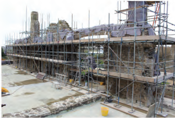
Plate 60: Working shot of east facing elevation of west wall during consolidation work. Looking southwest.
