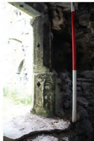
Plate 211. Detail view of replacement jamb in square window of Abbot's Stairwell in north facing ground level. Looking eastwards.
