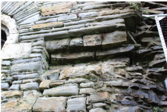
Plate 102: Remains of former spring of arch (135) in east facing external elevation of east wall alongside Slype passage. Looking west.
