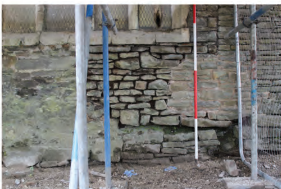
Plate 114. View of area of repair below late Tudor window in east wall (104). Looking west.
