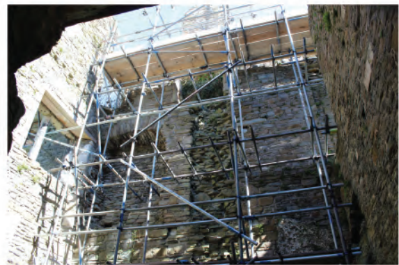
Plate 41: View of southern end of west facing elevation showing features in area of first floor. Looking eastwards.
