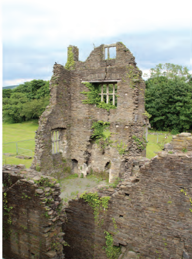
Plate 4. View of northeast range of Tudor Mansion during consolidation work. Looking northeast.
