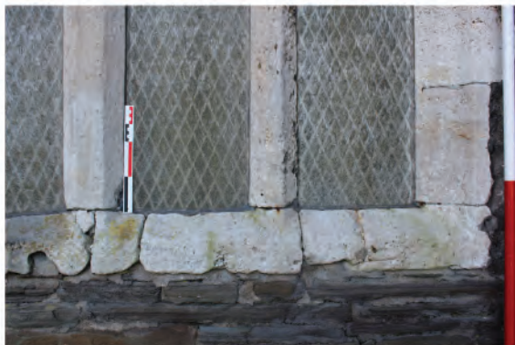
Plate 30: Detail of base jambs and mullions in late Tudor window in west wall ground floor (24).
