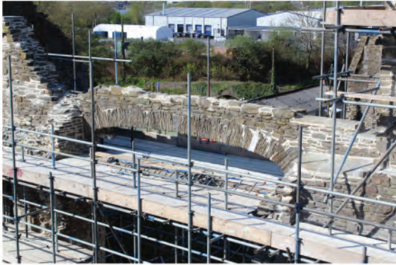
Plate 32: View of long relieving arch (2) of oriel window in west wall at first floor level. Looking westward from east wall.
