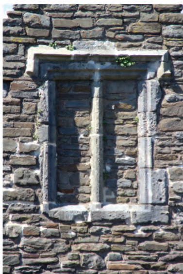
Plate 161. Detail shot of false window (160) in south facing elevation of south wall of bridge. Looking north.
