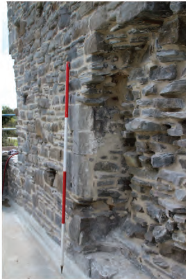
Plate 78: Detail shot showing ashlar quoins of former blocked in 13th century dormitory window (200) in west wall. Looking south.
