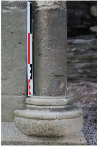
Plate 169. Detail shot showing moulding of base column on bridge central support pier. Looking west.
