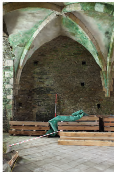
Plate 185. Blocked doorway in north wall of undercroft that once gave access to Novice Room. Looking north.
