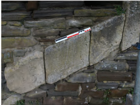
Plate 16: Detailed view of remains of Sutton stone handrail alongside Day Stairs in West wall. Looking southeast.
