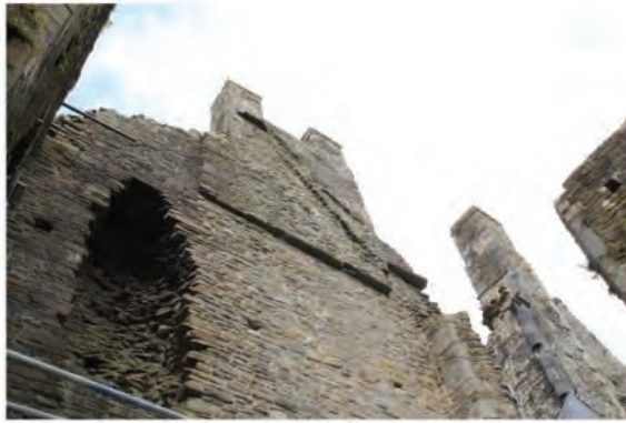
Plate 131. View looking up towards chimney pair and vice passage in east wall. Looking westwards.
