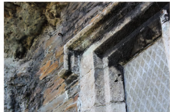
Plate 31: Detail of hood and return label in late Tudor window in west wall ground floor (24).
