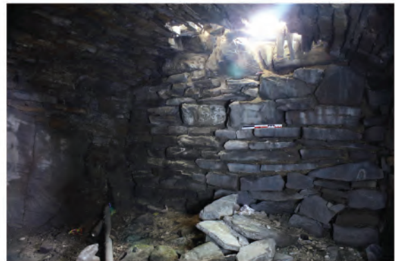
Plate 191. View of north facing elevation of cell / vault beneath Slype passage. Looking northeast.
