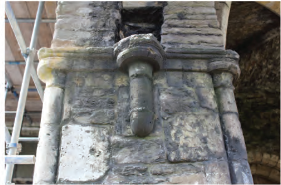
Plate 170. Detail shot showing decorative moulded corbel at top of bridge central support pier. Looking west.
