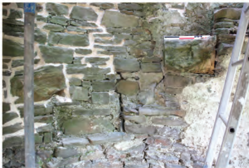
Plate 214. View of remains of steps from newel stair in Abbot's Stairwell. Looking eastwards.
