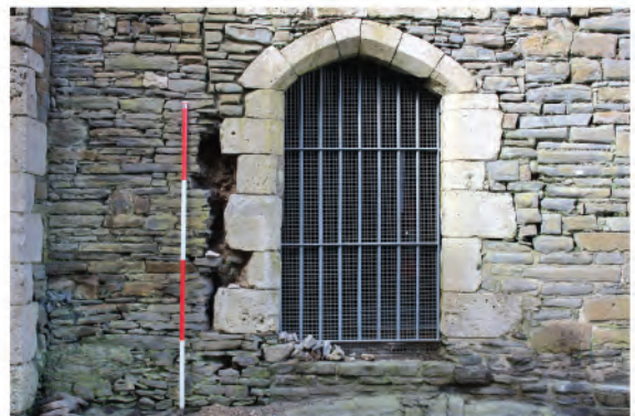
Plate 92: Detailed shot of doorway (136) into Novice Room in east wall. Looking west.
