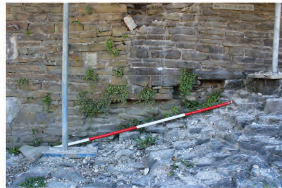
Plate 17: Detailed view of remains of Monk's Day Stairs in West wall. Looking east.
