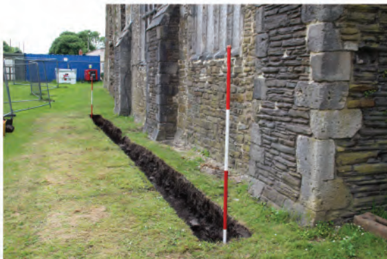
Plate 228. View of drainage trench following removal of redeposited material to required depth. Looking westwards.
