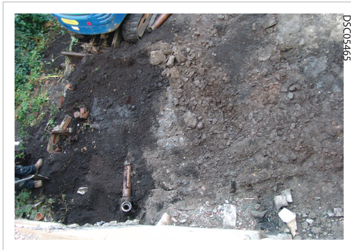
Plate 01: Initial excavation viewed from first floor. SW of plot into garden soil [104] exposing soil pipe [107] in cut [108] with fill [109]
