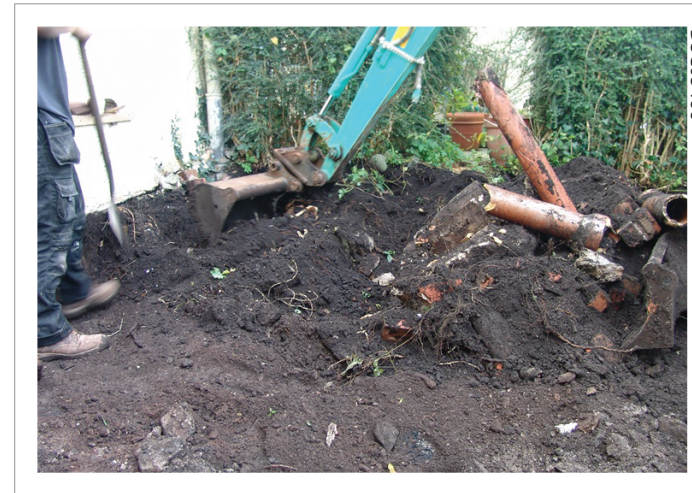
Plate 02: Initial excavation showing fill [109] and pipes [107] with brick supports. 6" soil pipe in salt glaze with later plastic insertions
