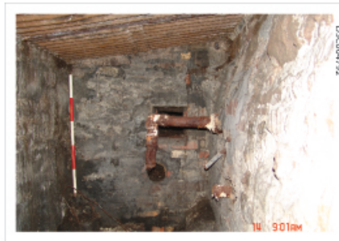
Plate 06: Boiler house, Bulging west wall of church
