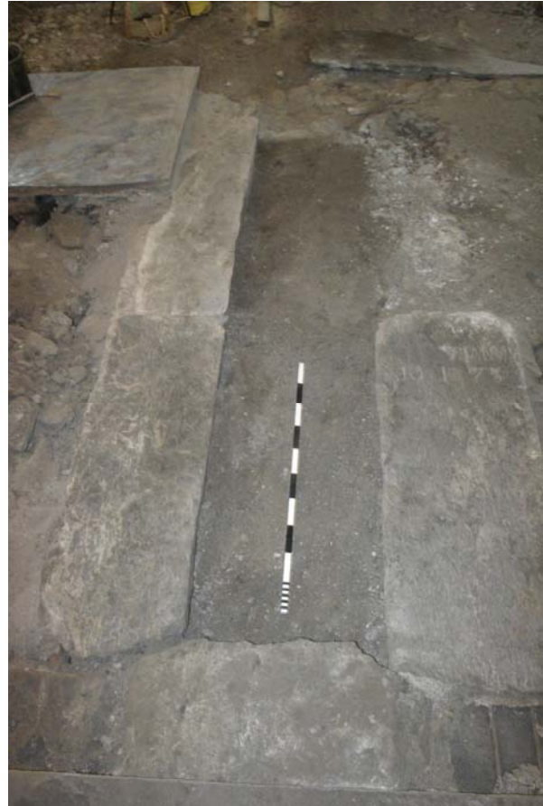
Fig. 7 Stone slab floor foundation at the entrance to the nave with one grave slab removed (and the photo scale introduced) to reveal the rubble make-up, viewed from the north. Photo CPAT 3805-0012
