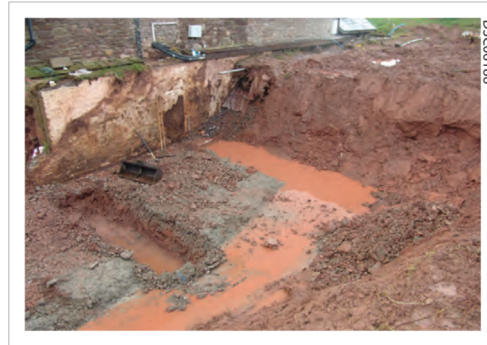
Plate 06: Overview of trenches 1,2 & 7 showing excavation to rear retaining wall, Fill evident top centre
