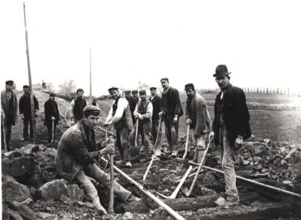
Figure 8: Platelayers at work on the Mountsorrel branch line in Leicestershire (source: http://heritage-centre.co.uk/visit-us/a-brief-history-of-the-railway/#jp-carousel-1665 )
