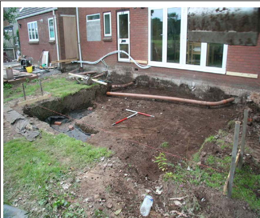
Fully excavated foundation trench and removed concrete path with redirected pipe. Roman surface under black geotextile middle left (looking south- east)
