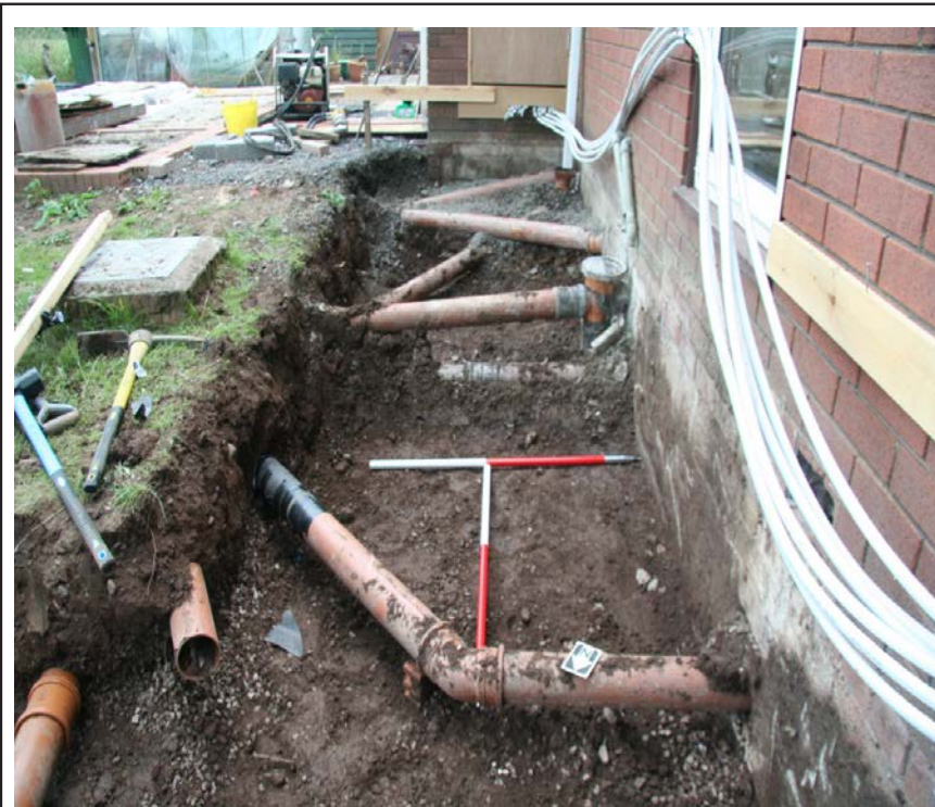
Fully excavated southern foundation trench under former concrete path with pipe work (looking south)
