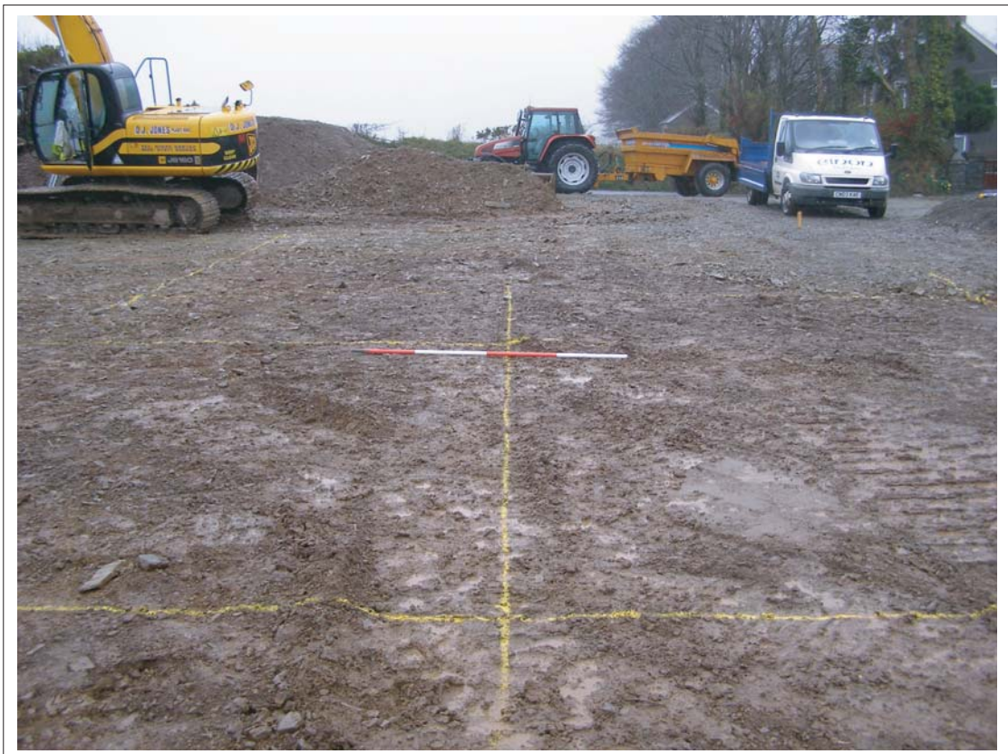
Plate 2: East end of site after removal of topsoil, looking north east. Scale 2m
