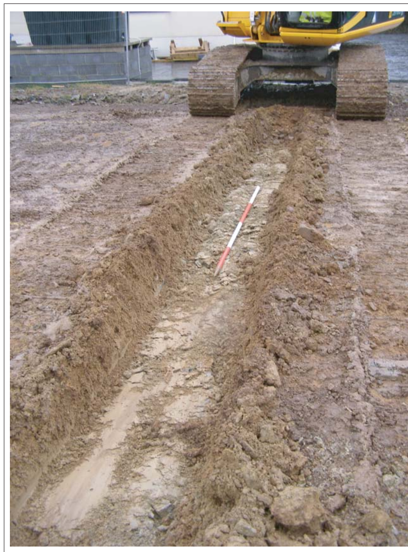
Plate 4: Southern foundation trench, showing subsoil removed to the top of the natural, looking east. Scale 2m
