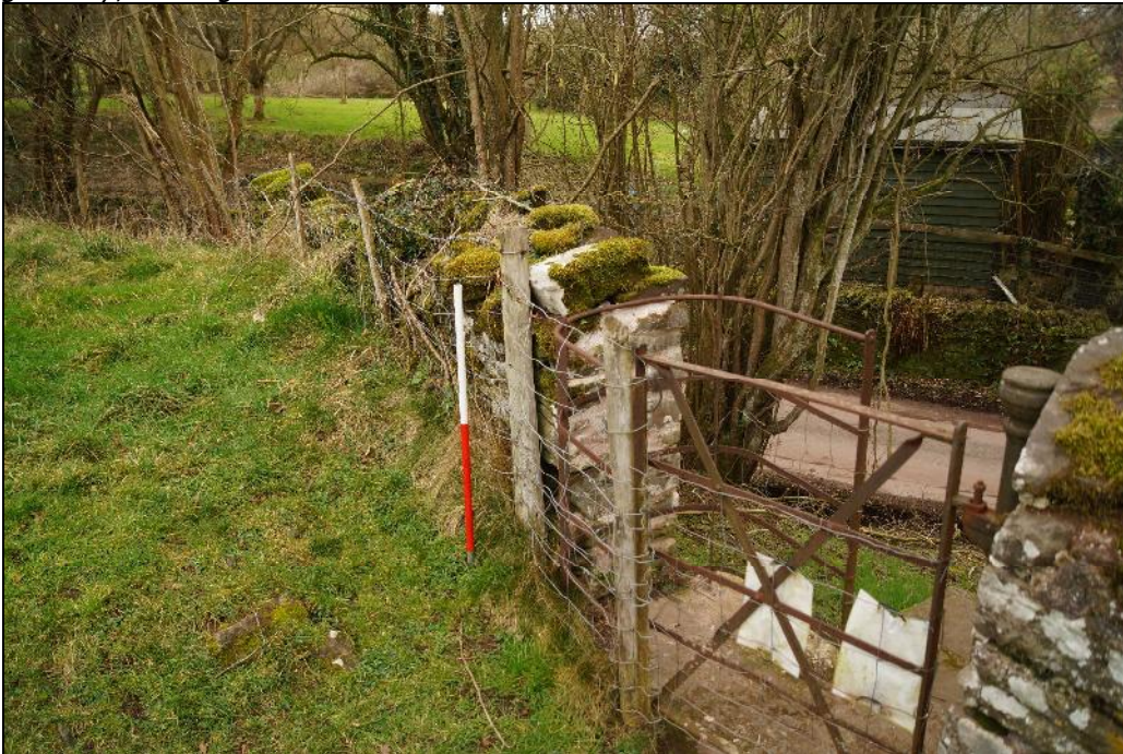
Plate 36: SEL2018_136, Repointed section of the western boundary wall just to the south of the gateway, looking southwest.
