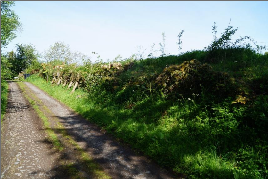
Plate 5: SEL2018_105, The southern part of the boundary wall looking west from the lane to the south. Note the shoring supporting the wall in the centre of the photograph.
