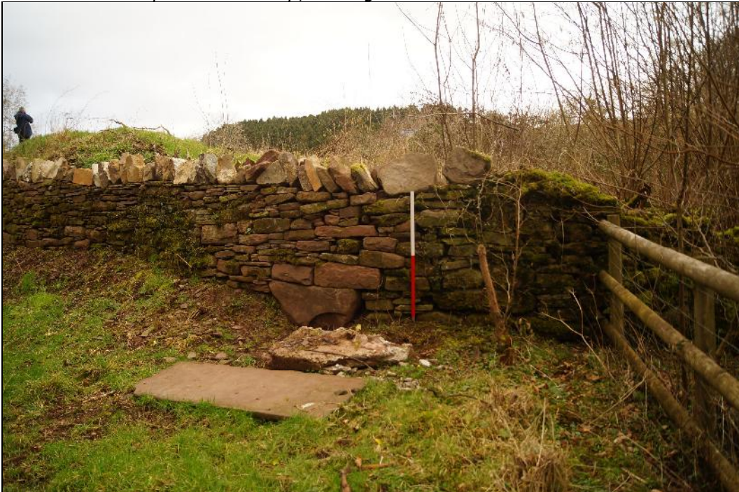
Plate 32: SEL2018_132, After restoration of the wall, with larger stones marking the location of the steps, looking northwest.
