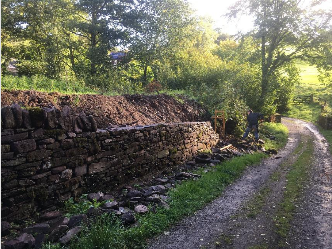
Plate 25: SEL2018_125, Restored section D and starting to take down section E, looking east. The height of the ground can be seen behind section D.
