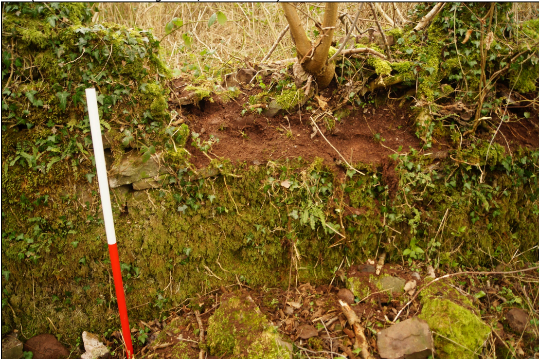
Plate 42: SEL2018_142, Loose stones removed from the section of the east wall to be repaired at SOXXXX, looking east (RV Williams Drawing 3892/08 Note 2.0)
