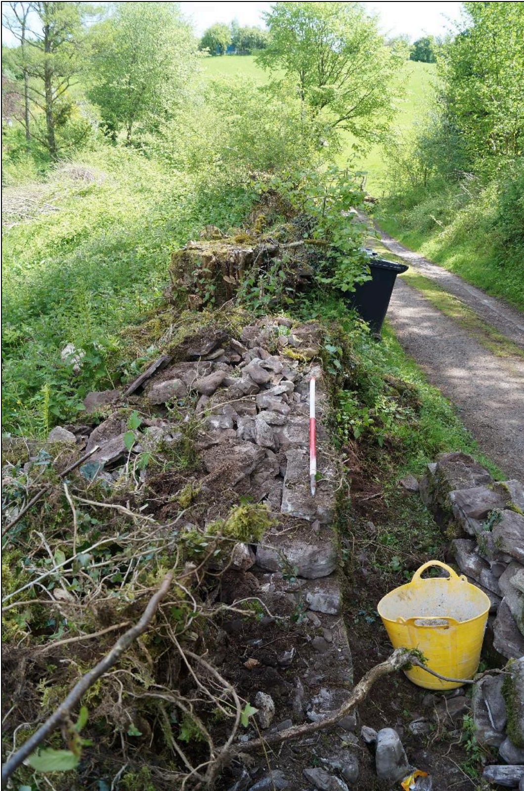
Plate 14: SEL2018_114, Next section of wall dismantled, less material needed to be removed here, looking east.
