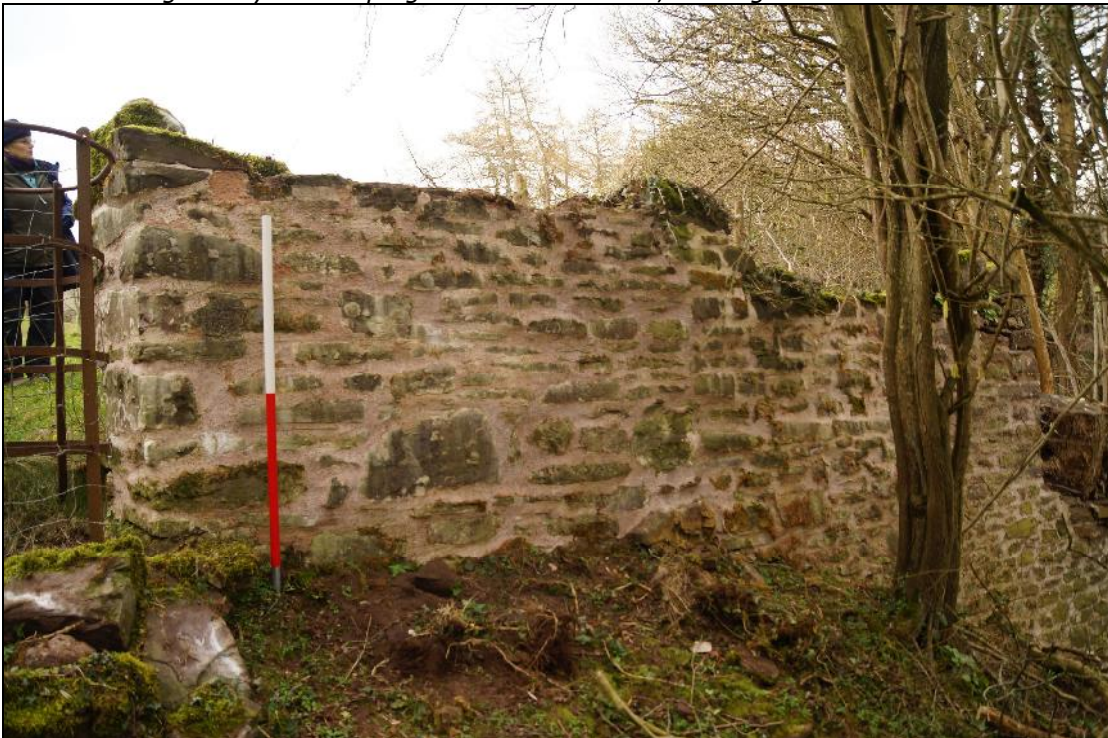
Plate 38: SEL2018_138, Repointed section of the western boundary wall just to the south of the gateway with coping stones removed, looking south-southeast.
