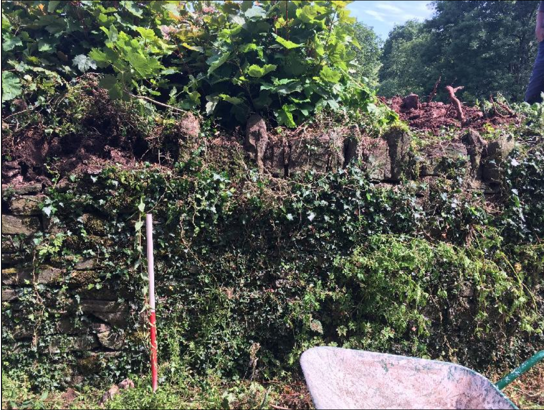
Plate 20: SEL2018_120, The wall still stood to full height at this point and the pattern of the coping stones changed, looking north.
