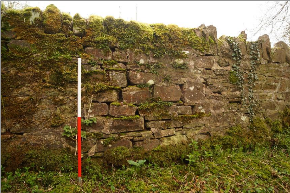
Plate 39: SEL2018_139, Bulge in the east wall at SOXXXX, looking east (RV Williams Drawing 3892/08 Note 2.0) .
