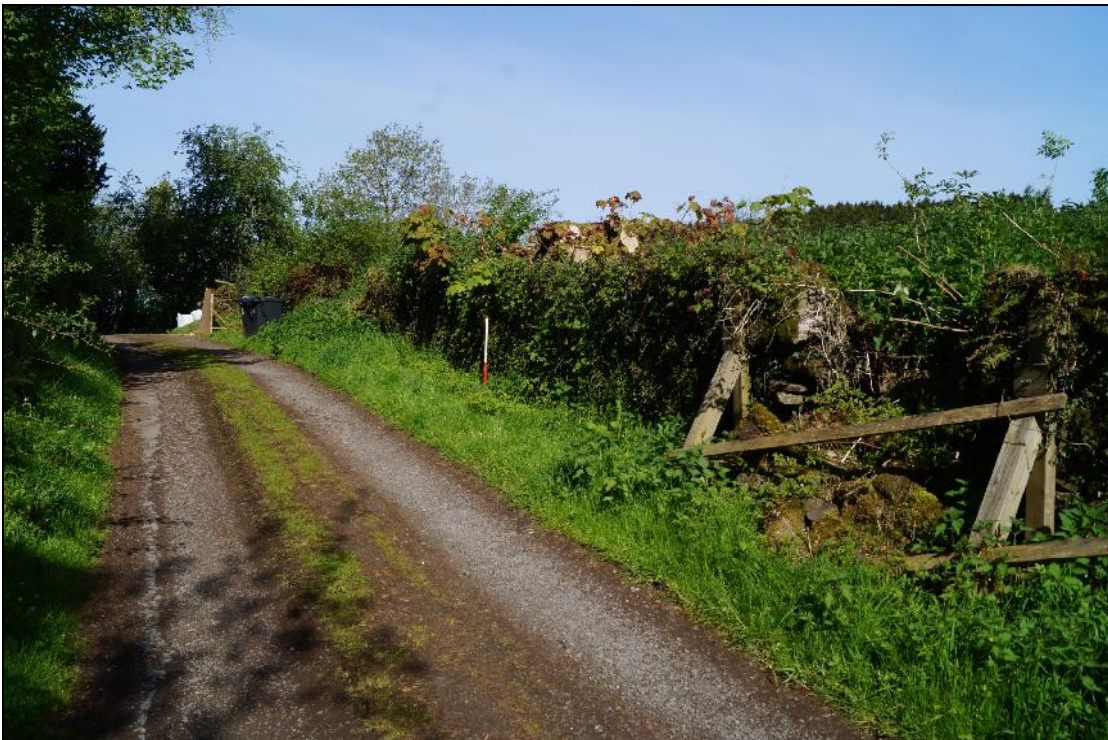
Plate 4: SEL2018_104, The southern part of the boundary wall looking west from the lane to the south. Note the shoring supporting the wall to the right of the photograph.
