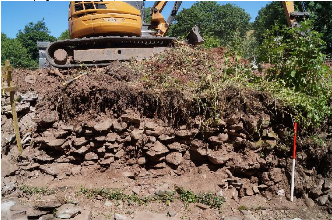
Plate 21: SEL2018_121, Section of the wall with the south face removed to show the rubble core of the wall, looking north. Occasional large stones act as tie stones.
