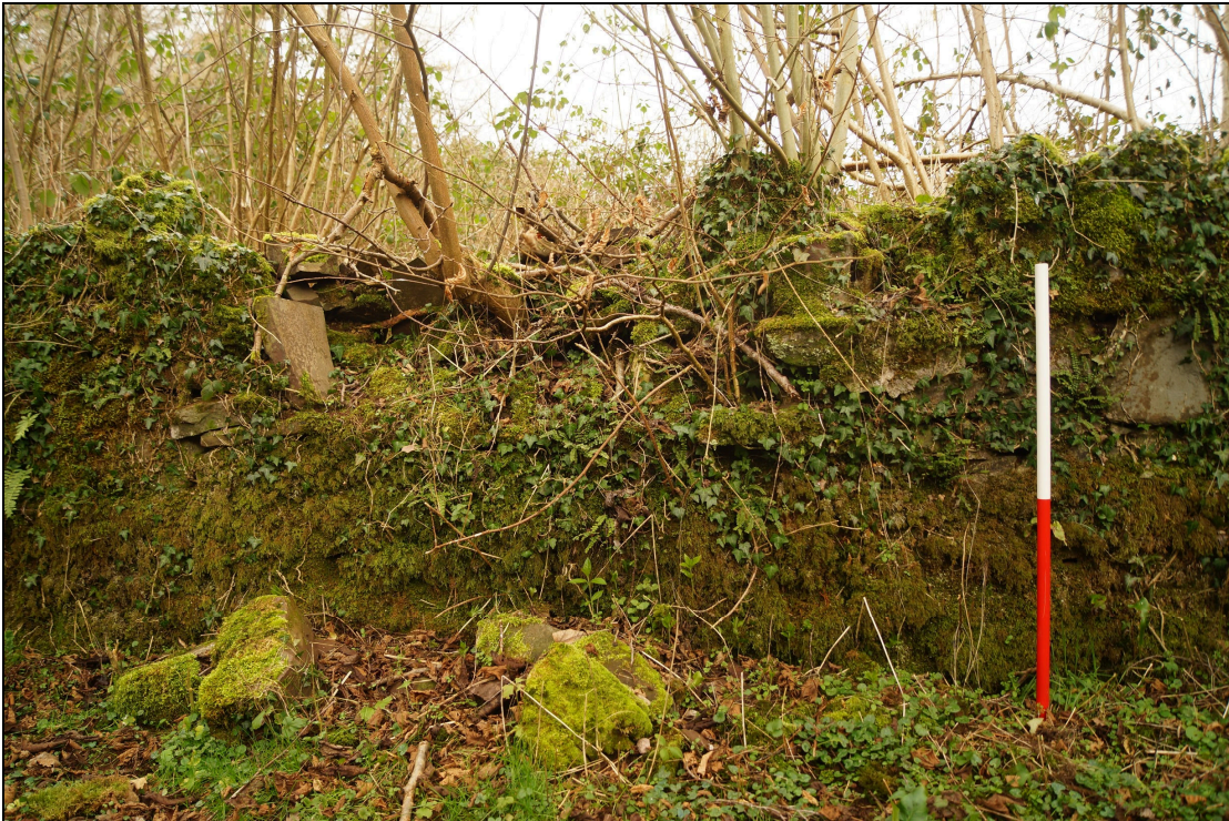
Plate 41: SEL2018_141, Section of the east wall to be repaired at SOXXXX, looking east (RV Williams Drawing 3892/08 Note 2.0)
