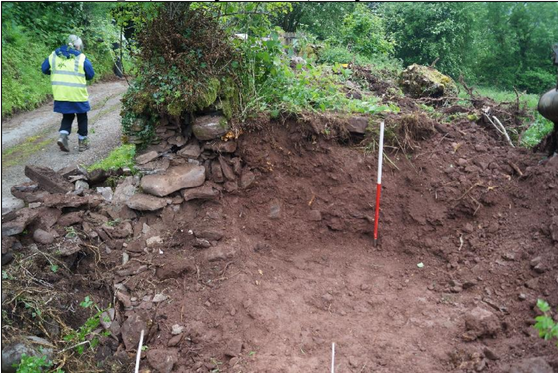
Plate 18: SEL2018_118, Tree bole and roots removed and section through wall and earth behind excavated, looking west.
