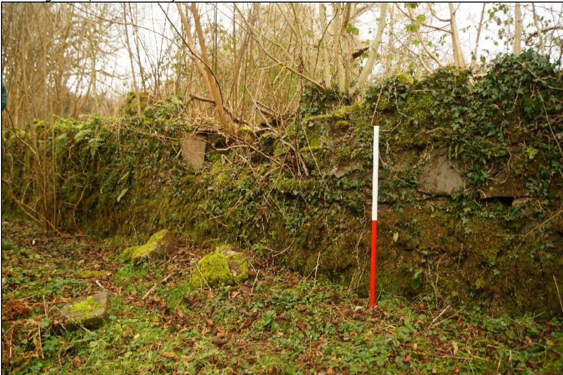
Plate 40: SEL2018_140, Section to eastern boundary wall to be repaired, looking southwest (RV Williams Drawing 3892/08 Note 1.0)
