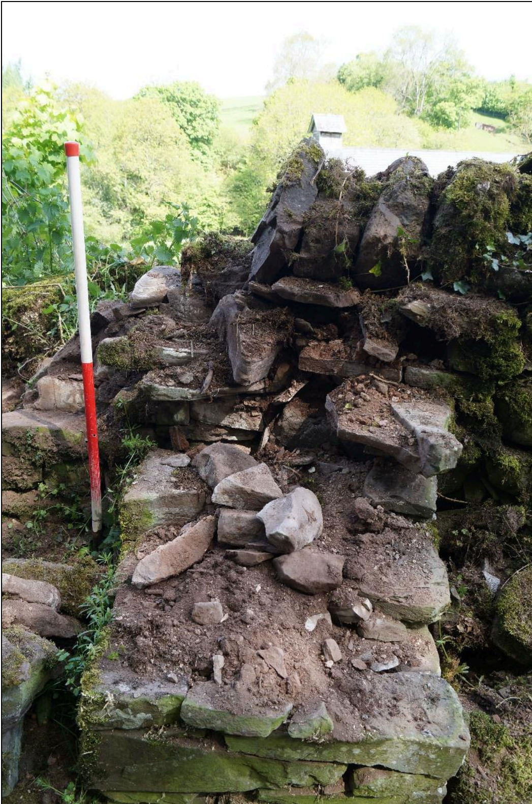
Plate 11: SEL2018_111, Dismantling the short section of wall at right angles to the boundary wall, looking north.
