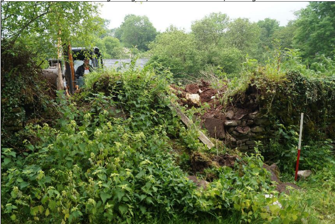
Plate 16: SEL2018_116, Removing large tree bole and roots from the inside of the wall, the wall in this section was already partially collapsed, looking northeast.
