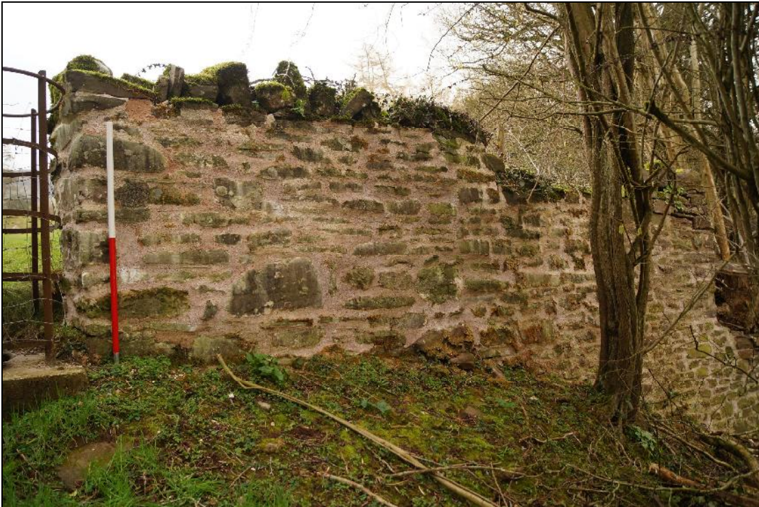
Plate 37: SEL2018_137, Repointed section of the western boundary wall just to the south of the gateway with coping stones to be reset, looking south-southeast
