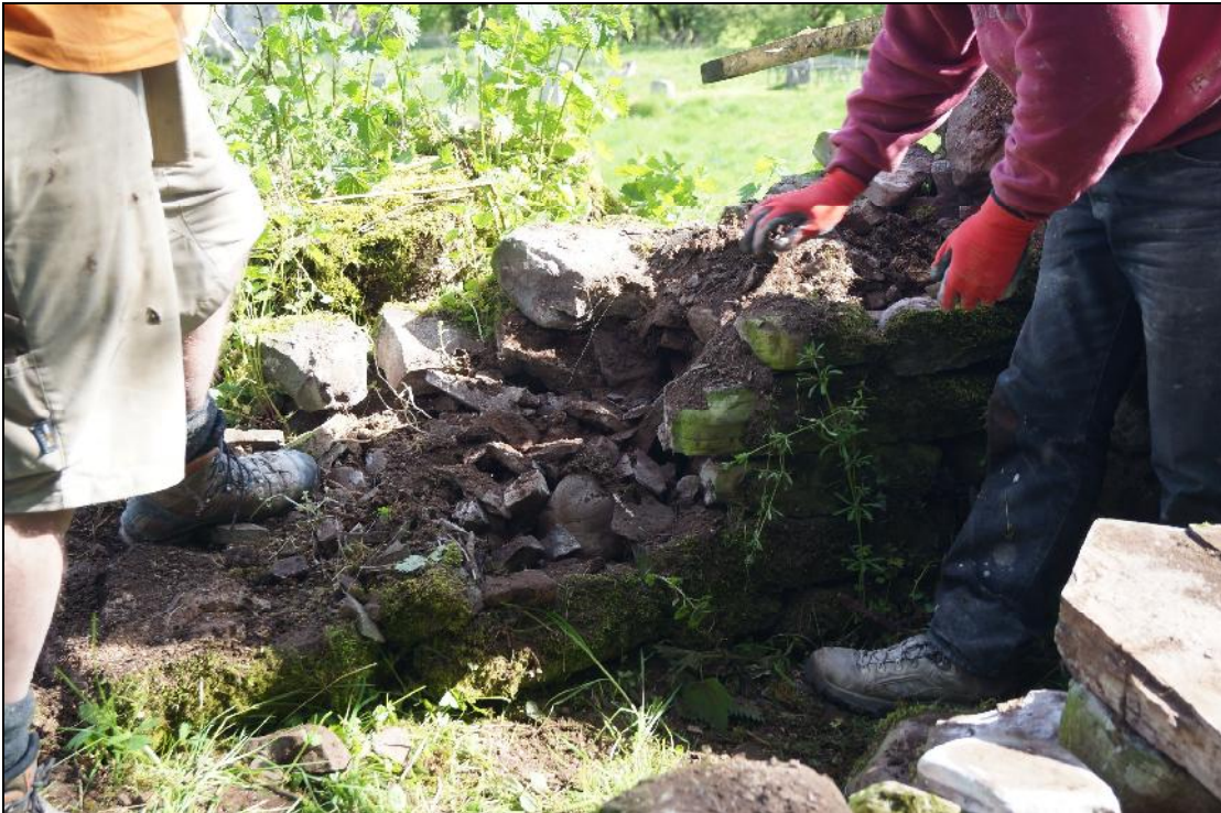
Plate 7: SEL2018_107, dismantling the wall to the east of the gateway in the southern boundary, looking northeast.
