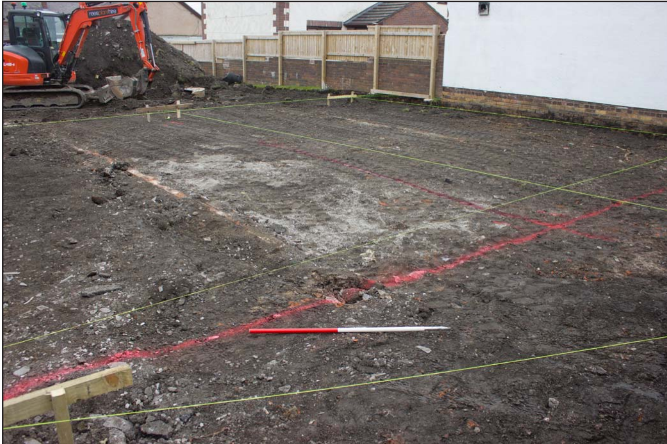
Plate 01: Pre excavation shot of site east of the Roman Catholic Presbytery, Brunswich Road, Buckley, - from the southwest - 1.00 scale
