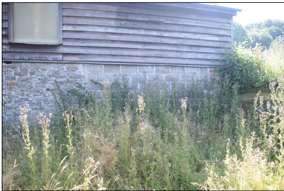
Fig. 5 Cart shed, viewed from the west showing wall section rebuilt in blockwork Photo CPAT 4942-017
