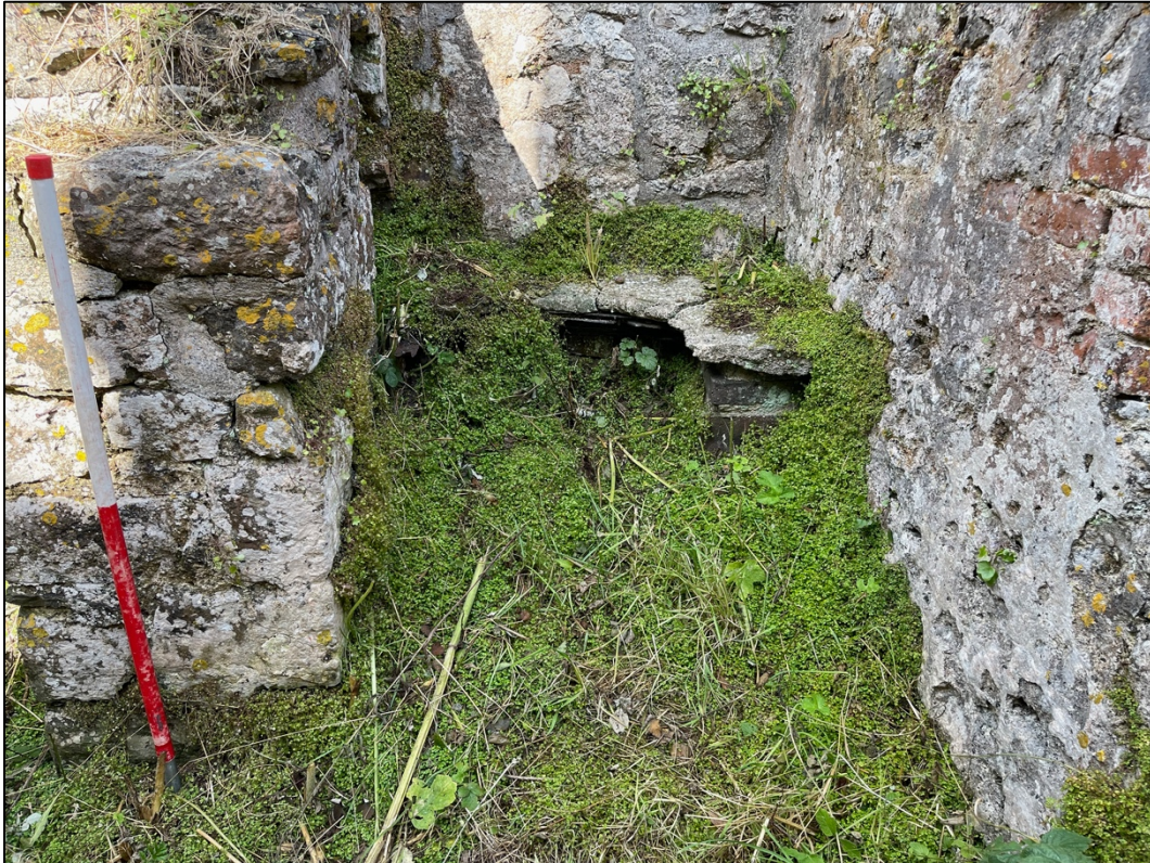
Plate 14. Location 15 Medieval Tower/19 th Century Kitchen, view of laundry copper stone hearth.
