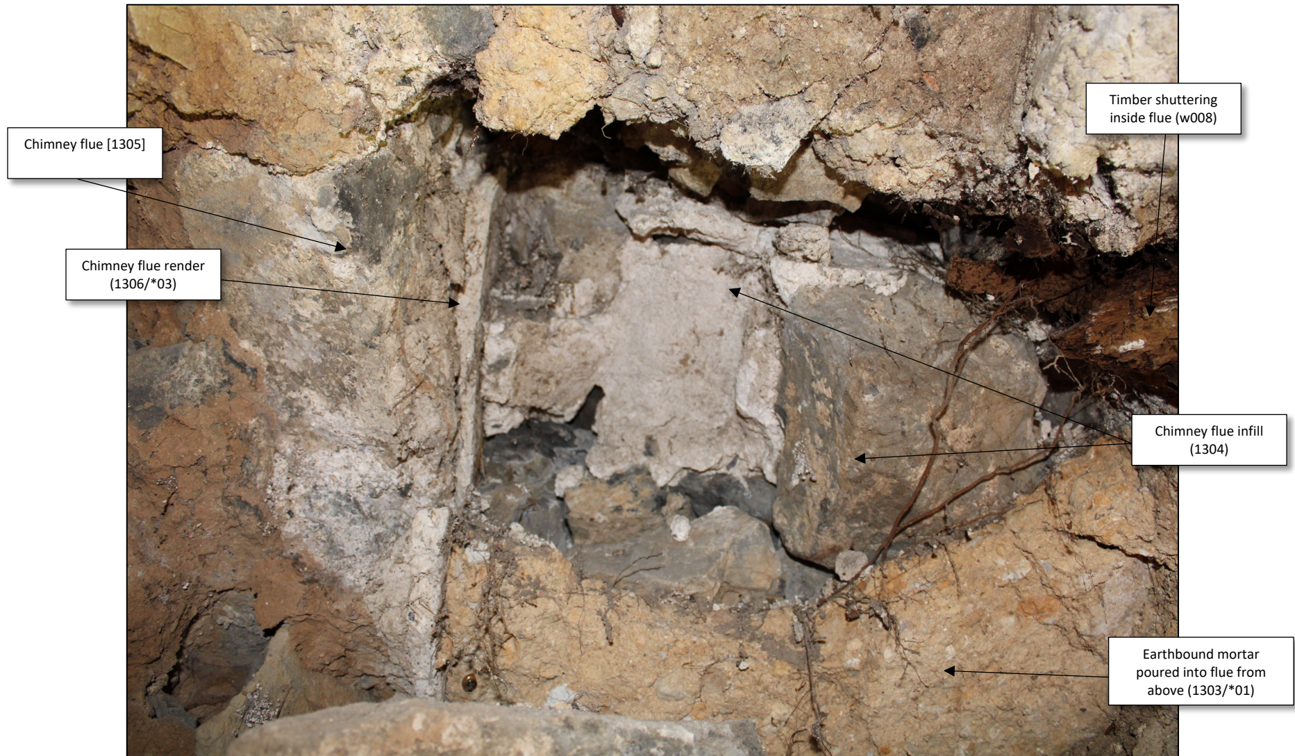
Plate 6. Location 13 NW Service Room, close view of chimney flue [1305], internal lime render (1306) and earthbound mortar infill (1303).
