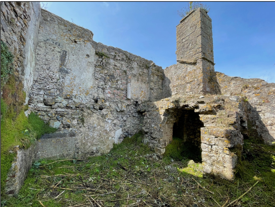
Plate 11. Location 15 Medieval Tower/19 th Century Kitchen, view of SE facing fireplace and chimney.
