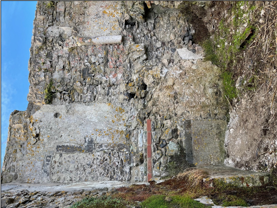
Plate 10. Location 15 Medieval Tower/19 th Century Kitchen, view of NE facing wall repaired.
