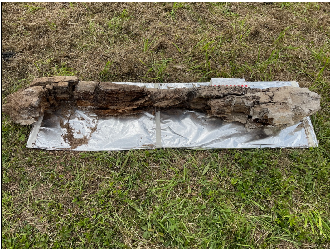
Plate 21. Location 13 NW Service Room, worked timber (w006) reused inserted above a former hearth or fireplace and was found in an advanced stage of decay.
