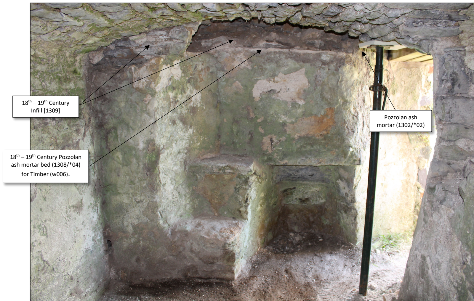
Plate 4. Location 13 NW Service Room, view to SW of hearth/fireplace following removal of Timber (w006).
