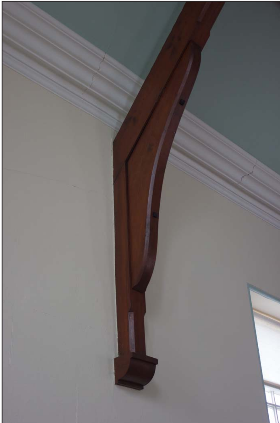
Plate 49: Roof truss support corbel within Gwynfa Chapel, Pen-y-ffordd, Holywell, Flintshire - from the southeast - no scale
