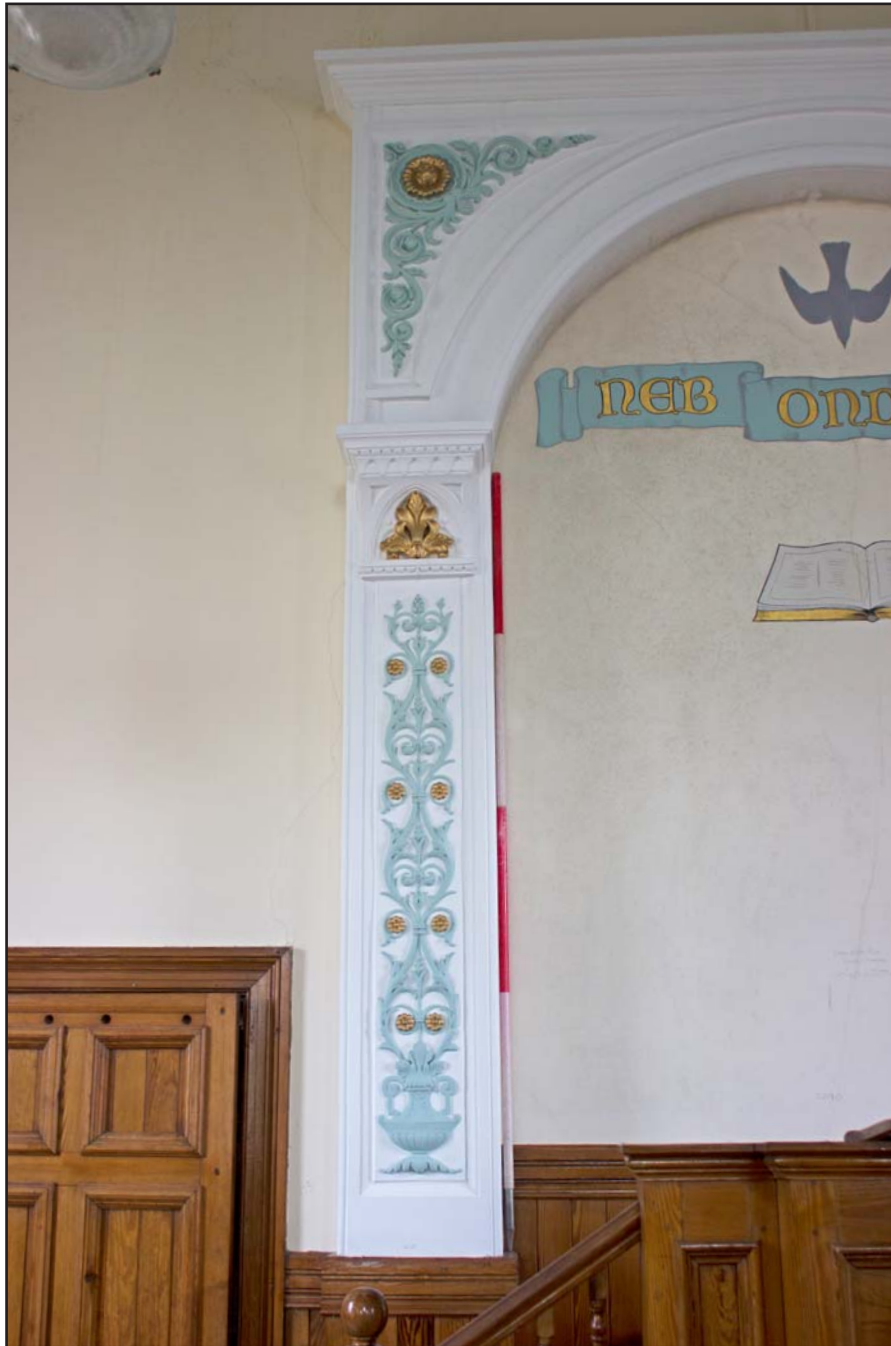
Plate 30: Detail of arch within Gwynfa Chapel, Pen-y-ffordd, Holywell, Flintshire - from the south - 2.00m scale
