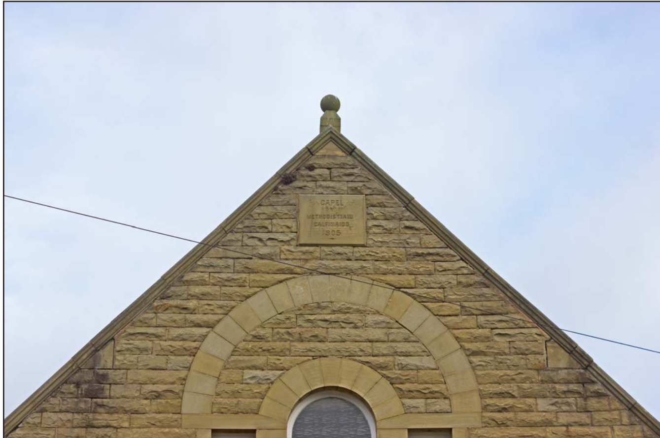
Plate 13: Finial & date stone, southern elevation, Gwynfa Chapel, Pen-y-ffordd, Holywell, Flintshire - from the south - no scale
