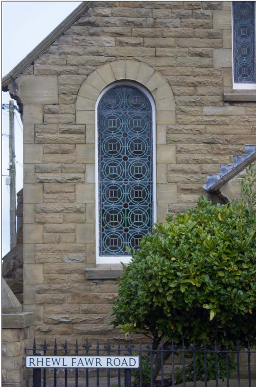
Plate 15: Ground floor window, southern elevation, Gwynfa Chapel, Pen-y-ffordd, Holywell, Flintshire - from the south- no scale
