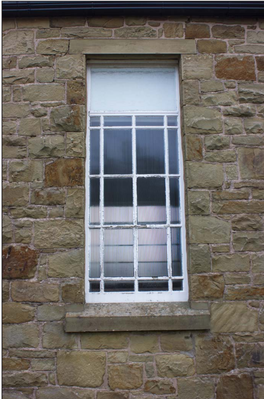
Plate 16: Ground floor window, western elevation, Gwynfa Chapel, Pen-y-ffordd, Holywell, Flintshire - from the west - no scale
