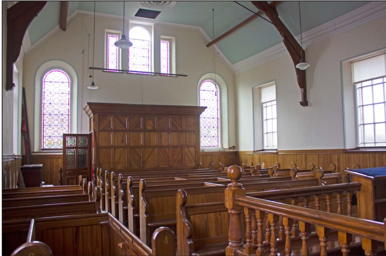
Plate 19: Main Chapel body, Gwynfa Chapel, Pen-y-ffordd, Holywell, Flintshire - from the north - 2.00m scale
