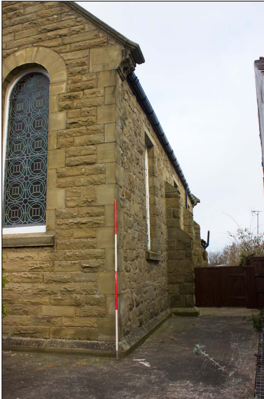
Plate 10: External eastern elevation of Gwynfa Chapel, Pen-y-ffordd, Holywell, Flintshire - from the southeast - 2.00m scale
