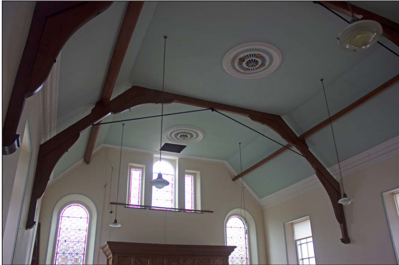
Plate 45: Oblique shot of the ceiling of Gwynfa Chapel, Pen-y-ffordd, Holywell, Flintshire - from the northeast - no scale
