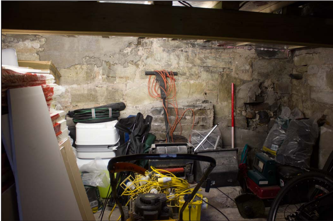
Plate 56: Boiler room, Gwynfa Chapel, Pen-y-ffordd, Holywell, Flintshire - from the northwest - no scale
