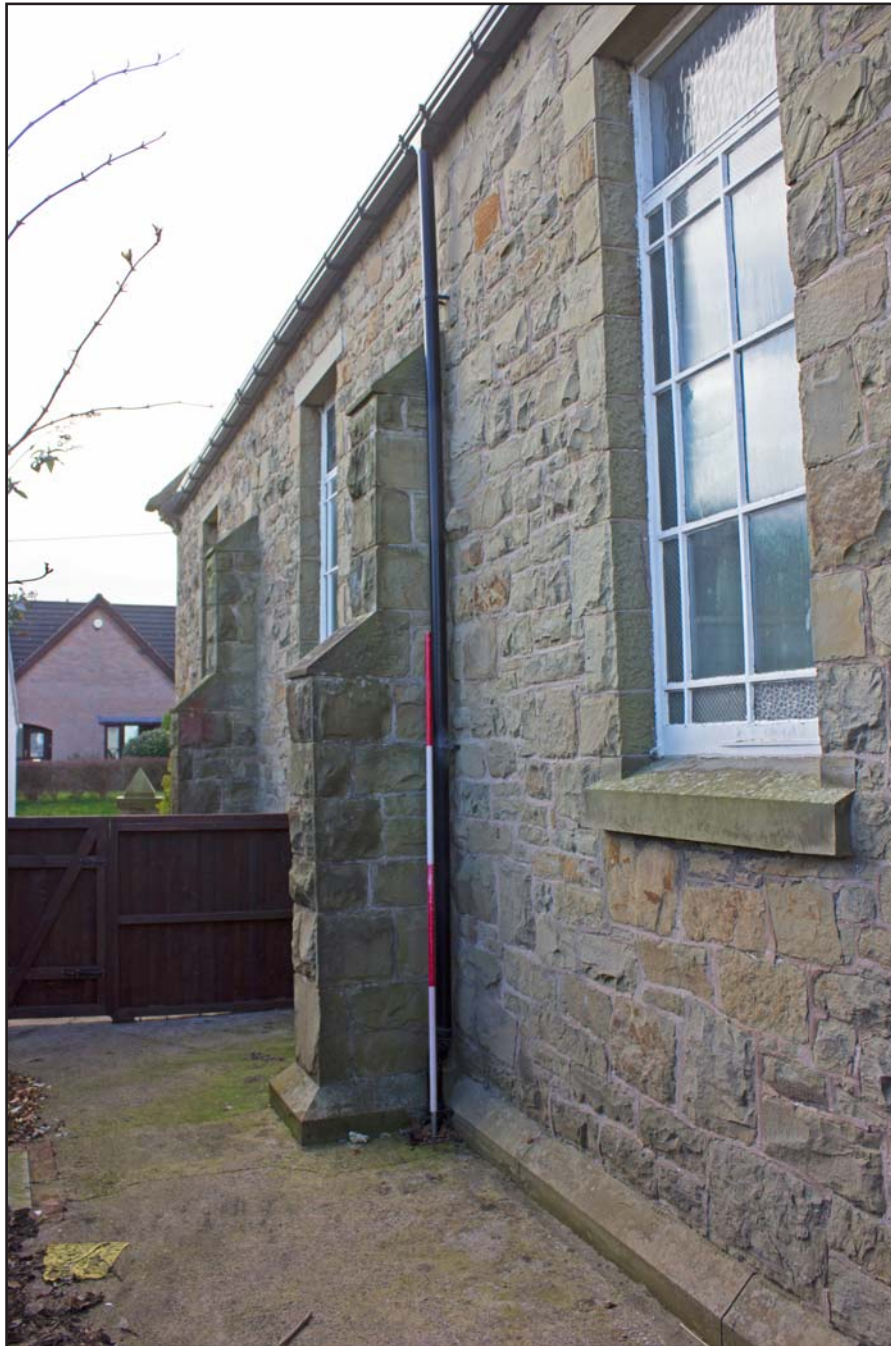
Plate 09: External eastern elevation of Gwynfa Chapel, Pen-y-ffordd, Holywell, Flintshire - from the northeast - 2.00m scale
