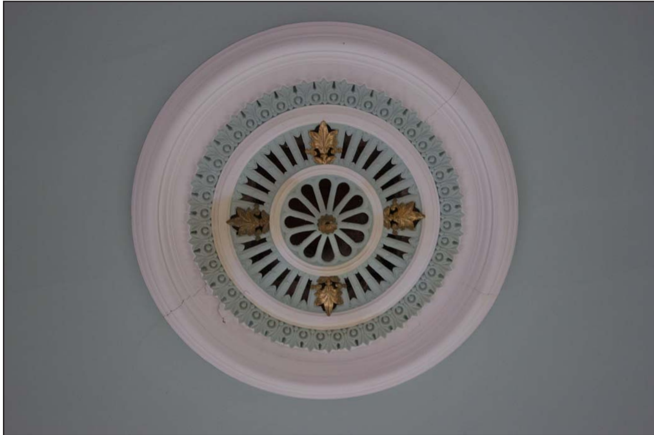
Plate 47: Central ceiling rose within Gwynfa Chapel, Pen-y-ffordd, Holywell, Flintshire - from the north - no scale
