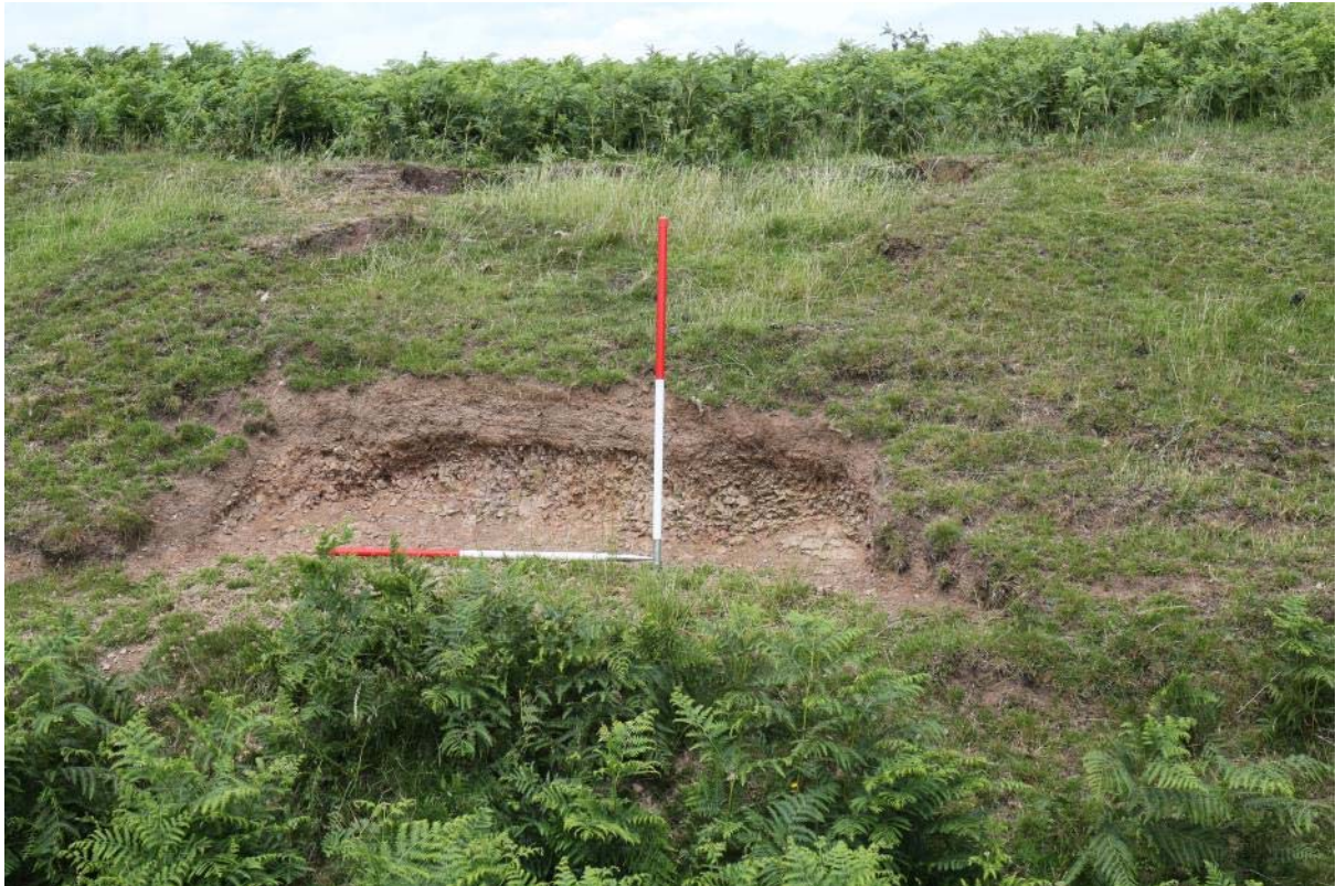
Locations 4, 5 & 6, before repair, IMG_7466, 18.07.2015
