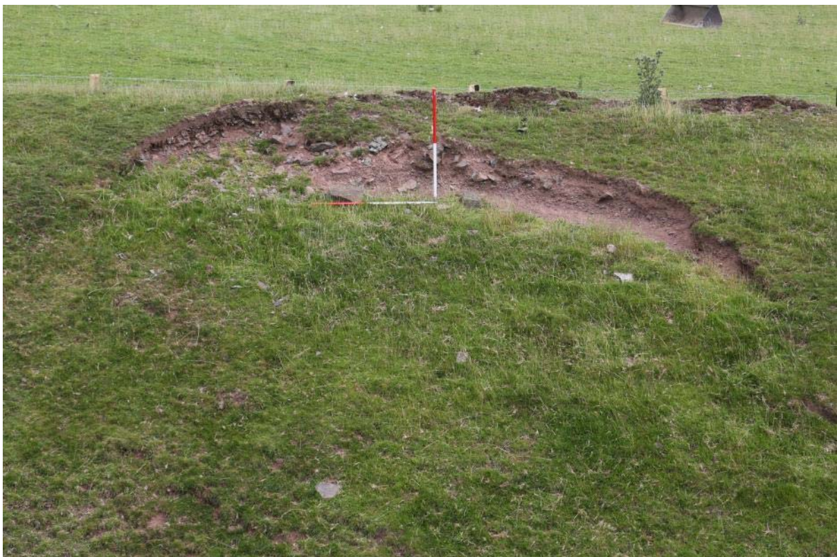
Location 10, before repair, IMG_7469, 18.07.2015
