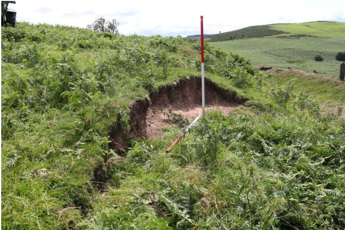
Location 7, before repair, IMG_7465, 18.07.2015
