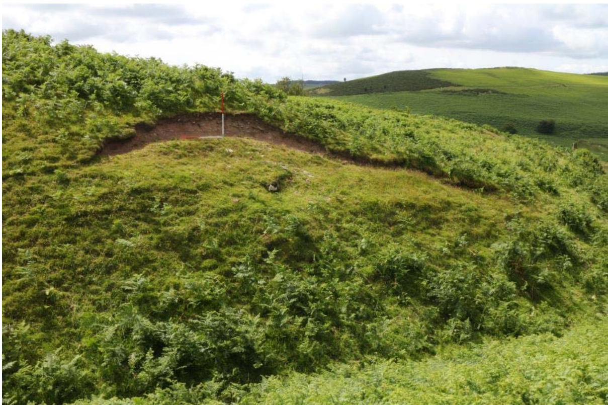
Location 8, before repair, IMG_7457, 18.07.2015
