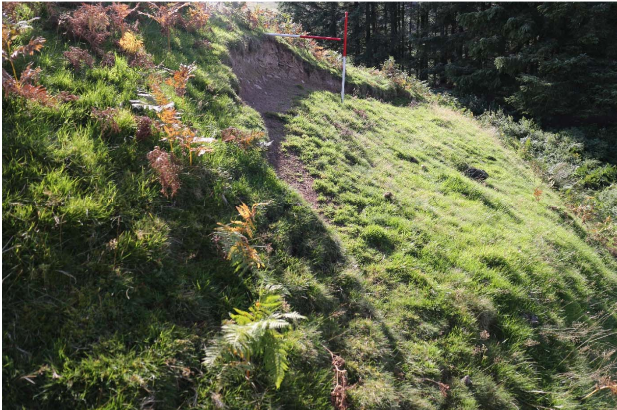
Location 8, before repair, IMG_2454, 02.10.2014
