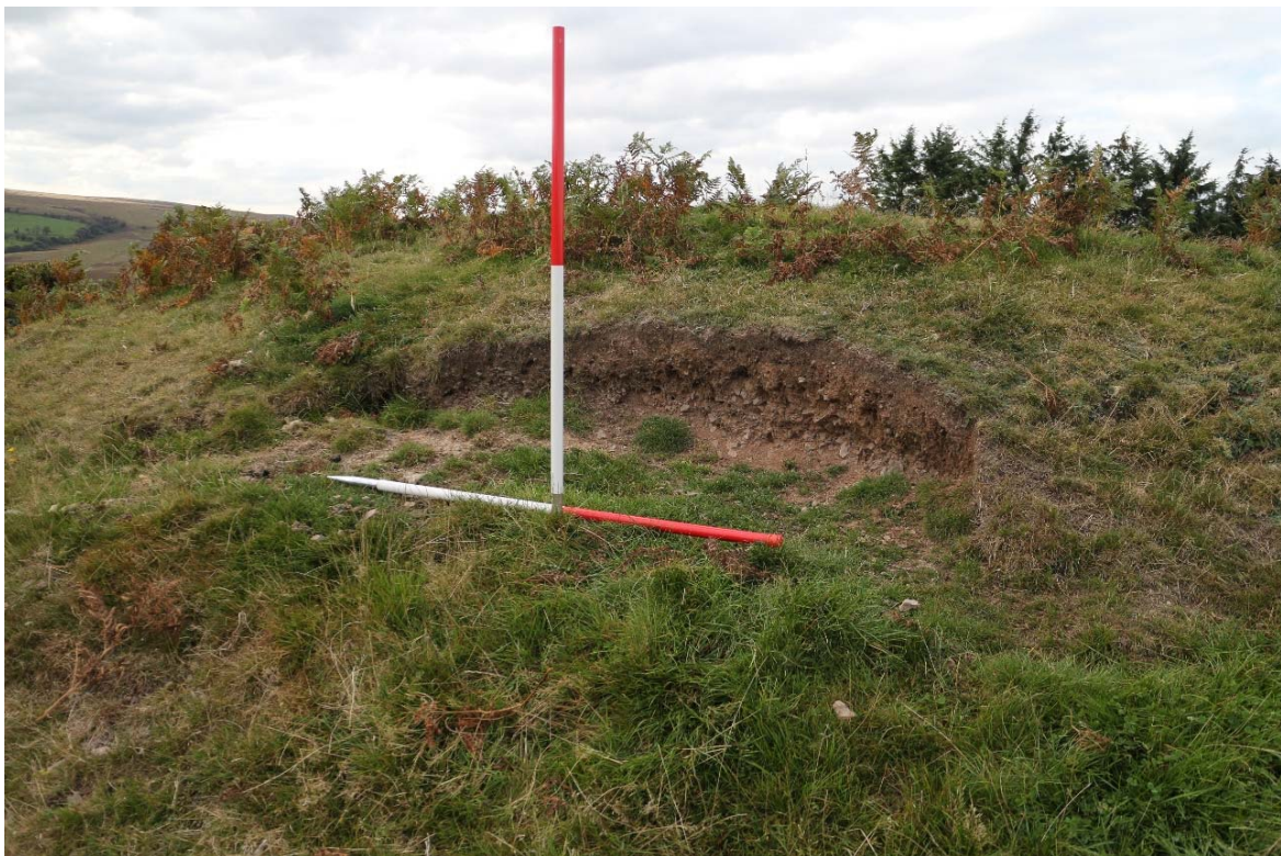
Location 2, before repair, IMG_2482, 02.10.2014
