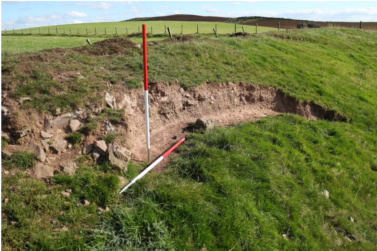
Location 10, before repair, IMG_2442, 02.10.2014
