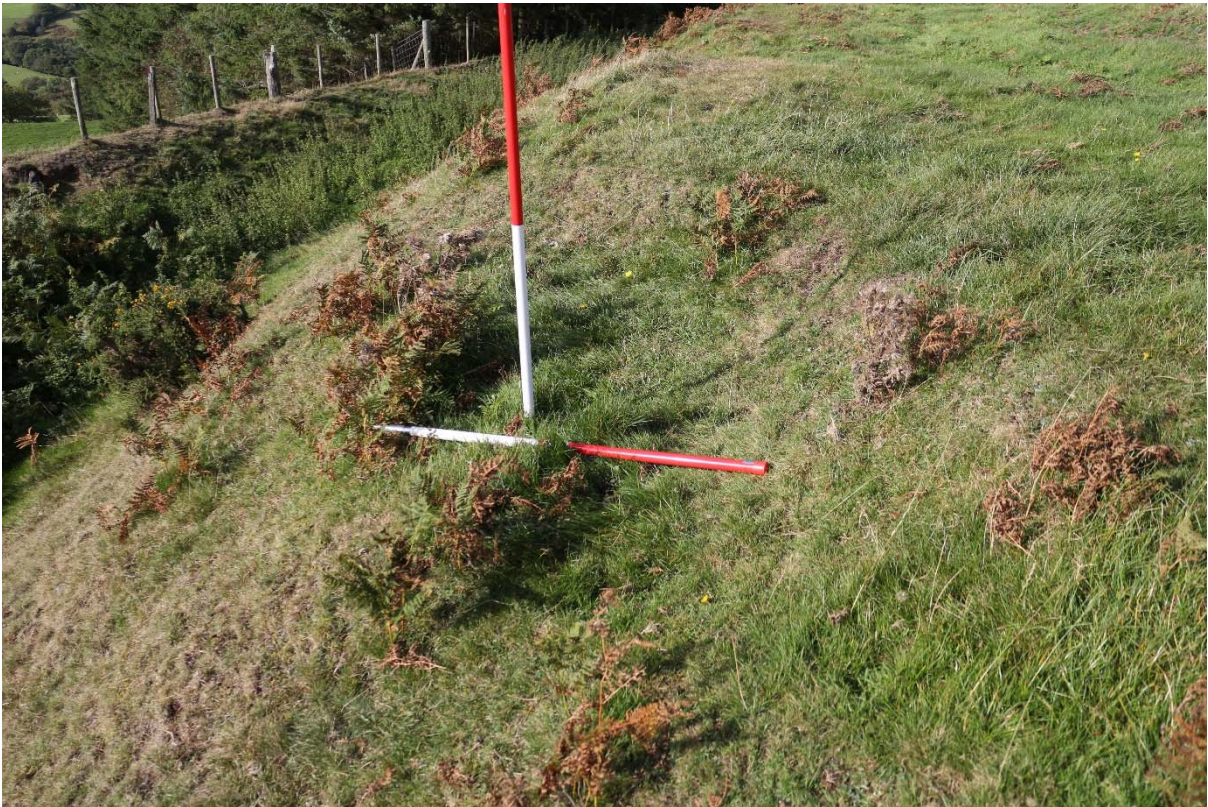
Locations 4, 5 & 6, before repair, IMG_2470, 02.10.2014
