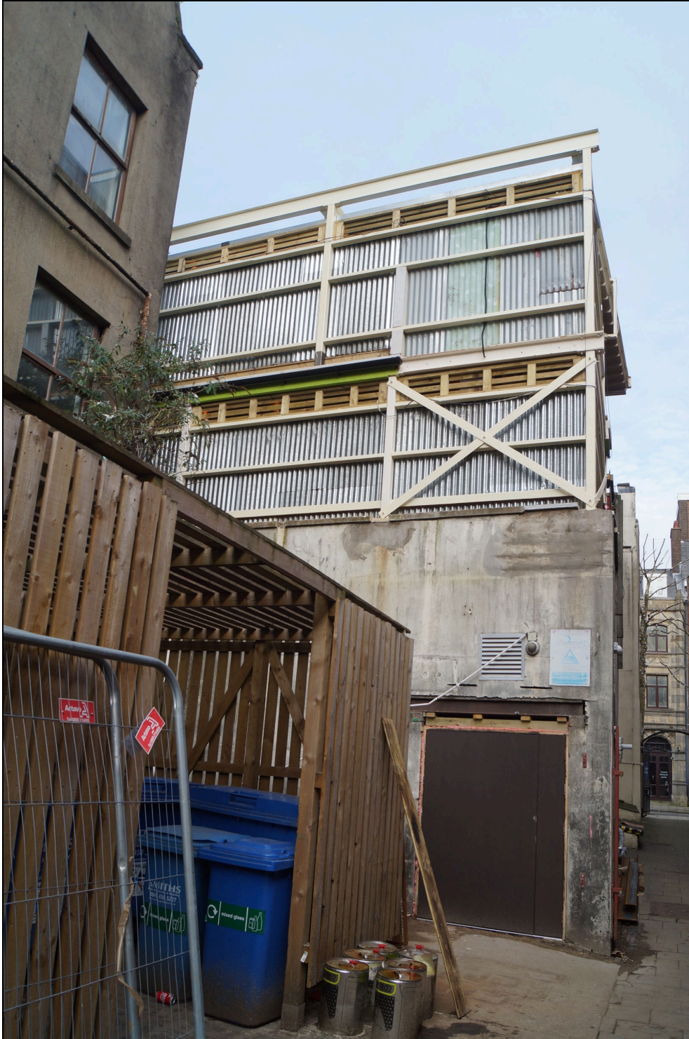
Plate 5: A view of the rear of the property showing the back of the new canopy over the mezzanine floor, rising above the southern end of the post-1999 extension to the former bank building. Looking north-northwest.
