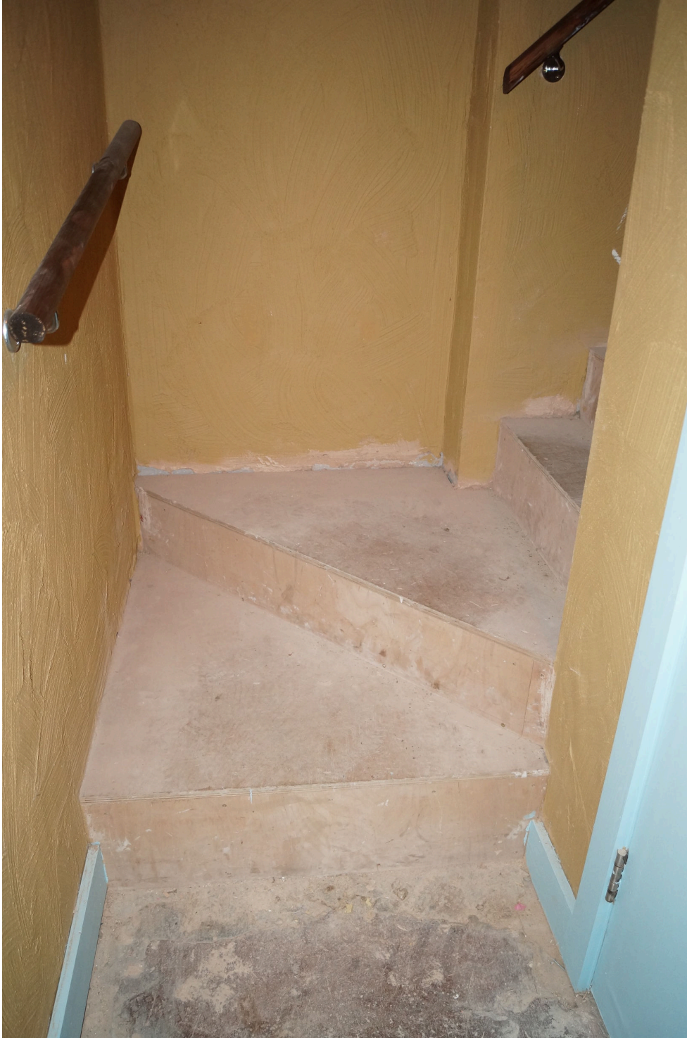
Plate 13: A view of the bottom of the stairwell, fire escape leading from the first to second floors, labelled B on Figure 11. New steps have been installed above the original steps to create broader steps and a less steep stairway for safety purposes. The original steps are hidden but undamaged. Looking south-southeast.
