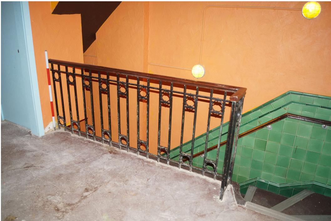
Plate 11: A view of the balustrade at the top of the stairs which lead from the ground floor entrance, No 51, on the eastern side of the building to the first floor offices. Looking east.
