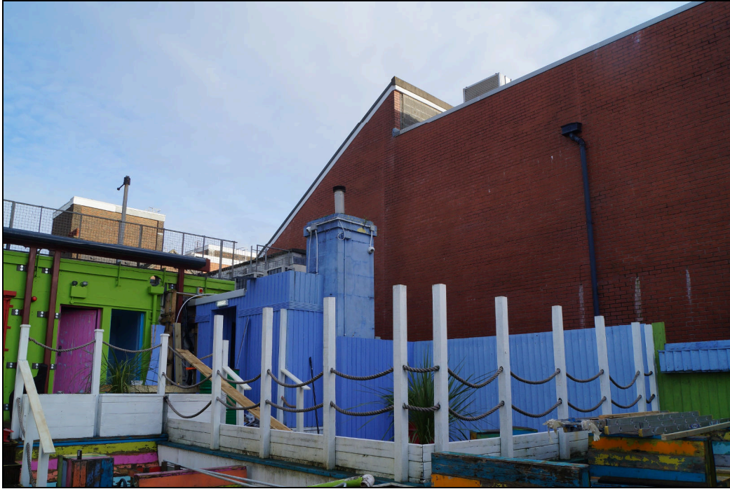
Plate 8: A view of the existing roof terrace. The rear wall of the original bank building is painted green. Note the large late 20 th century building to the east which blocks views in and out of the site. Looking northeast.
