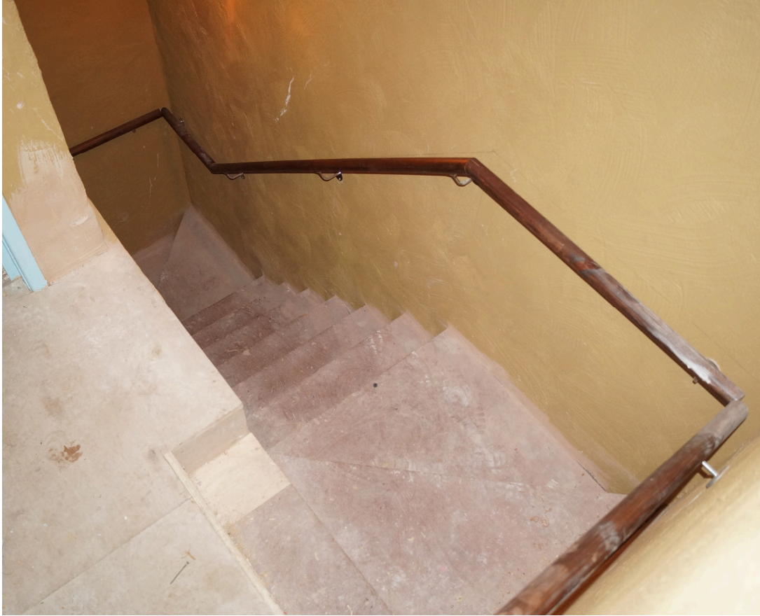
Plate 14: A view of the top of the stairwell/fire escape between the first and second floors, labelled B on Figure 12. New steps have been installed above the original steps to create broader steps and a less steep stairway for safety purposes. The original steps are hidden but undamaged. Looking northeast.
