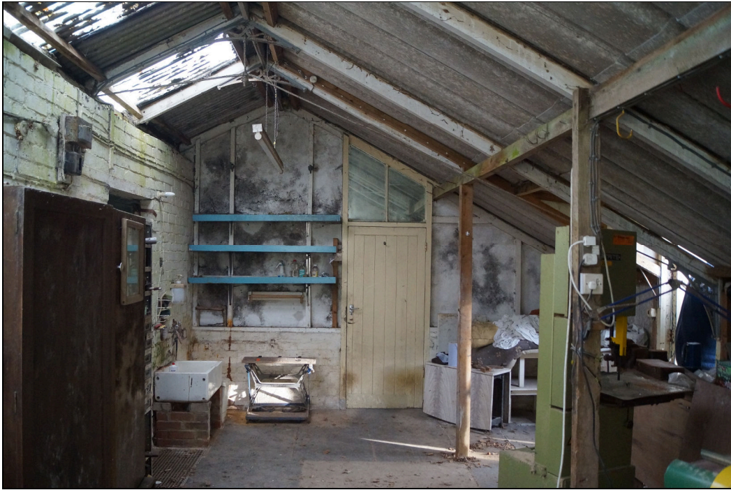
Plate 14: GGN2019_014 – A view inside the western part of the building. Note the original stone slabs around the side of the room and a concrete slab in the centre. The concrete may infill a former water tank or soil bed associated with the original use of the building as a glasshouse. Looking east.
