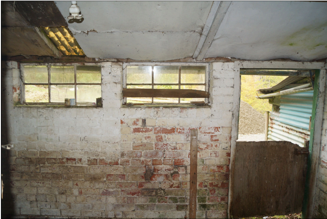
Plate 11: GGN2019_011 – A view of the northern lateral wall of the "stable". The metal-framed windows and brick walling appear to be original elements in the Edwardian potting shed. There is a later extension visible through the door to the right. Looking north.
