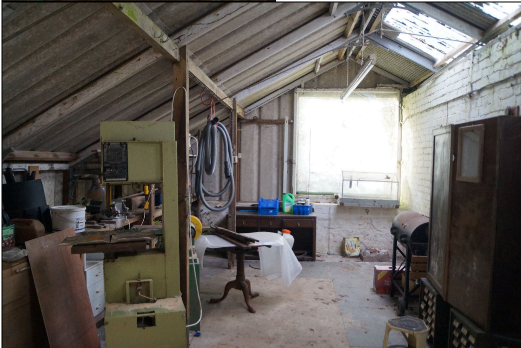
Plate 13: GGN2019_013 – A view inside the western part of the building. Note the original stone slabs around the side of the room and a concrete slab in the centre. The concrete may infill a former water tank or soil bed associated with the original use of the building as a glasshouse. Looking west.
