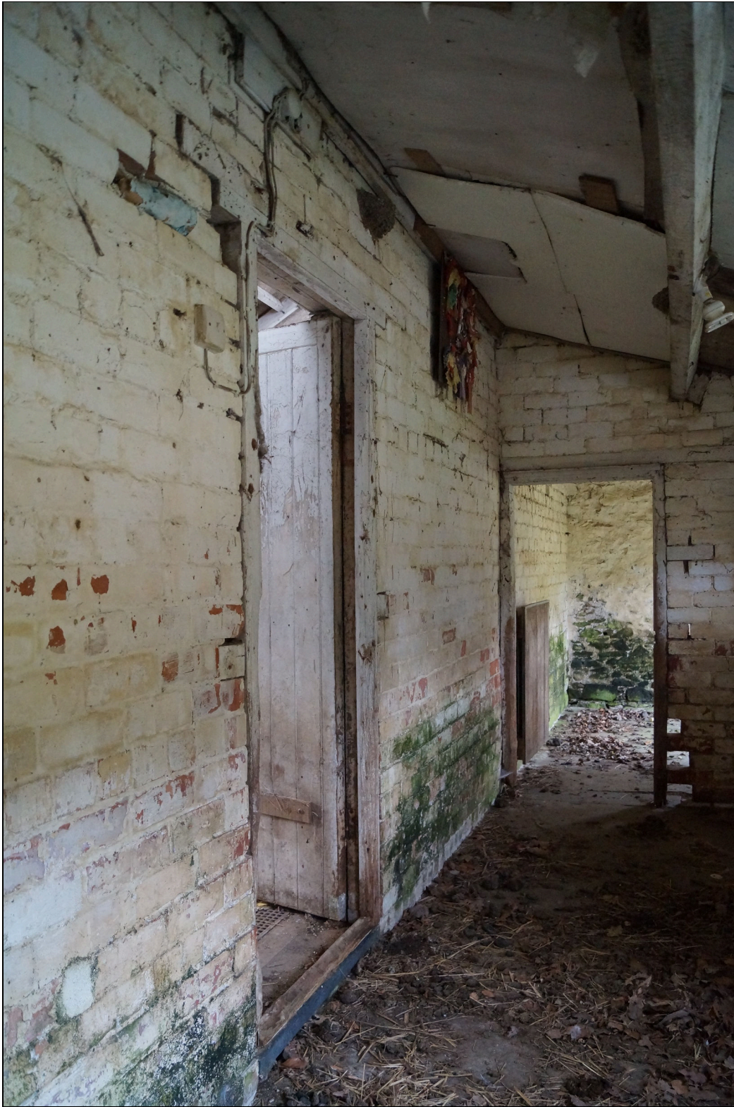
Plate 10: GGN2019_010 – A view inside the "stable" showing the door into the former glasshouse, left of centre. Original drain covers seem to be in place in the floor inside the door. Looking west-southwest.
