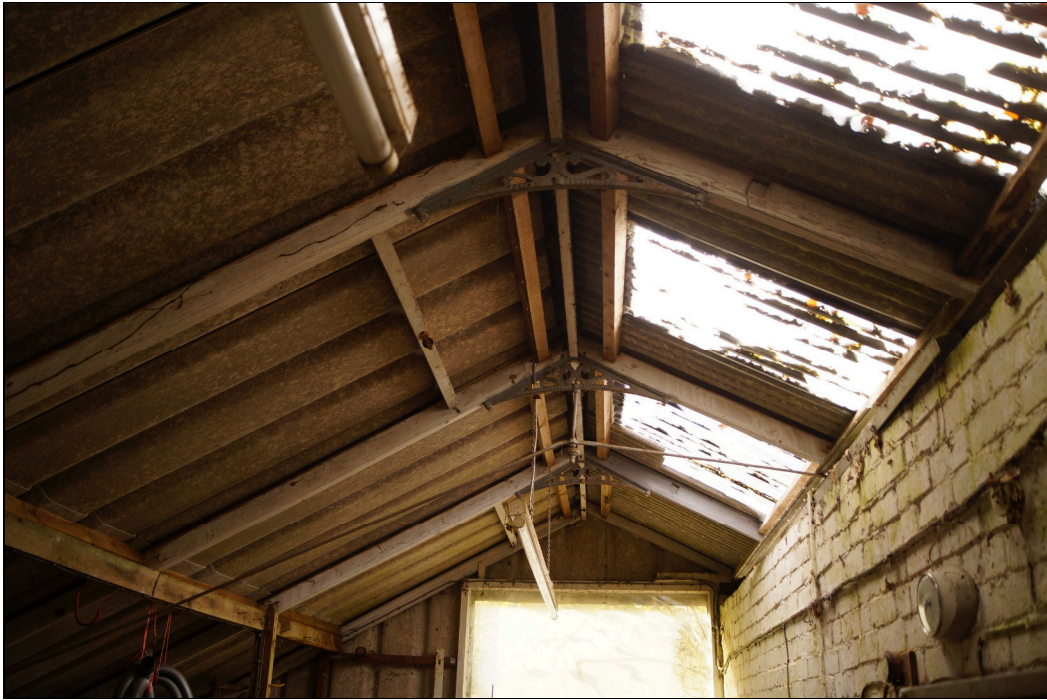
Plate 5: GGN2019_005 – A view of the roof and metal brackets in the western part of the building. Looking west.
