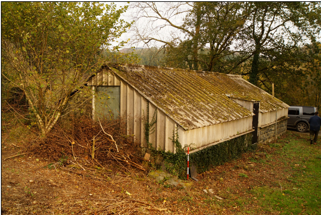
Plate 15: GGN2019_015 – An external view of the building. The corrugated asbestos sheeting seems to have replaced the original glass roof and walls over the front (south) side of the building. Looking northeast.
