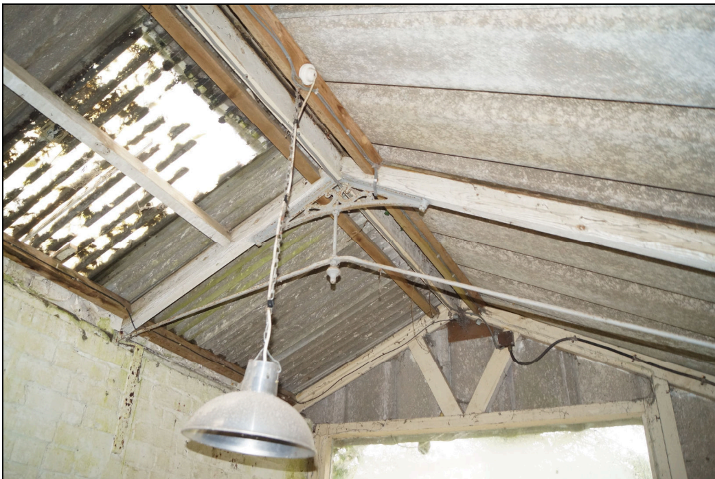
Plate 2: GGN2019_002 - A view of the metal brackets and struts at the apex of the roof in the workshop, which are original and form the roof structure of the glasshouse. Looking east-northeast.
