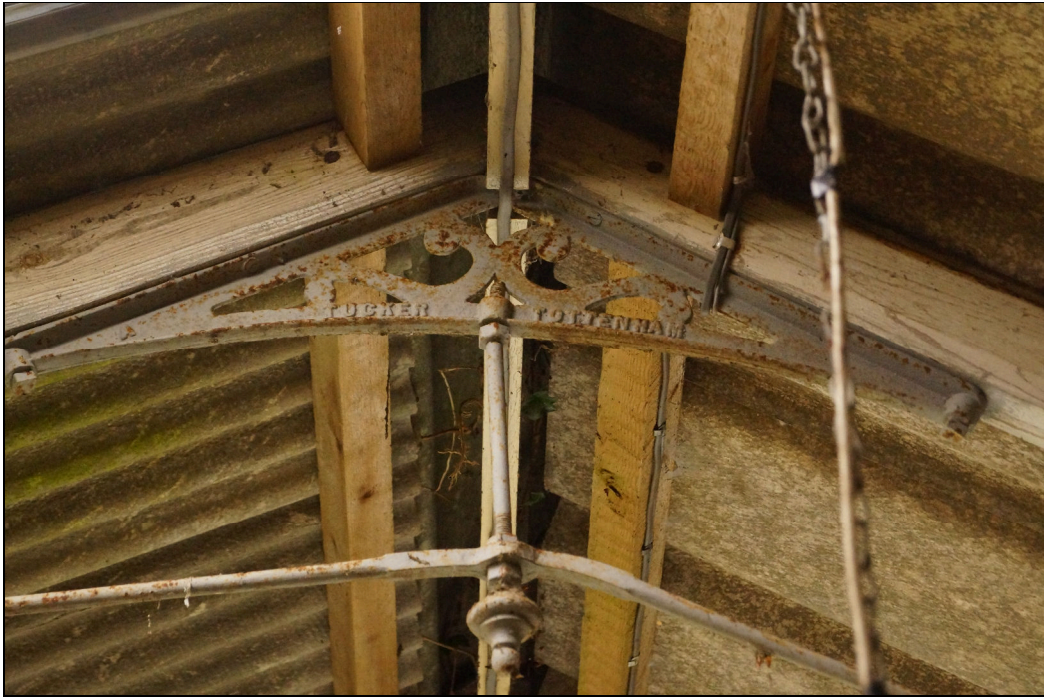
Plate 3: GGN2019_003 – A closer view of the roof brackets in the workshop showing the “Tucker Tottenham” stamp of the specialist glasshouse manufacturer who designed and supplied the structure. Looking east.
