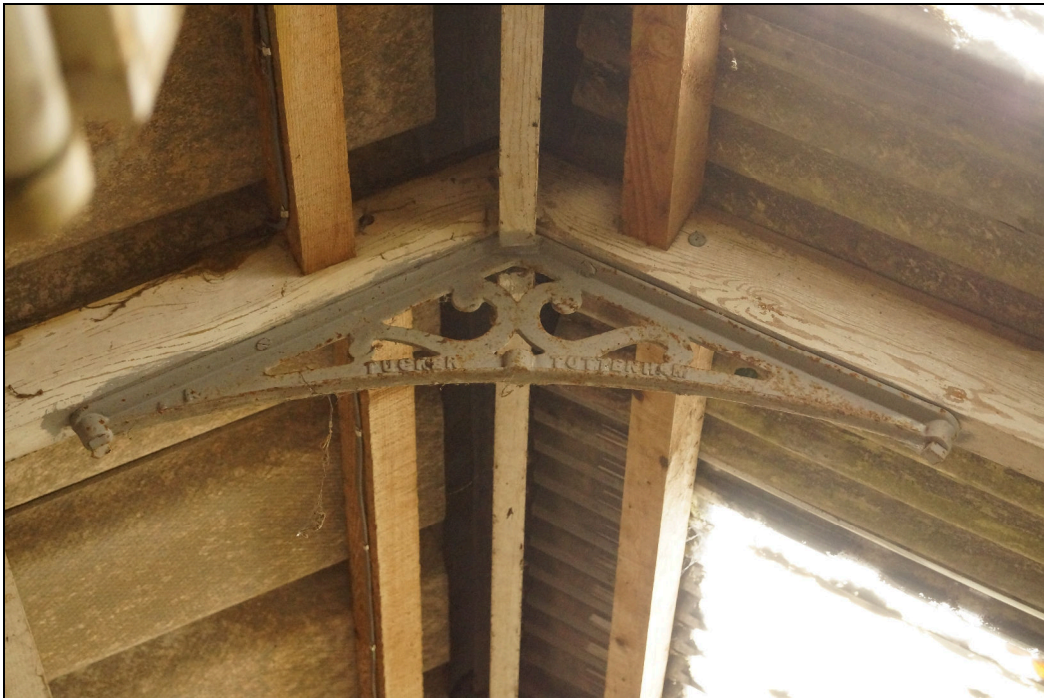
Plate 4: GGN2019_004 – A view of the roof brackets in the western part of the building showing the manufacturers stamp. Looking west.
