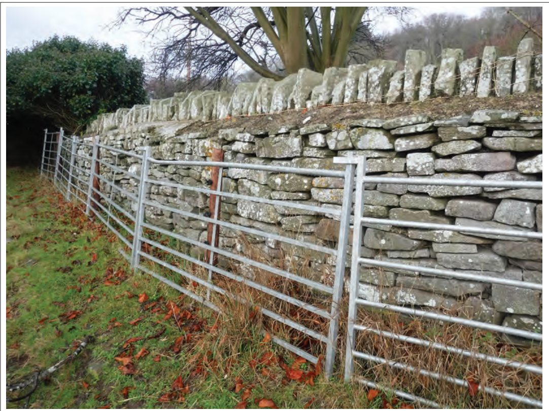
Plate 6. Drystone wall bounding the driveway to the north of the proposed development area, looking north-west.
