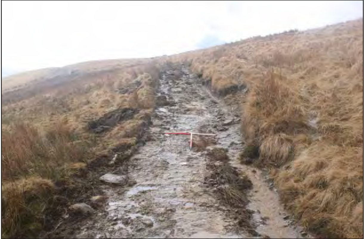
Plate 23 View south-west of area 3a after removal of large central high standing rut (western area of scheme)
