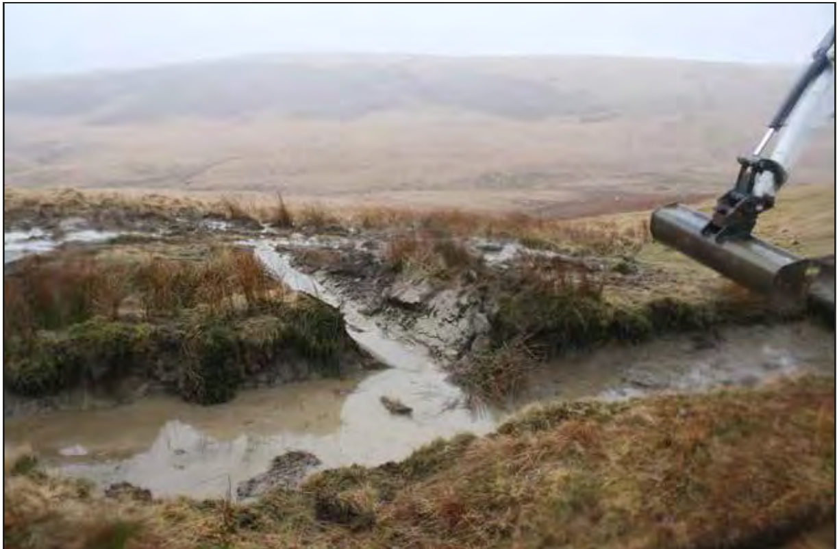
Plate 12 View south of drainage grip installed within area 8 (eastern area of scheme)
