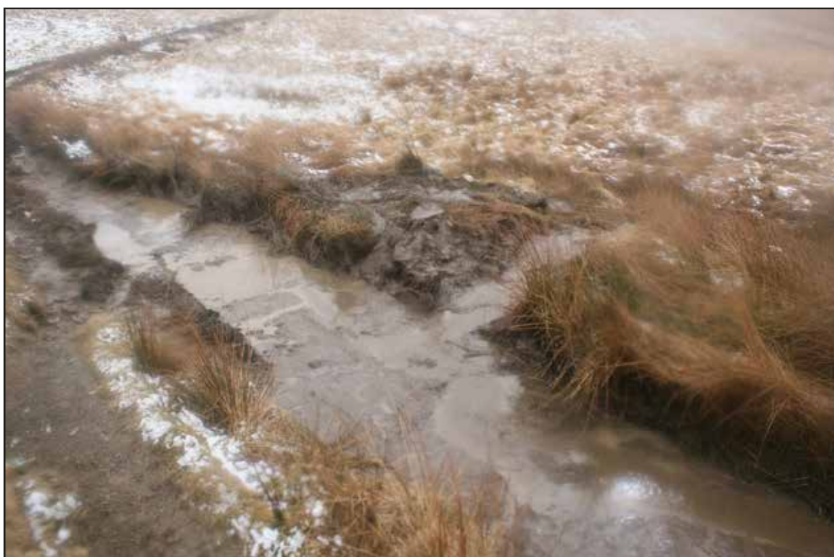
Plate 28 View south-east of drainage grip installed within area 7 (western area of scheme)
