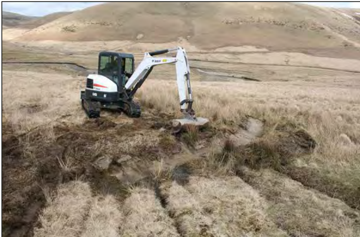
Plate 4 View east of drainage grip being installed within area 2 (eastern area of scheme)
