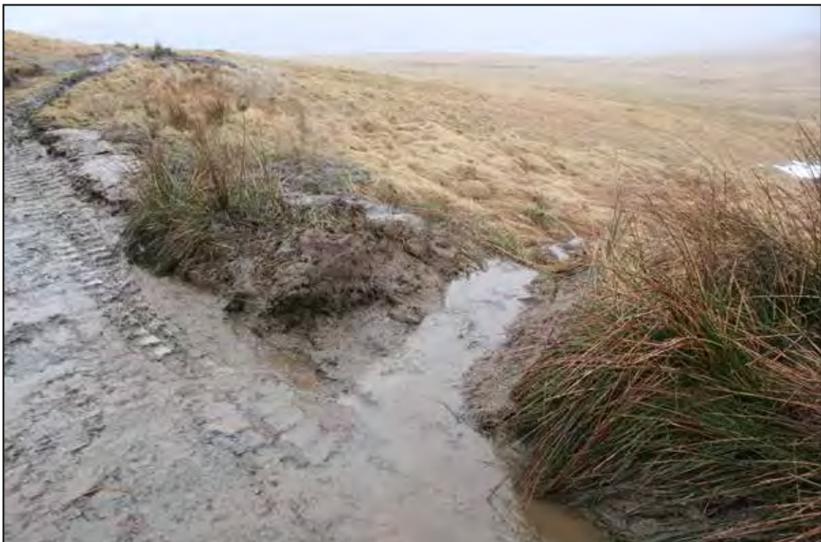
Plate 8 View south-east of drainage grip installed within area 4b (eastern area of scheme)
