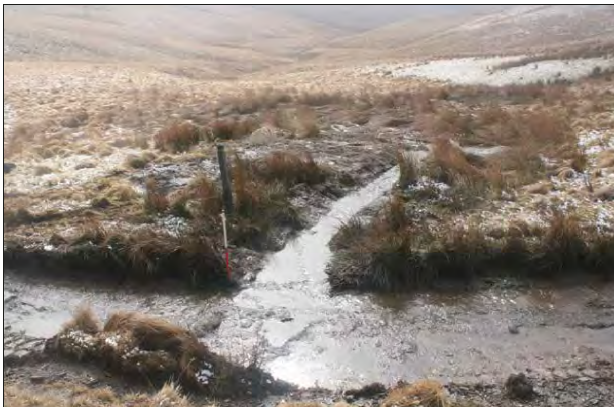
Plate 27 View south of drainage grip installed within area 6 (western area of scheme)
