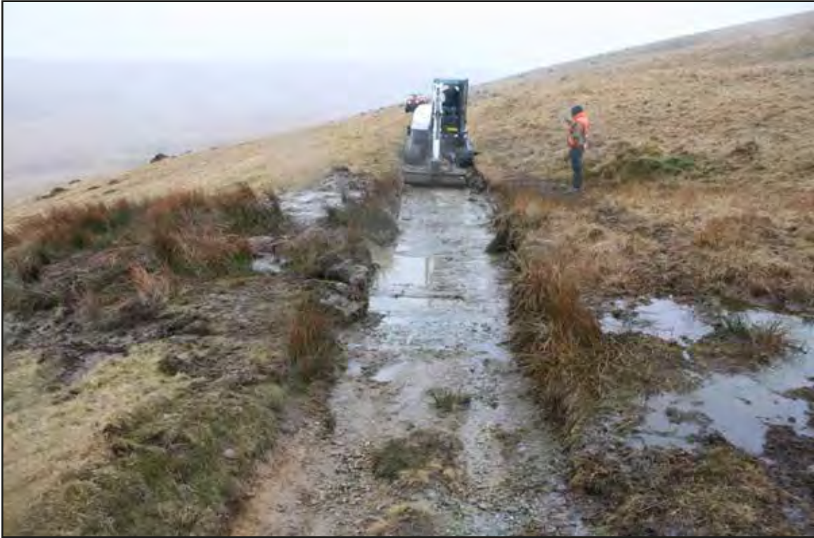
Plate 9 View west of drainage grip installed within area 5 (eastern area of scheme)
