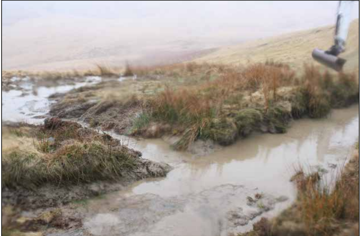
Plate 11 View south of drainage grip installed within area 7 (eastern area of scheme)
