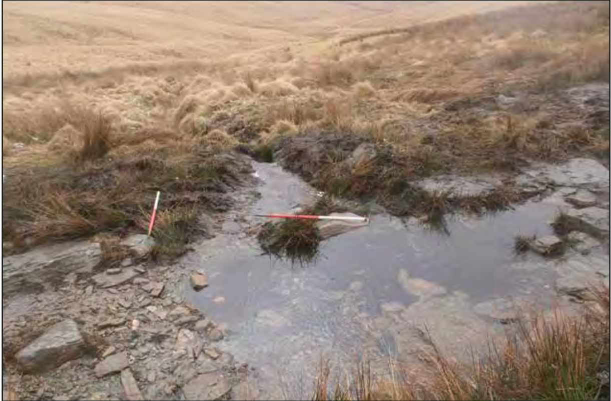
Plate 25 View south of small grip installed within area 5 (western area of scheme)
