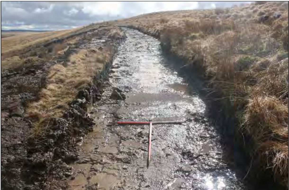
Plate 20 View south-west of re-grading works completed in area 1(western area of scheme)
