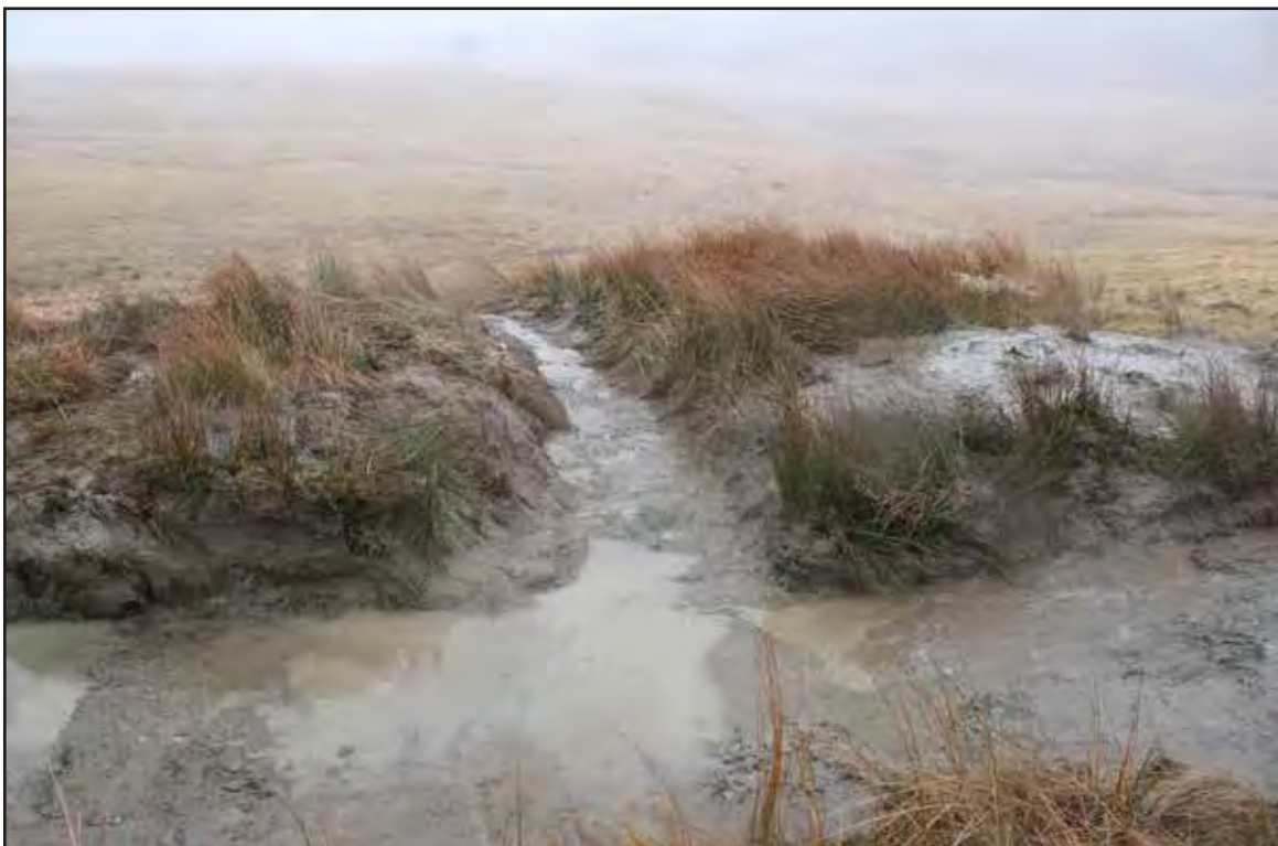
Plate 10 View south of drainage grip installed within area 6 (eastern area of scheme)
