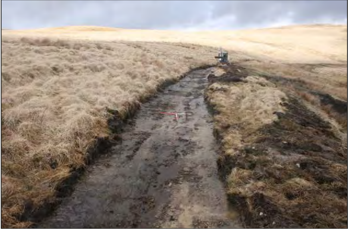
Plate 19 View north-east of re-grading works completed in area 1(western area of scheme)
