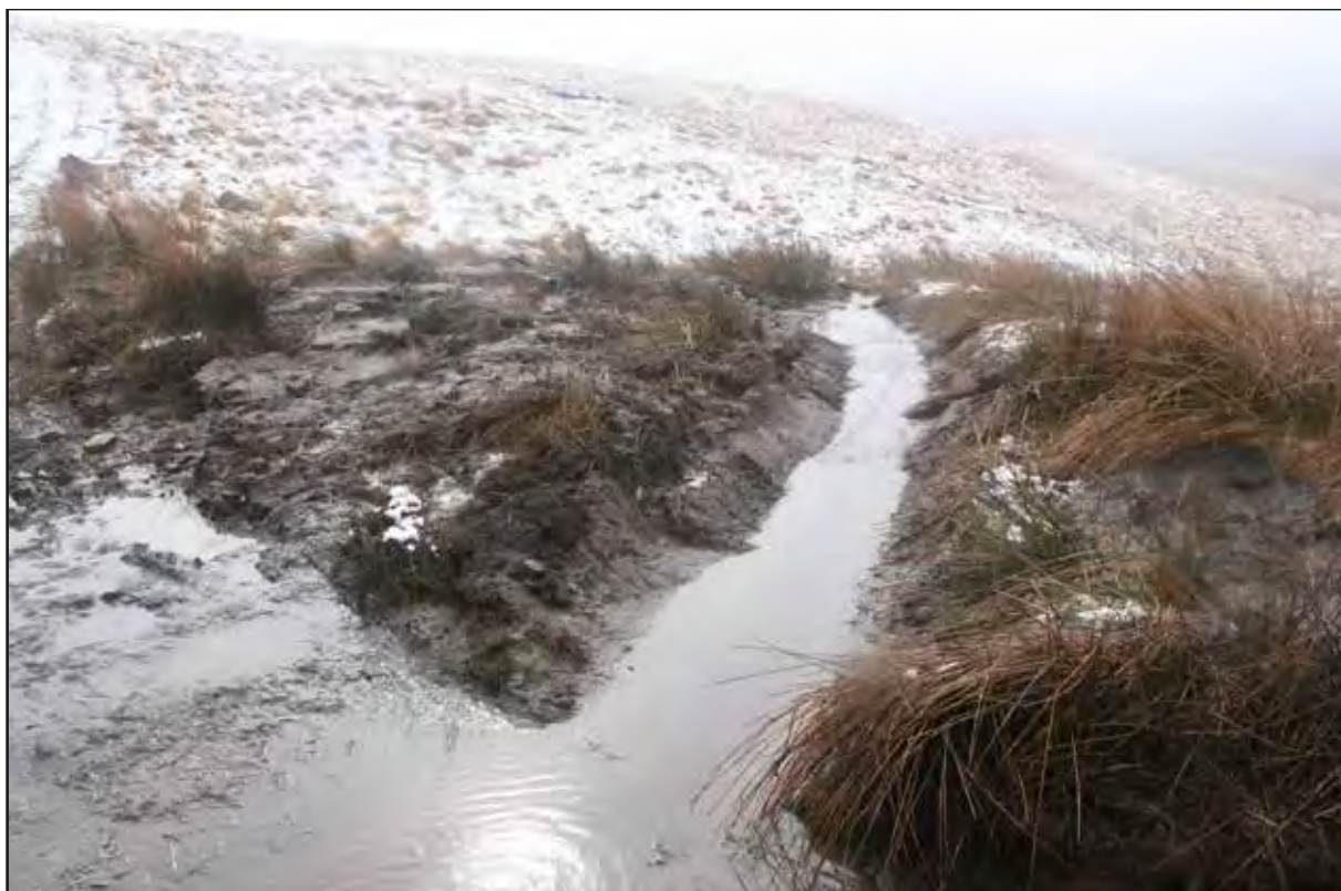
Plate 31 View south-west of drainage grip installed within area 8 (western area of scheme)
