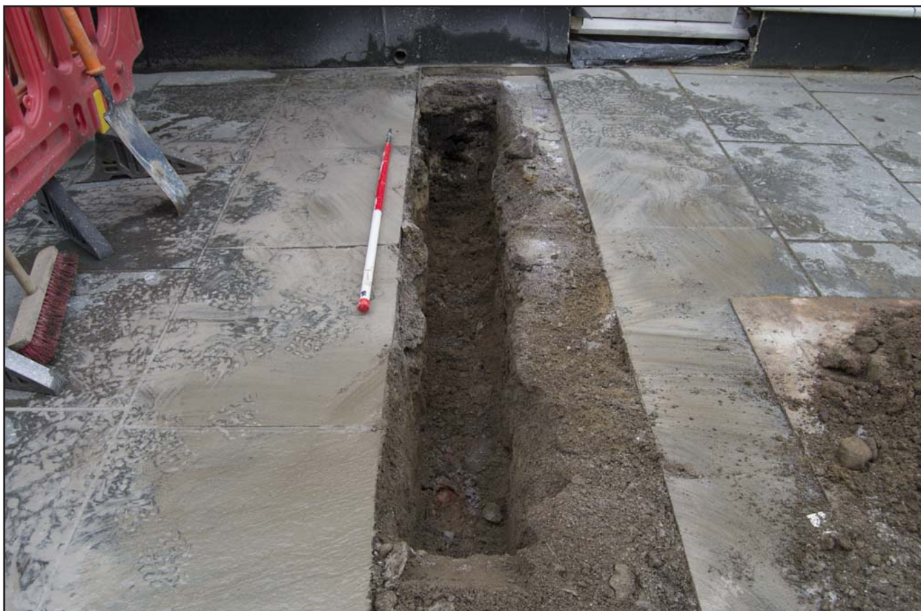
Plate 8: View of Trench A excavated to 450mm depth through pavement adjacent to Nos. 9 to 11 Castle Ditch - scale 1x1m; view from W (archive reference: G2775_17).
