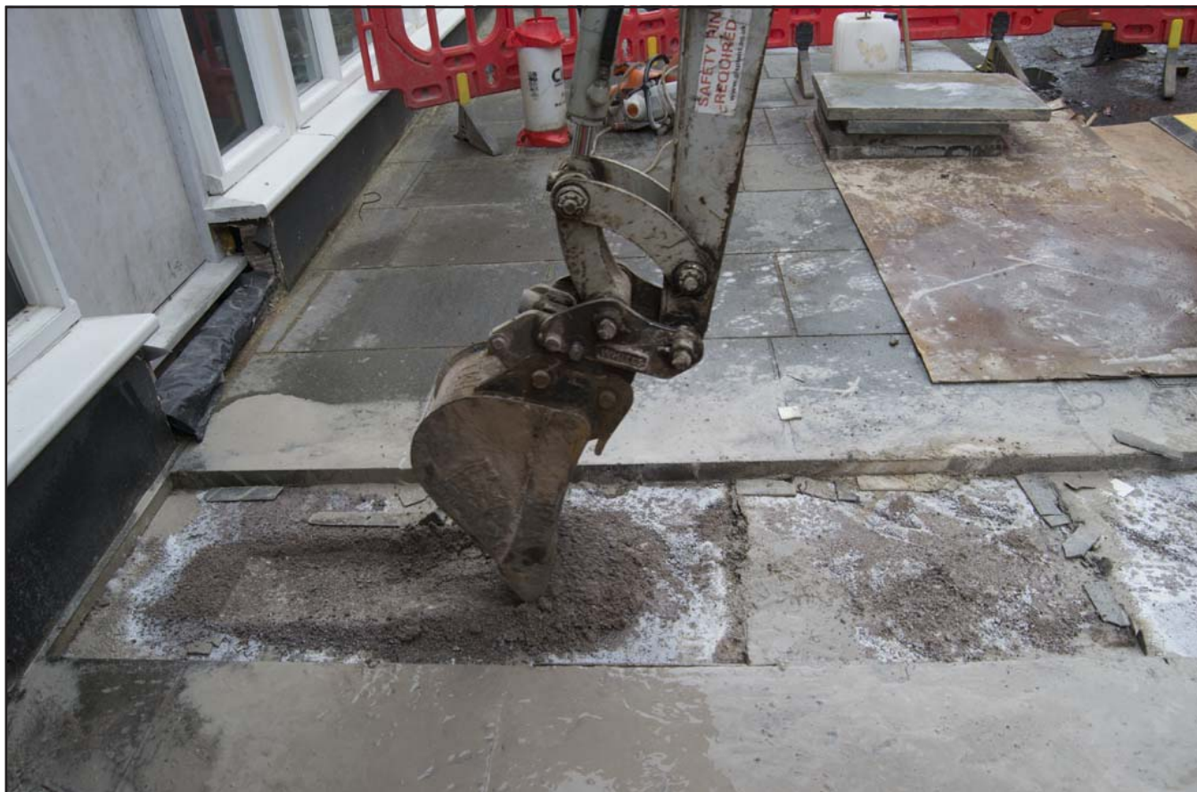
Plate 7: Working shot of excavation of made ground in Trench A using excavator - scale 1x1m; view from W (archive reference: G2775_15).
