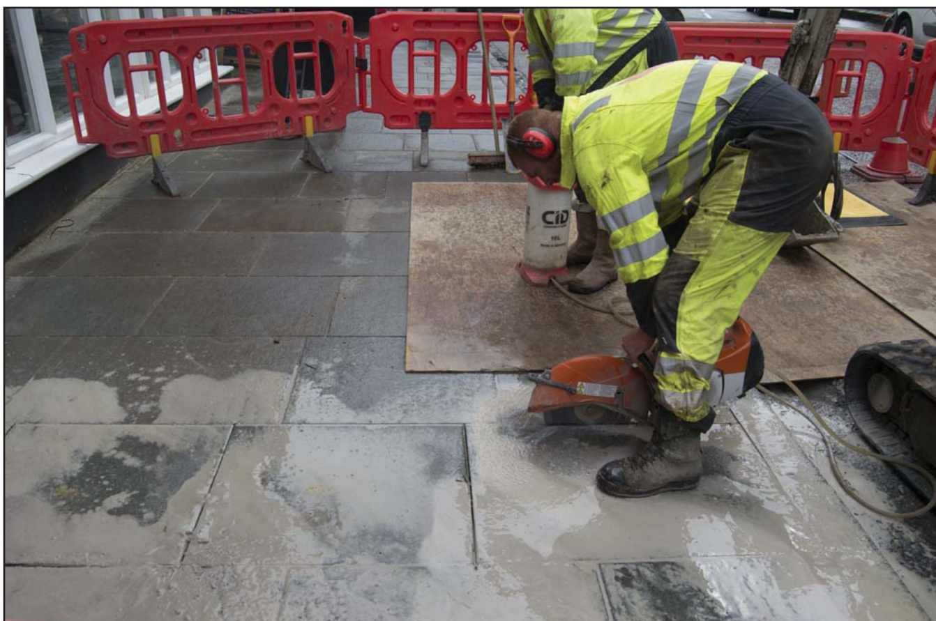
Plate 4: Working shot of work in progress showing cutting of concrete slabs in Trench A using a circular saw - scale not used; view from W (archive reference: G2775_08).
