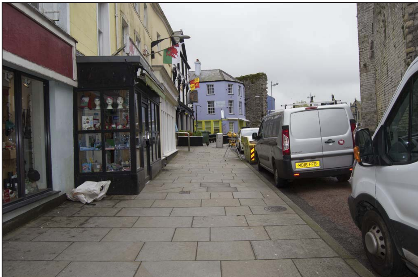
Plate 3: Pre-commencement view of groundworks for electrical cable connection to Nos. 9 to 11 Castle Ditch - scale not used; view from WSW (archive reference: G2775_04).
