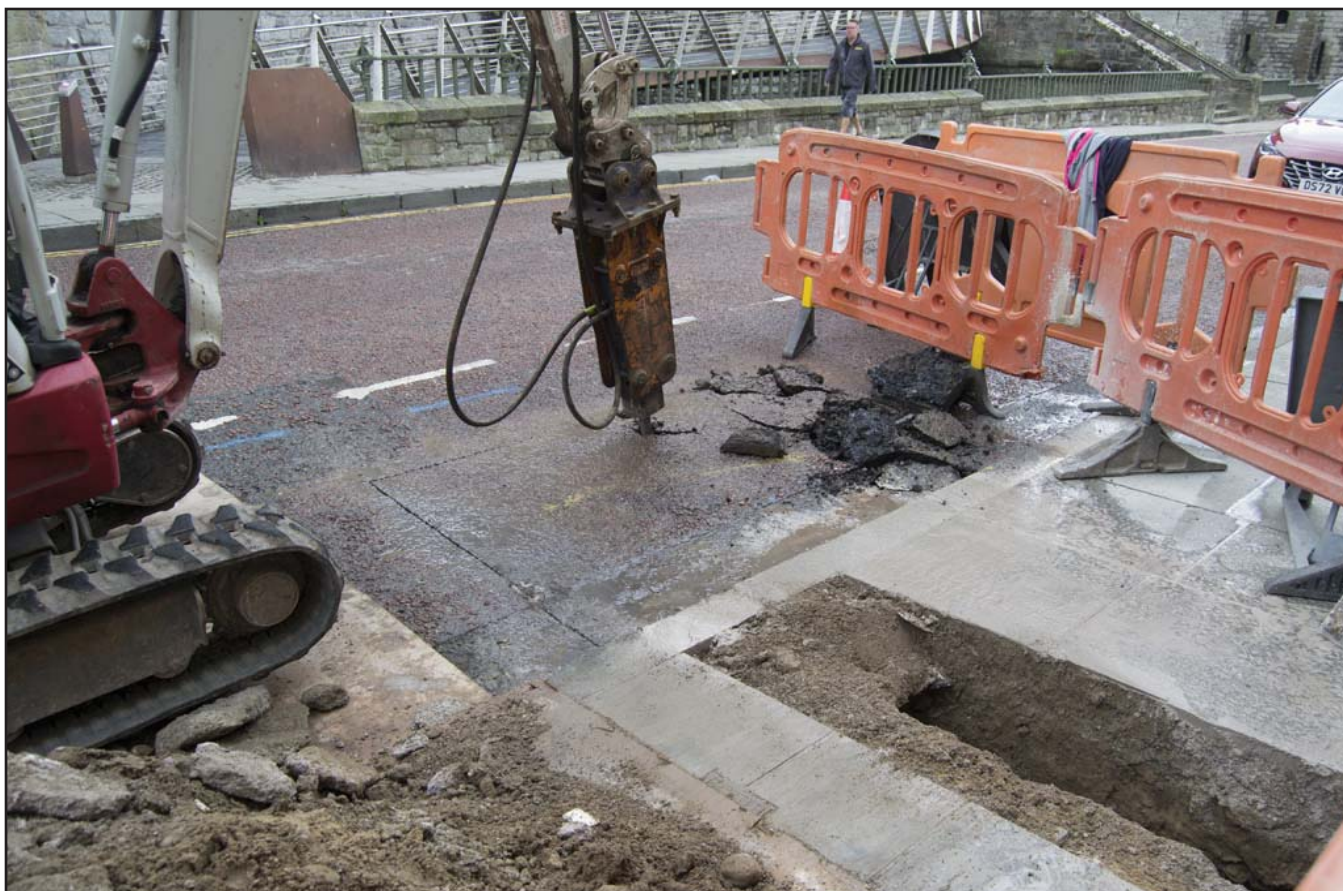
Plate 10: Working shot of road surface broken down by machine as part of Trench B route - scale not used; view from ENE (archive reference: G2775_22).
