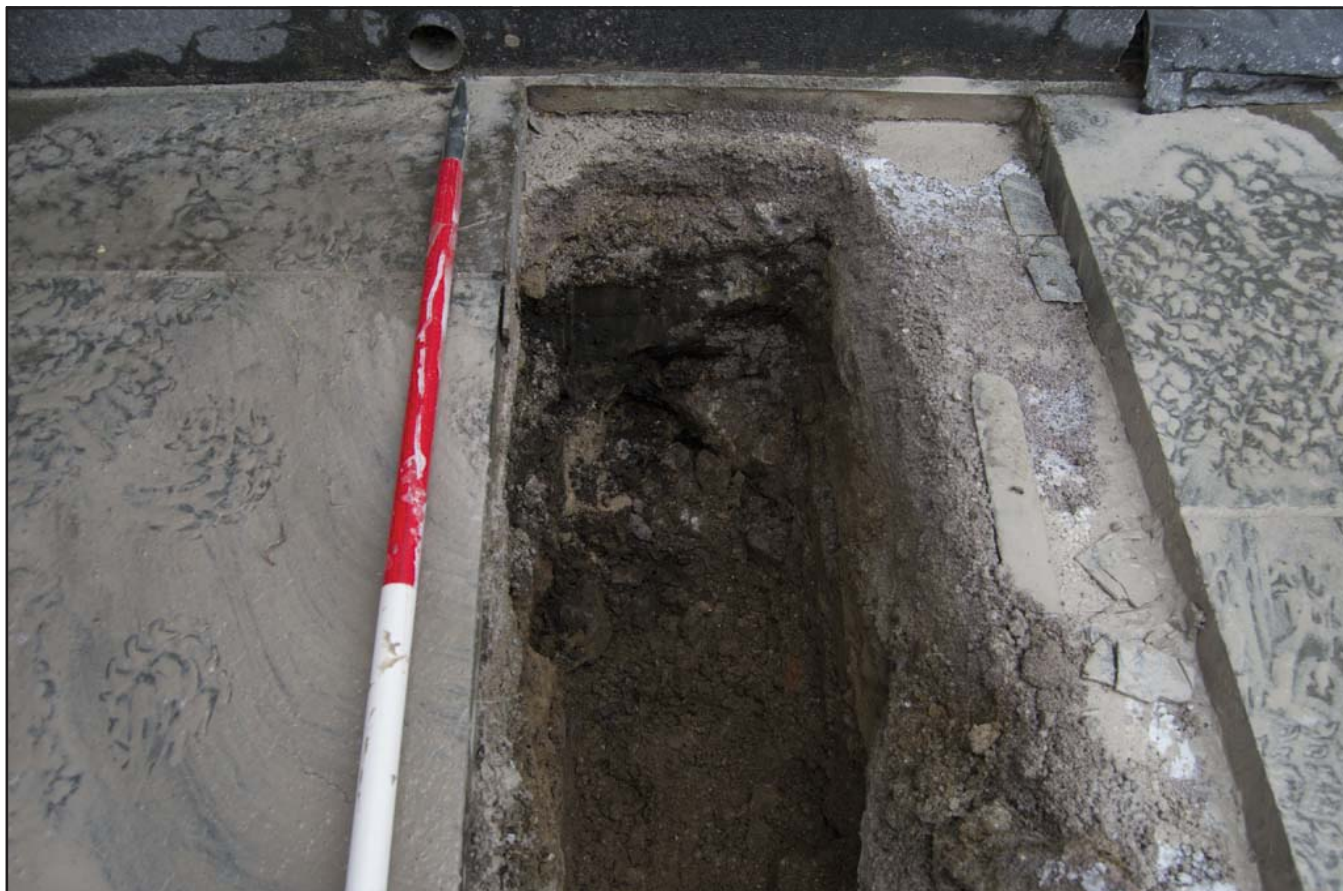
Plate 9: Close up view of south facing section showing foundation of Nos. 9 to 11 Castle Ditch - scale 1x1m; view from W (archive reference: G2775_18).
