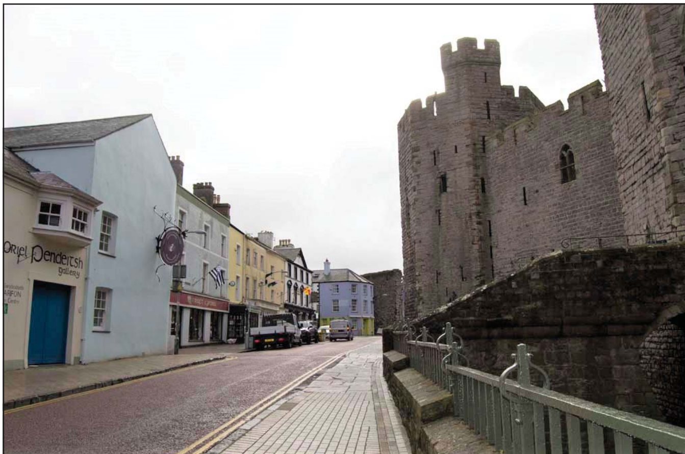
Plate 1: Pre-commencement view of groundworks for electrical cable connection to Nos. 9 to 11 Castle Ditch - scale not used; view from WSW (archive reference: G2775_01).
