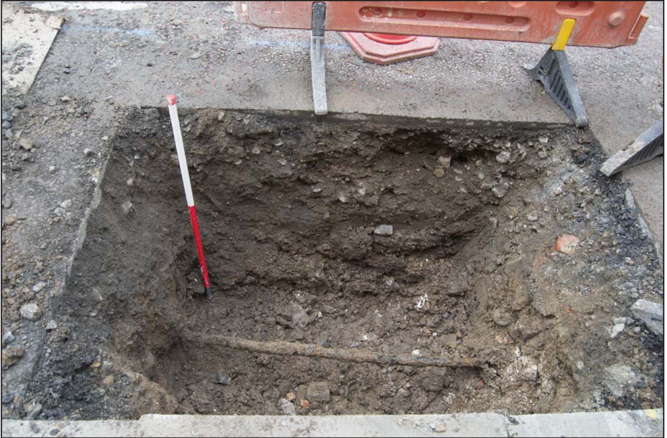
Plate 11: North facing section of Trench B excavated to 1.10m depth, showing existing electric main - scale 1x1m; view from N (archive reference: G2775_26).
