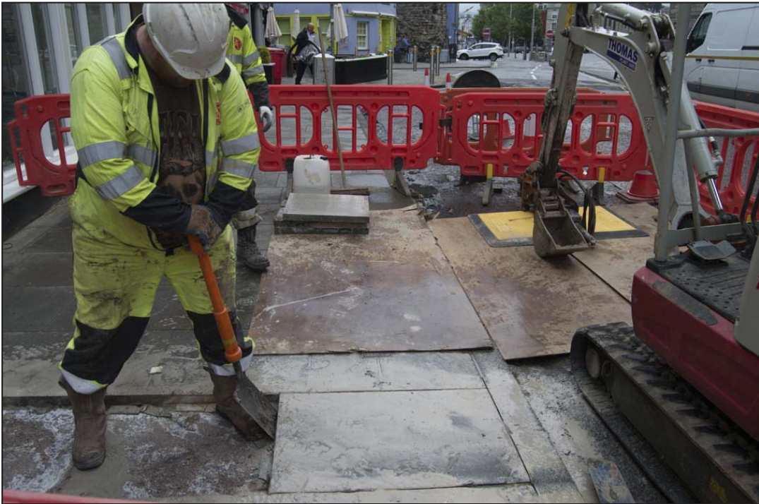
Plate 5: View of removal of concrete pavement slabs in Trench A by shovel and hand - scale not used; view from W (archive reference: G2775_10).
