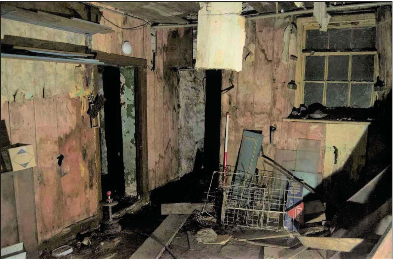
Plate 12: View of room with blocked up window - scale 1x1m; view from NW (archive reference: G2775_29).
