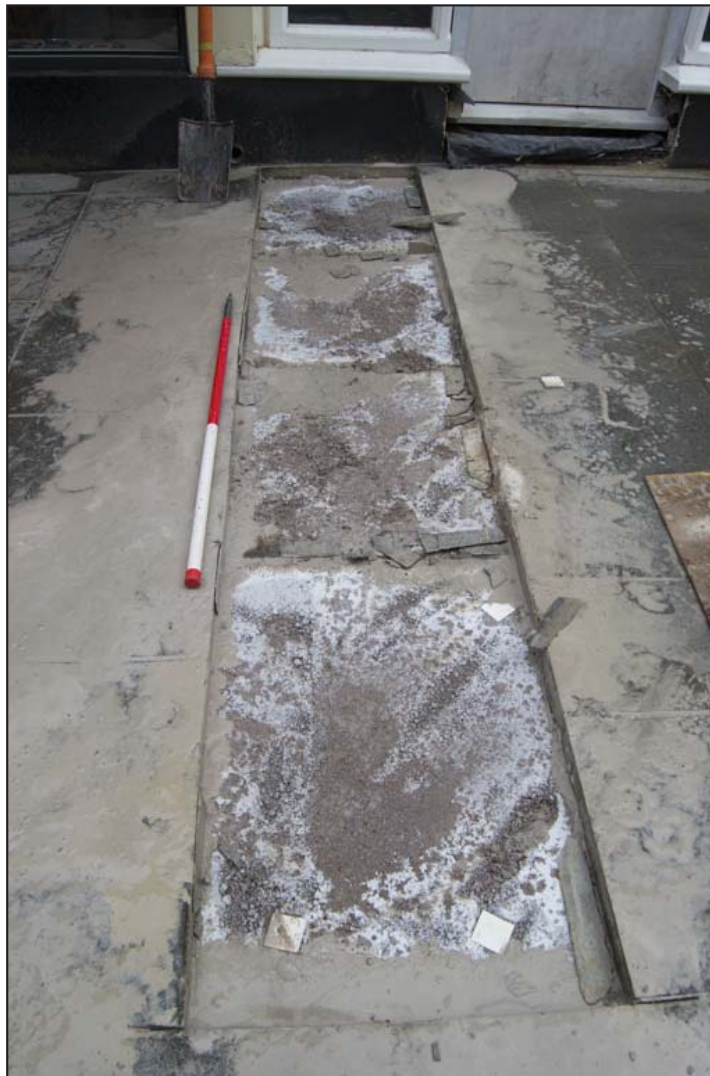
Plate 6: View of made ground beneath concrete slabs in Trench A - scale 1x1m; view from S (archive reference: G2775_13).
