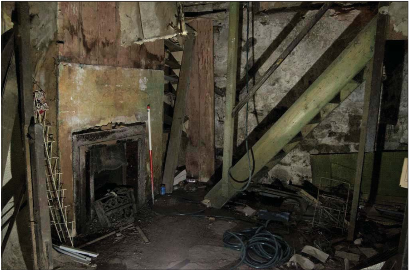
Plate 13: View of room with blocked up window showing steps and original fireplace - scale 1x1m; view from SE (archive reference: G2775_30).
