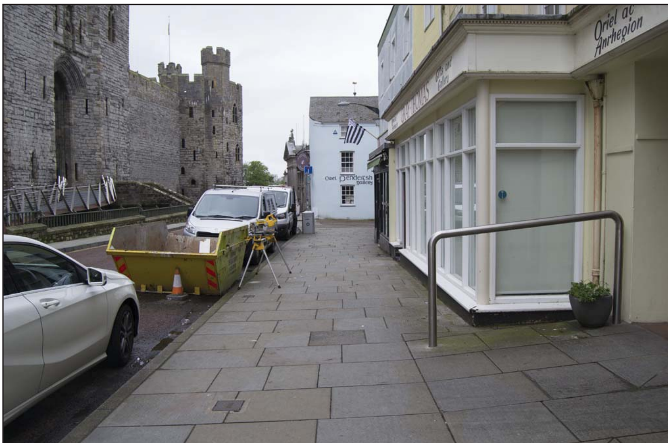
Plate 2: Pre-commencement view of groundworks for electrical cable connection to Nos. 9 to 11 Castle Ditch - scale not used; view from ENE (archive reference: G2775_03).
