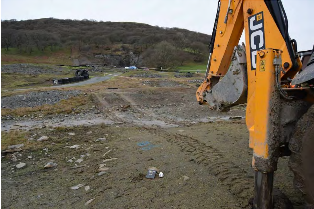
Photo 3: General shot of excavations in the centre of the site. Facing north.
