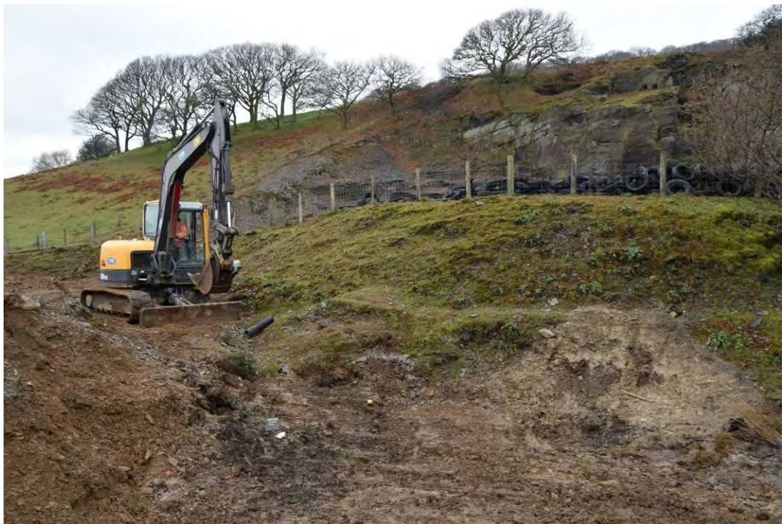
Photo 2: General shot of excavations at the northern end of the site. Facing northwest.
