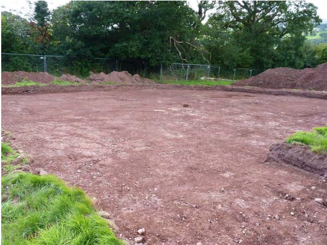
Photo 3: General shot looking east across the excavated area. Slwch Lane lies behind the treeline to the rear.
