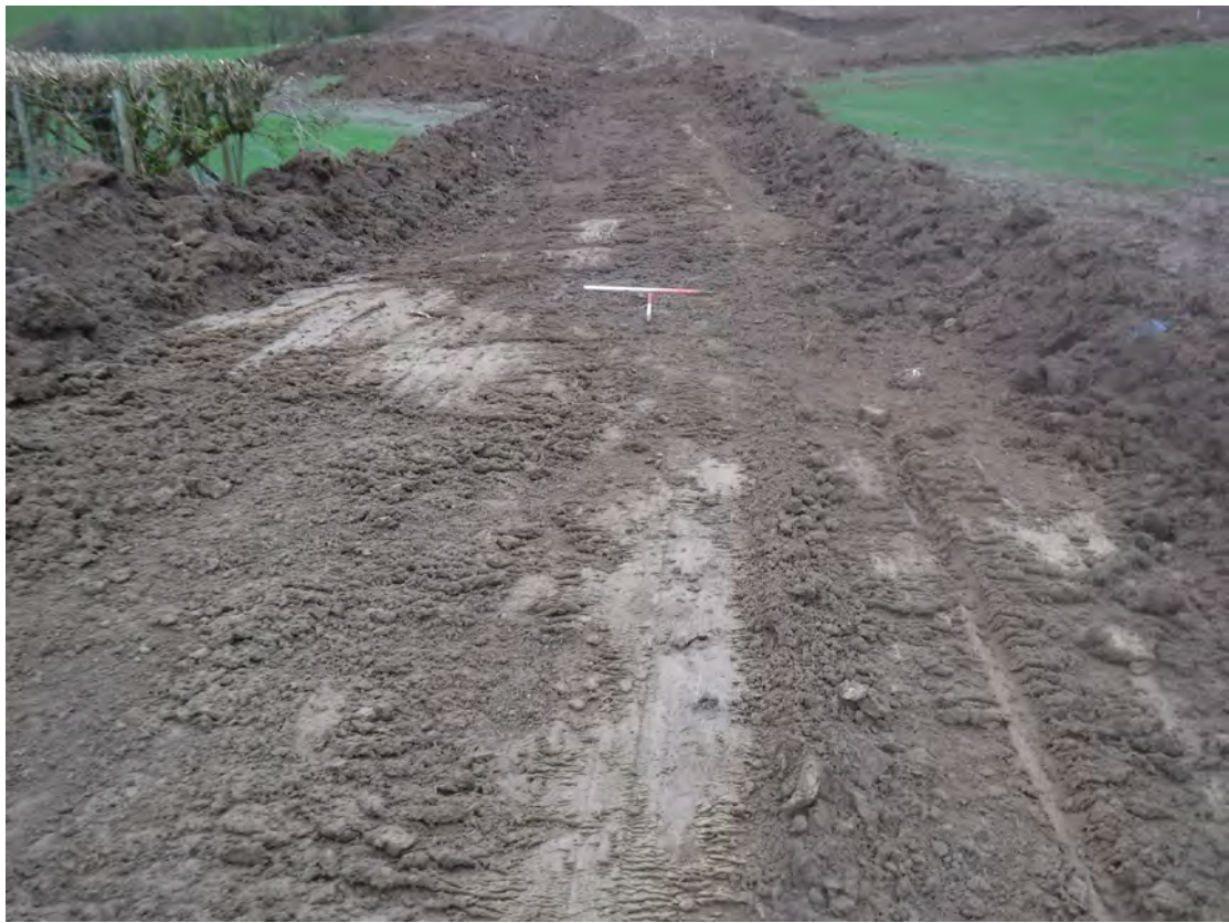
Plate 9. Topsoil (2001) stripped for new haul road within Area B. Scales 2 x 1m
