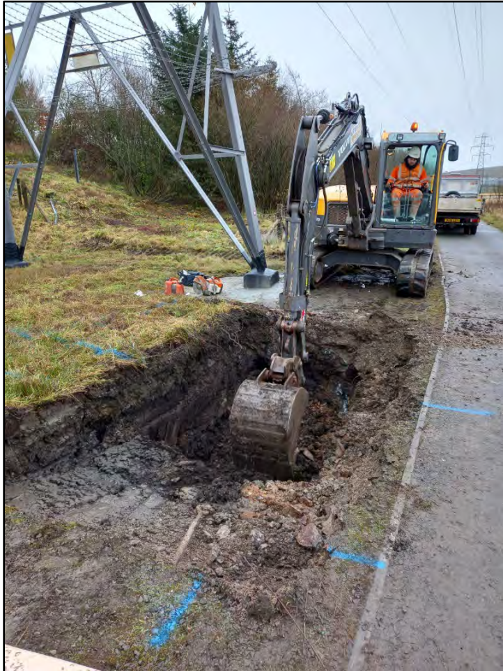
Plate 7 : DD3A Test Pit 1 SW of existing pylon, Working Shot, View to E
