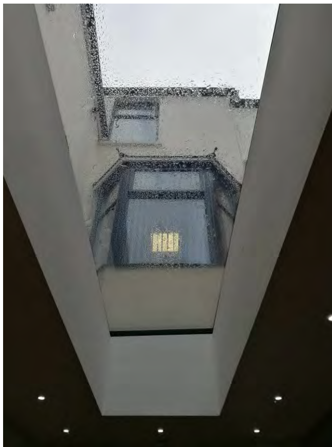
Photo 12: View from within current single-storey extension, looking up through the roof light at the original rear wall of No.19. This will be retained.
