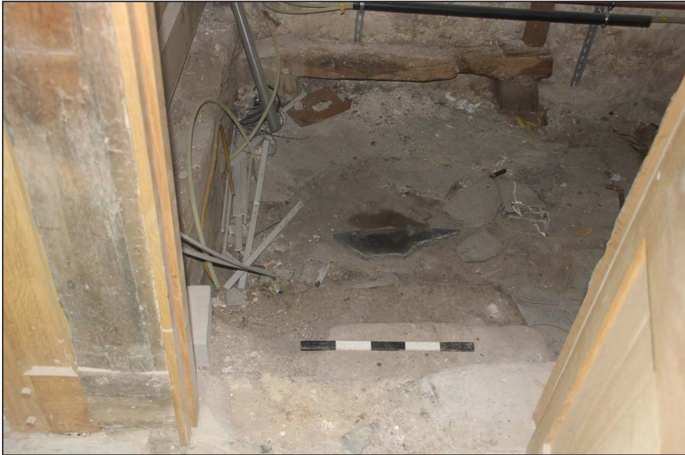
Plate 30: Revealed stone steps in well of stair, from the west. Scale 0.5m.
