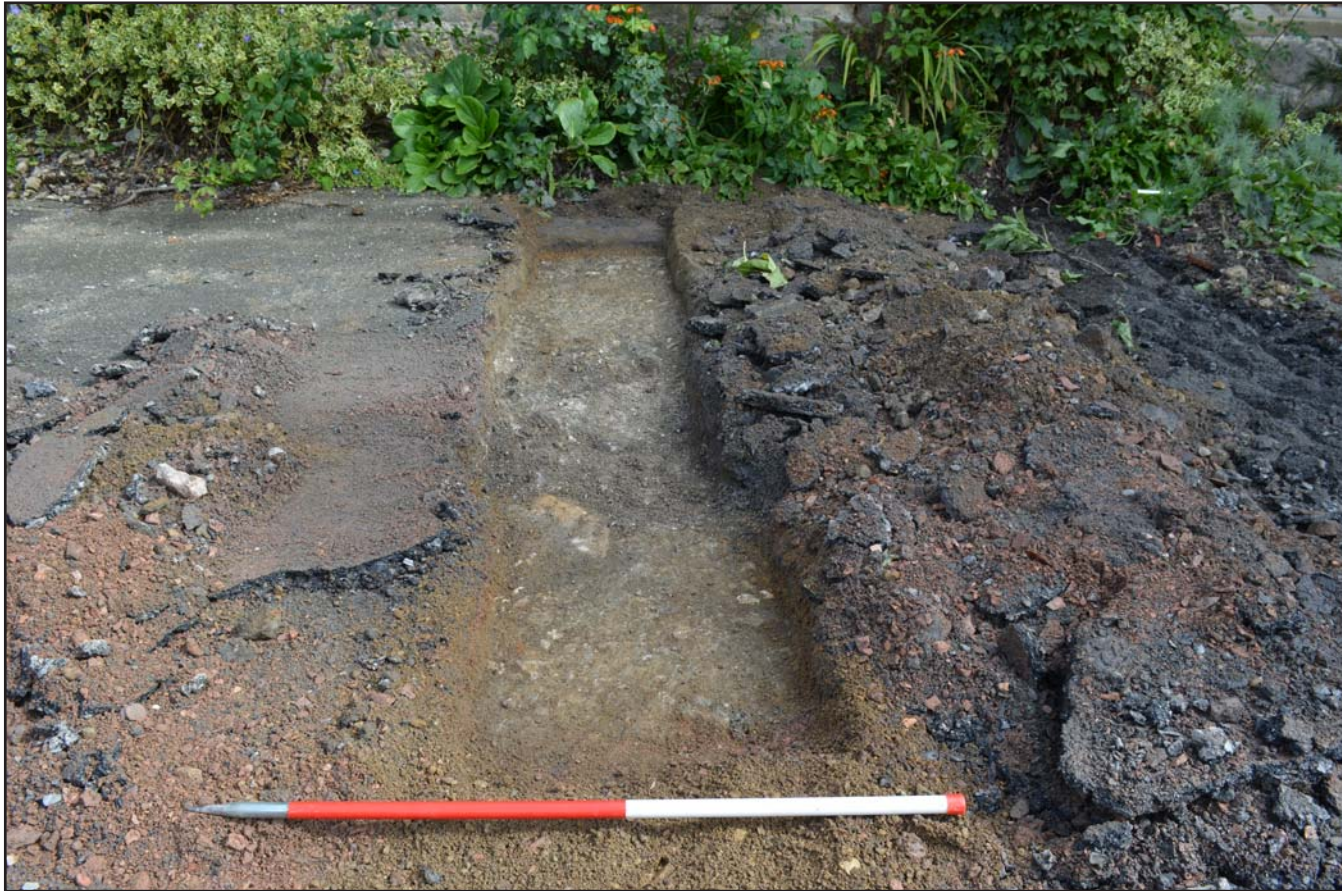
Plate 06: Drainage connection C1 showing relict surface deposit (06) and cut of drain [07], from the southwest. Scale 1.0m.
