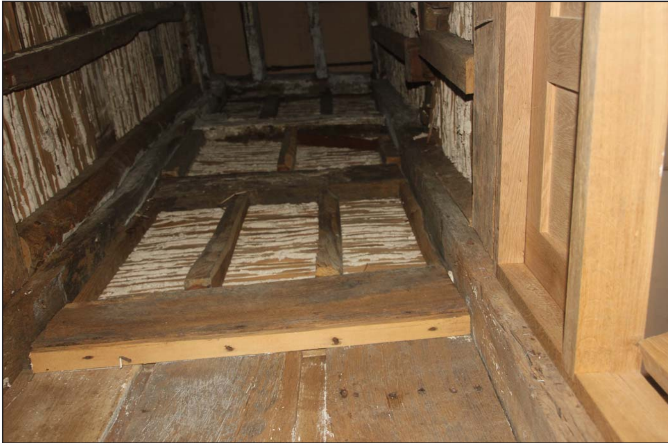
Plate 29: Revealed timber framing and wattle and daub walls in well of stair, from the northwest.
