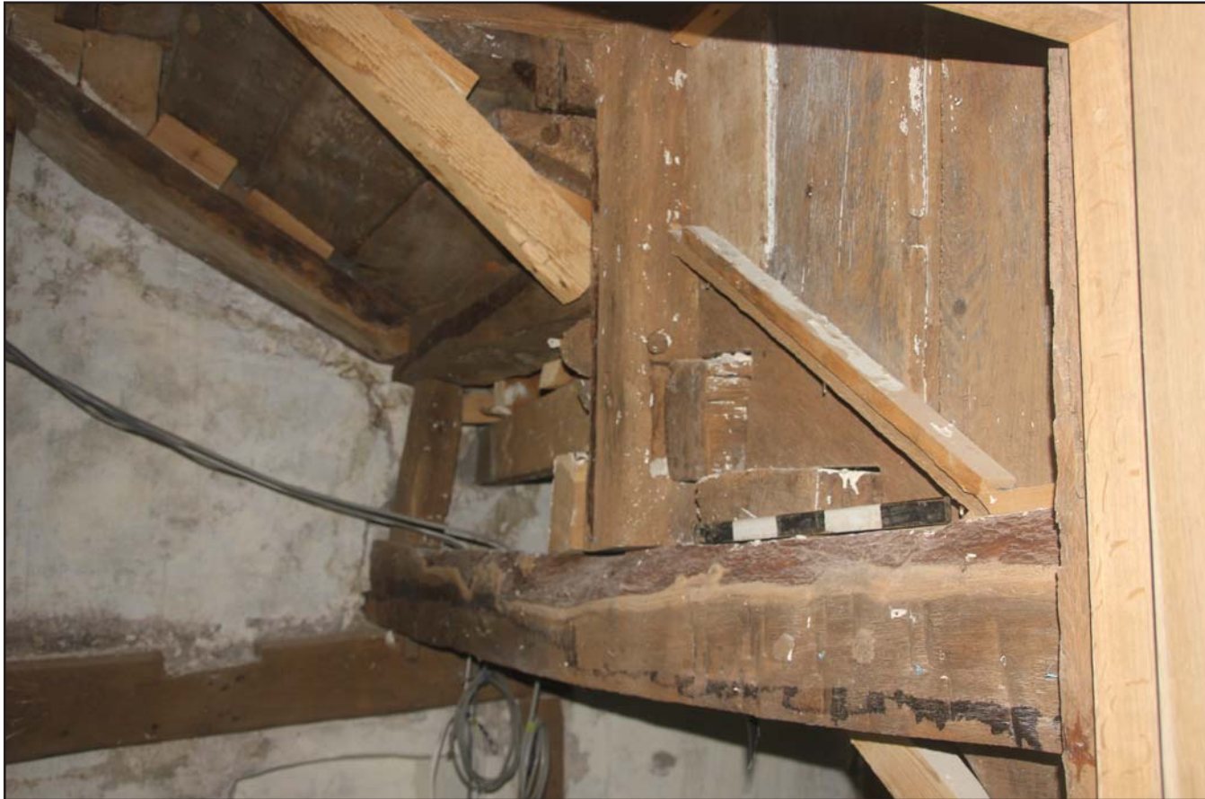
Plate 28: Revealed timber framing in well of stair, from the west. Scale 0.5m.
