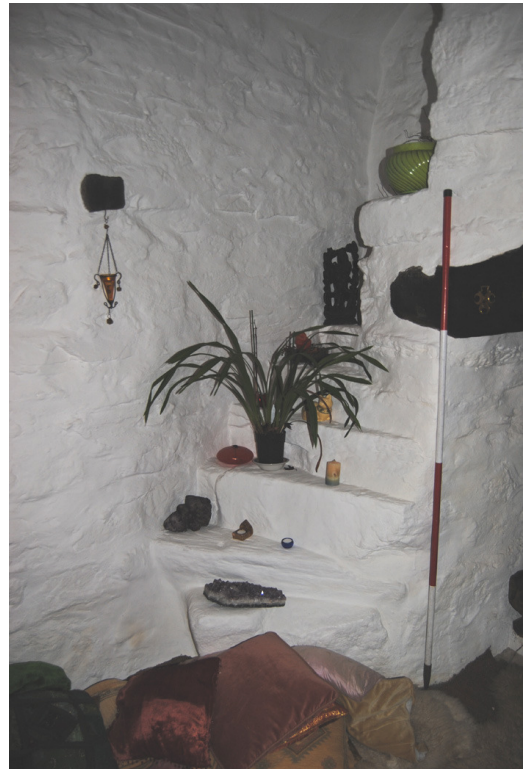
Plate 35: Stone winder stair to north of FP; note cut off joist of former first floor.
