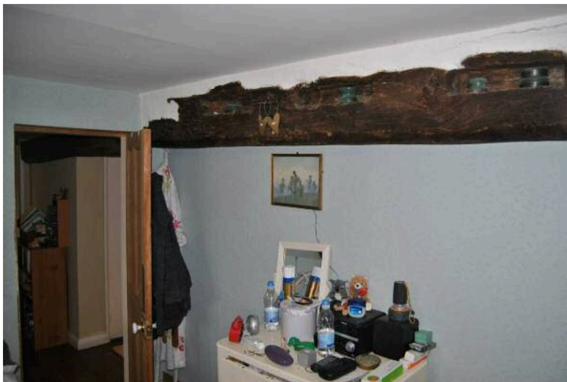
Plate 29: Sockets for 1ft wide ceiling joists in axial beam, exposed below raised ceiling within [F3].
