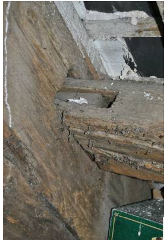
Plate 40: Detail of bridled scarf joint to threaded purlin. INB. purlin notched to respect principal
