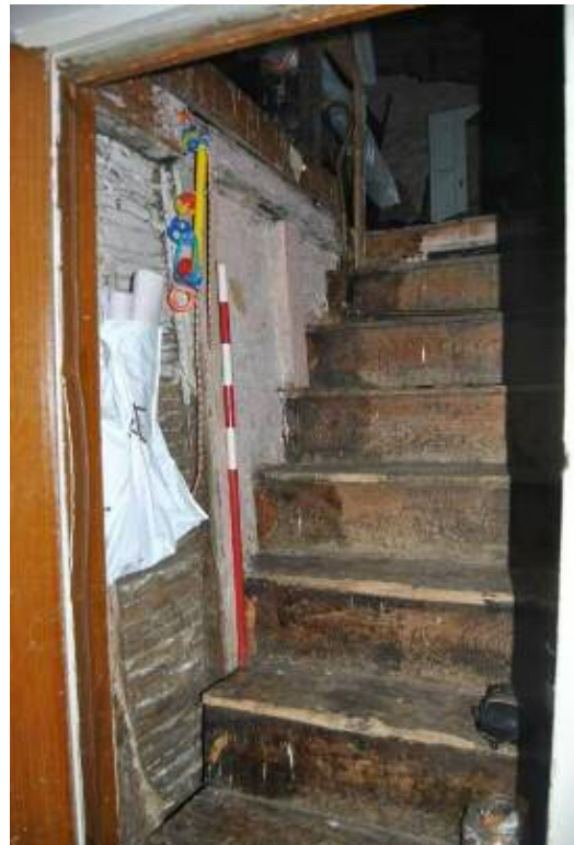
Plate 32: Enclosed, straight-flight stair rising to roof-space from landing [FB1].
