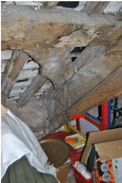
Plate 37: Multiple pegging of arch-brace to principal. NB. 2-part brace, jointed just above level of wall-head.
