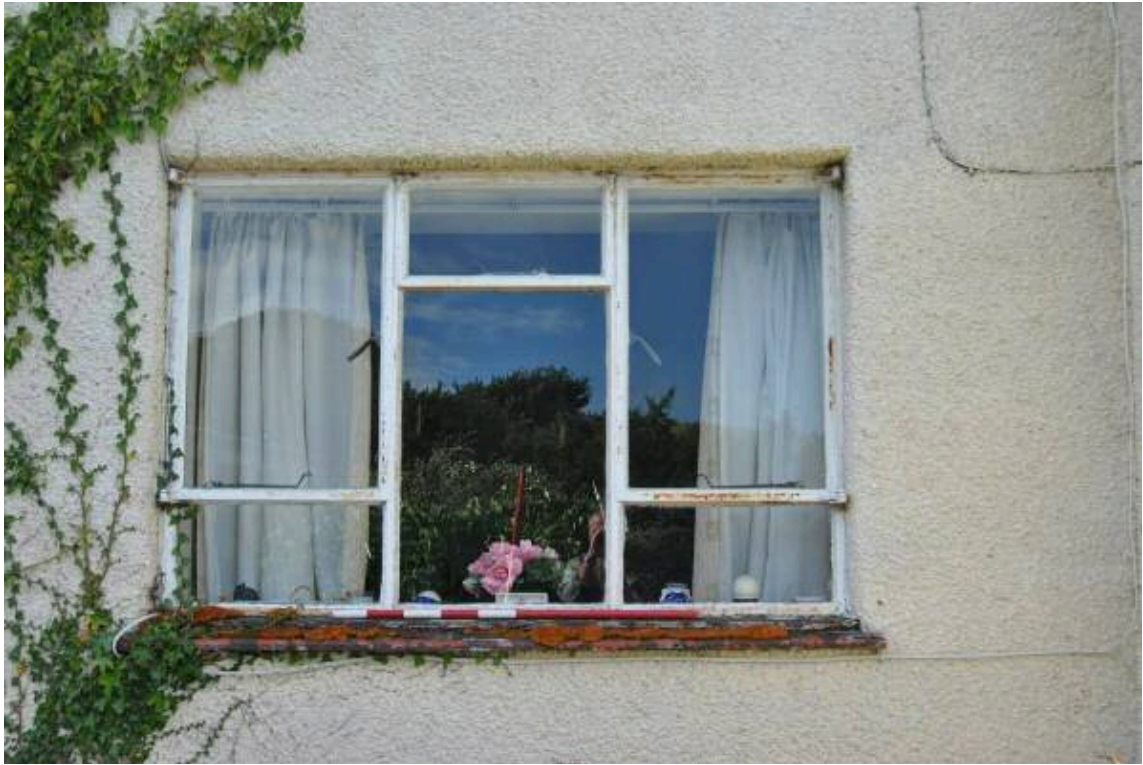
Plate 3: Unsympathetic steel-framed windows, introduced throughout in late 1950s.
