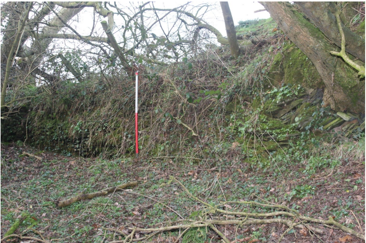
Photo 26: Facing northwest. Wall retaining the outside of the bank on the west side of Castell Pen-yr-Allt, with a 1m scale.
