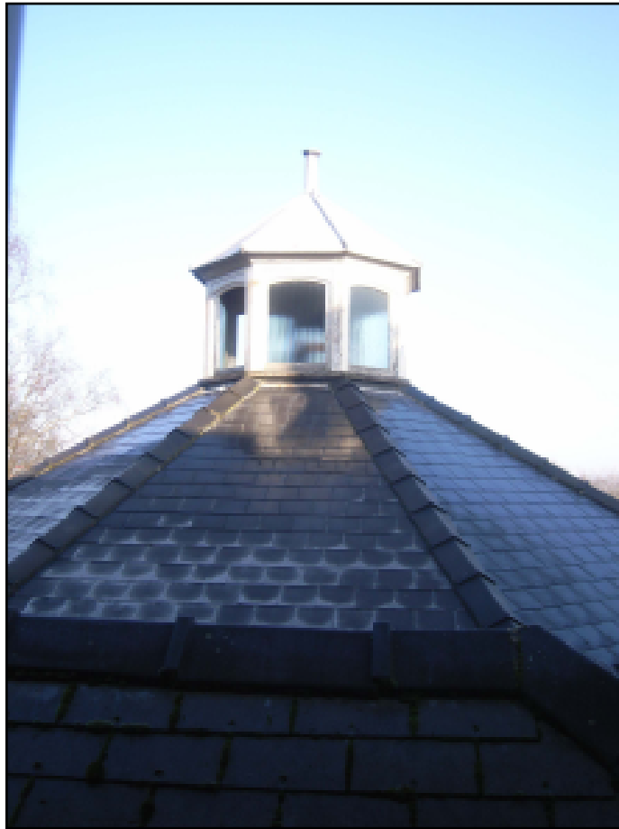
Plate 5 Lantern atop conical roof of the octagonal courthouse to rear of Shire Hall. View to north
