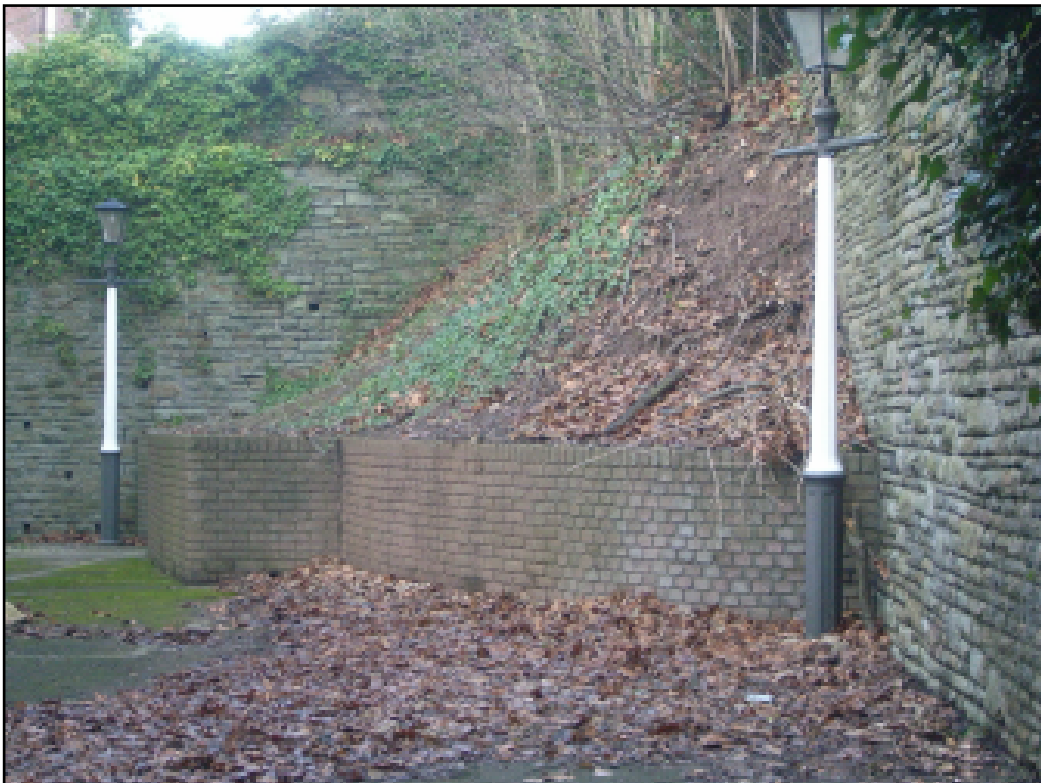
Plate 6 Two original gas lampstandards made of cast iron, in yard to rear of Shire Hall. A third one stands behind the photographer. View to west
