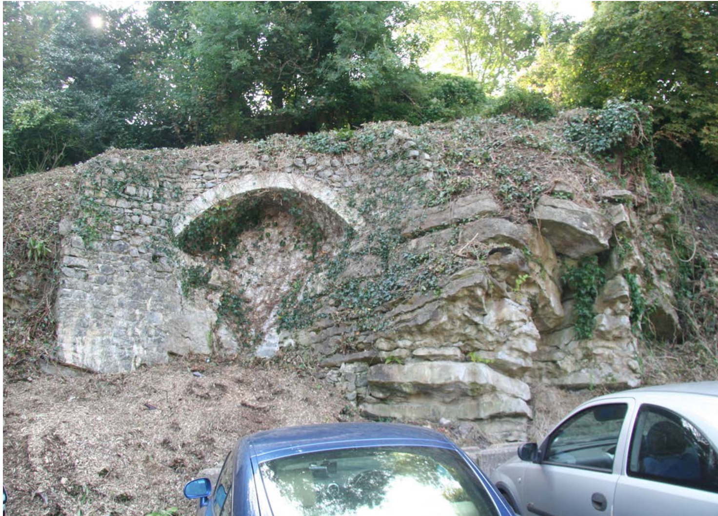
View of section of stone wall and arch on the eastern edge of the rear external car park (looking east)
